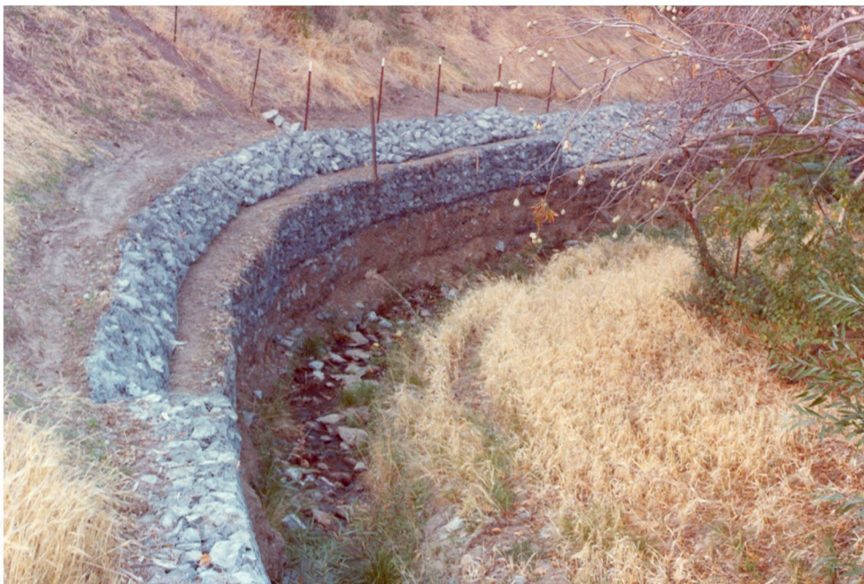
Figure 20. A, Schematic section view of gabion-faced Geogrid embankments constructed as part of a bank repair along Alhambra Creek in Martinez, California. The use of soil backfill lessened off-haul costs for excavation and negated two-thirds of the required rock fill import necessary to fill a conventional all-gabion retention structure. B, Photograph of the completed channel repair, looking downstream. Wall height is 9 to 12 ft (~2.7–3.6 m) with a 6-ft-deep (~1.8 m) footing to protect against undercutting.
