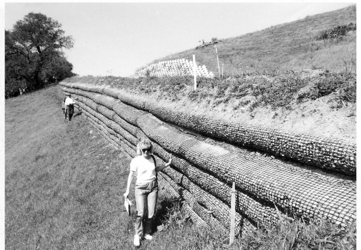
Figure 15. A, As-built view of a Geogrid gravity retention structure constructed using native gravelly colluvium. Total wall height is ~10 ft (~3 m) with a grip distance of 10 ft. B, As-built view of a vertical Geogrid retention structure constructed on a 20% grade to support a roadway crossing of a colluvial-filled swale. Tensar SS-2 geogrid was utilized with crushed gravel at the outside face to act as a protection against fire, rodent activity, and to provide a reaction surface for compaction near the exposed face.
