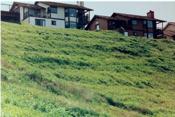
Figure 14. Two views of a Geogrid-reinforced landslide repair accomplished on an emergency basis between October and December 1986 in Crockett, California. The lower view shows the finished slope six weeks after completion in late January 1987. The slope had been hydroseeded and Geogrid face wrap acts as an excellent mulch mat.
