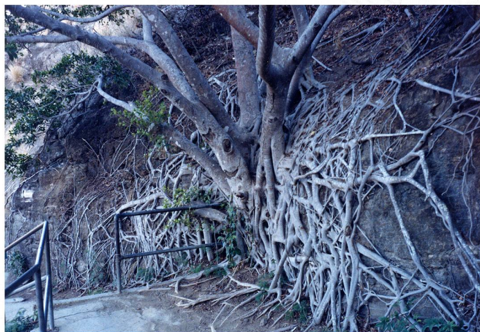
Figure 10. Nature's concept of soil reinforcement is shown to good effect in the root network of a banyan tree, here stabilizing a nearly vertical cut in colluvium on a National Park Service trail at Diamond Head, Oahu, Hawaii. Water percolating through the colluvium serves to propagate the expanding root system. The new technologies of micropiles, soil nailing, fiber-reinforced soil, and bioengineering emanate from this natural example. In terms of frictional contact area, such tropical trees are easily capable of engendering 10,000 psf increased shear strength to the soil.
