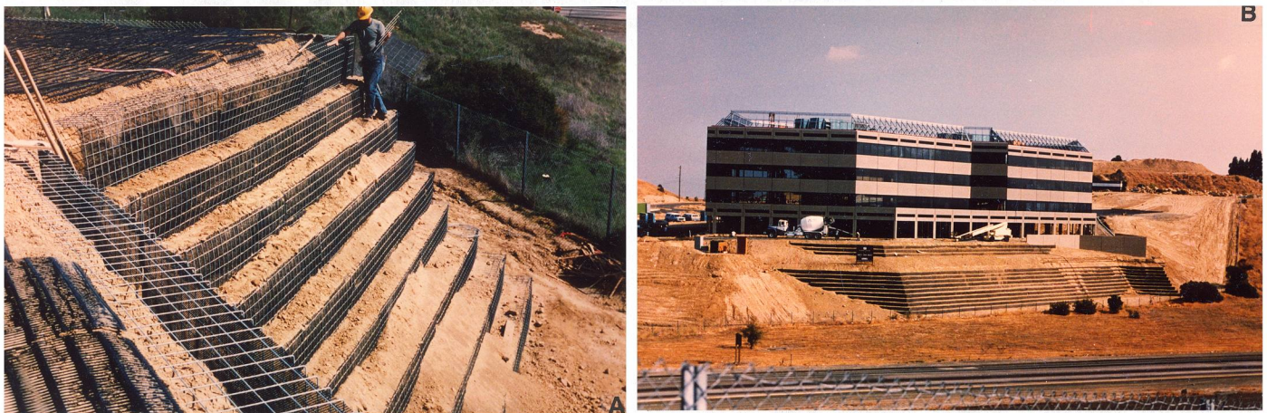
Figure 23. A, Construction view showing emplacement of welded wire mesh facing elements being used with Geogrid soil reinforcement to construct a 0.5:1 embankment slope below a proposed office complex. Welded wire mesh retention systems have been promoted for some years by Hilfiker Corporation in California and Pacific Wire in Tacoma, Washington. Such systems are employed by the same theories applicable to Geogrids and geomembranes. However, Geogrids can be less expensive to purchase and place because they do not require extensive tying. B, As-built view of the completed embankment of 11,000 yd 3 (~8360 m 3 ) beneath the Crest Office Park complex, Martinez, California.
