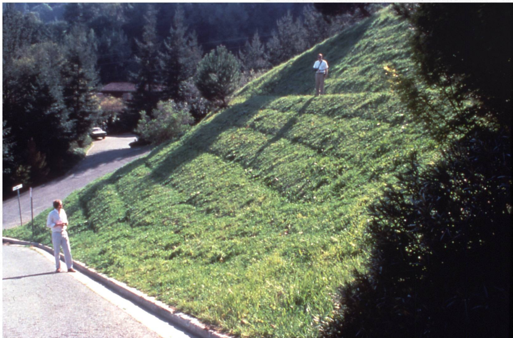
Figure 16. A, Typical face wrap detail on a Geogrid reinforced embankment steeper than 1:1. The grid provides an excellent mulch for hydroseeding, much like jute mesh. B, As-built view of a face-wrapped Geogrid repair on a 60-ft-high (~18 m) cut slope failure that involved bedrock exposed in an old 1:1 road cut. The repair of such steep slopes cannot be accomplished with traditional methods of removal and recompaction. Note excellent cover of hydroseeded grass.
