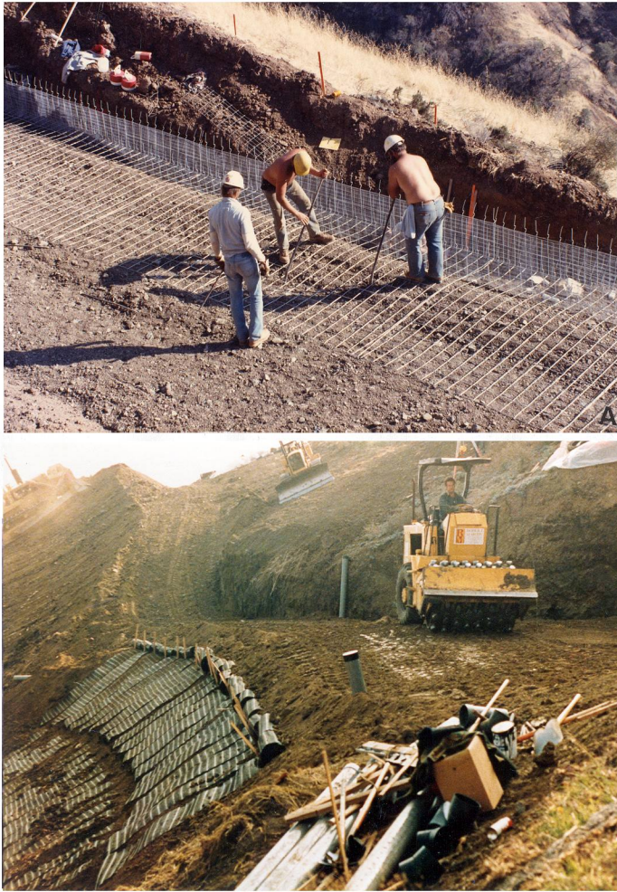
Figure 12. A, Placement of welded wire mesh soil reinforcement near the face of a vertical embankment structure during construction. Soil is then spread over the mesh and compacted in 6–8-in-thick (~15–20 cm) lifts. The area immediately adjacent to the free face usually requires local compaction with hand-operated vibratory equipment. B, Compaction of fill lifts in a landslide repair between successive layers of Tensar Geogrid with face warps at 4 ft (1.2 m) intervals. The slope face was repaired at a slope of 1.7:1 directly beneath a series of existing structures.
