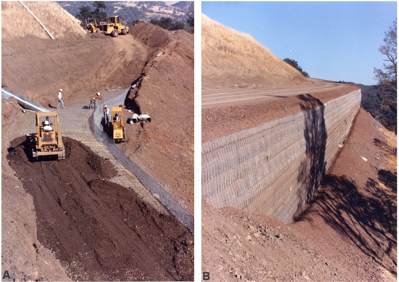
Figure 22. A, Earthen lift being spread over welded wire mesh. In lifts about 2 ft (~0.6 m) high, a mechanically stabilized highway embankment with vertical face was constructed across an active landslide area. B, As-built view of a welded wire mesh embankment constructed parallel to the road's 10% grade. The face may deform outward as the fill consolidated with time, especially when wetted.
