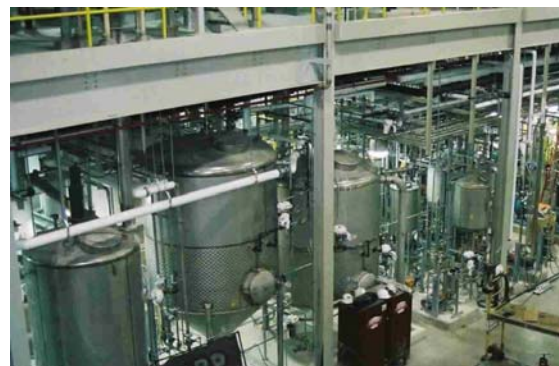
Fermentation tanks and separation equipment
