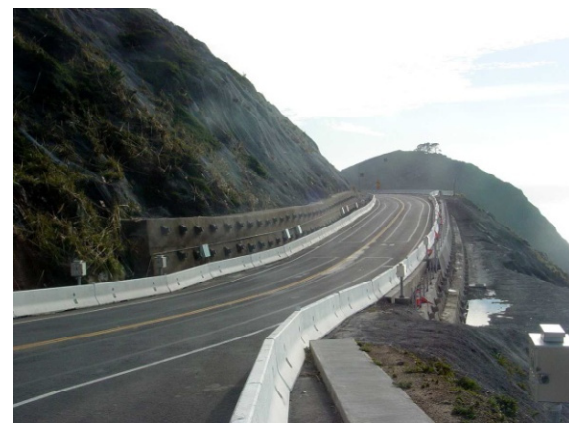
Challenge for GE students: Build a pipeline thru this? GE Senior design class, California.
