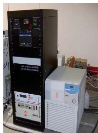
1 – Chiller, 2 – High Voltage Supply, 3 – RF Supply, 4 – Gas Pressure Figure 2. Power Control Systems. 1
