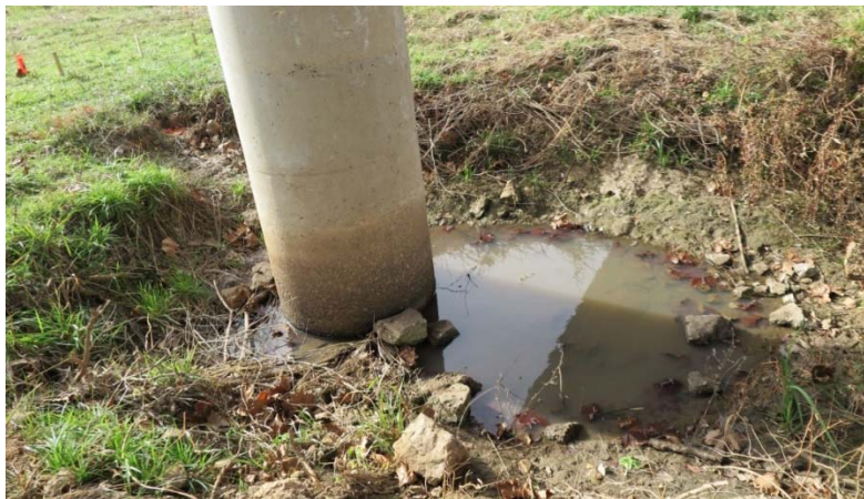
Figure 2 The Bridge Pier with a Scour Hole
