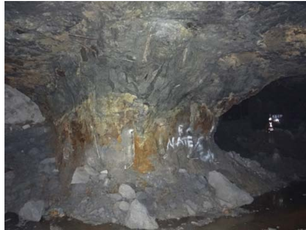
Figure 13: Spalling pillar in Doe Run's Buick Mine.
