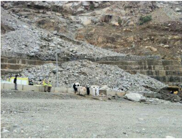
Fig. 4 Debris flow along site 1 in Al-Hada highway and the existing bulkhead type barriers
