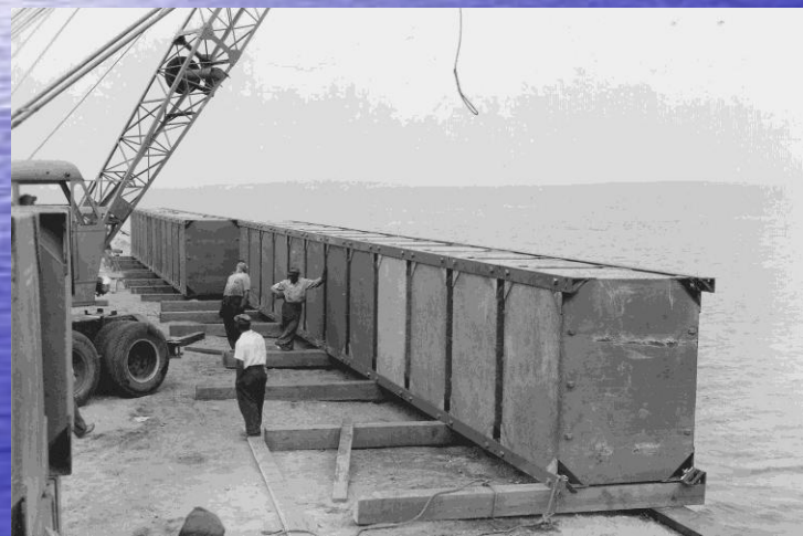
"Pontoon strings" were fabricated by employing steel angle stiffeners along each corner.
