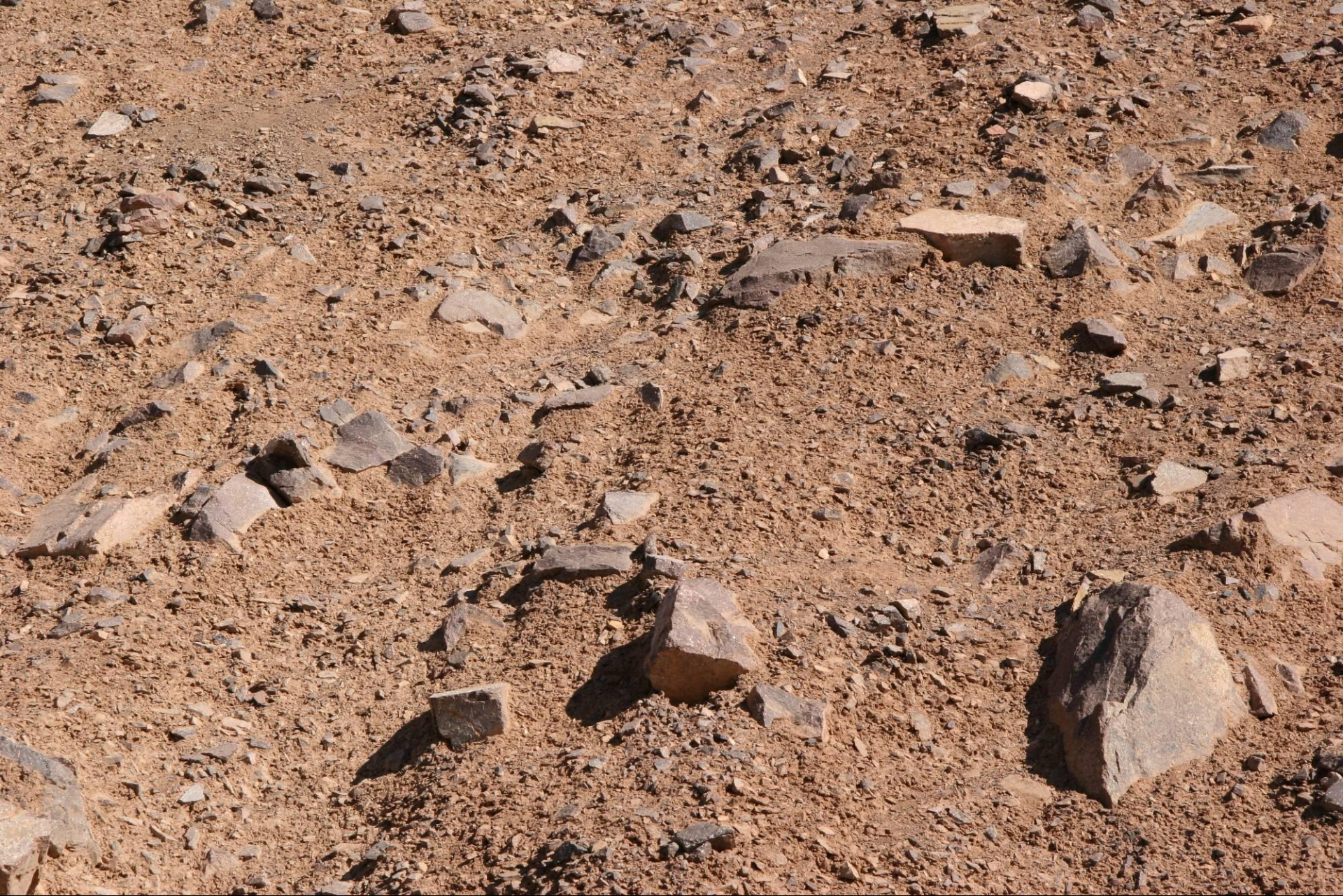
Close up of “dirty” rockfill exposed at failure site. For scale, the large rocks are 10-12” in diameter.
