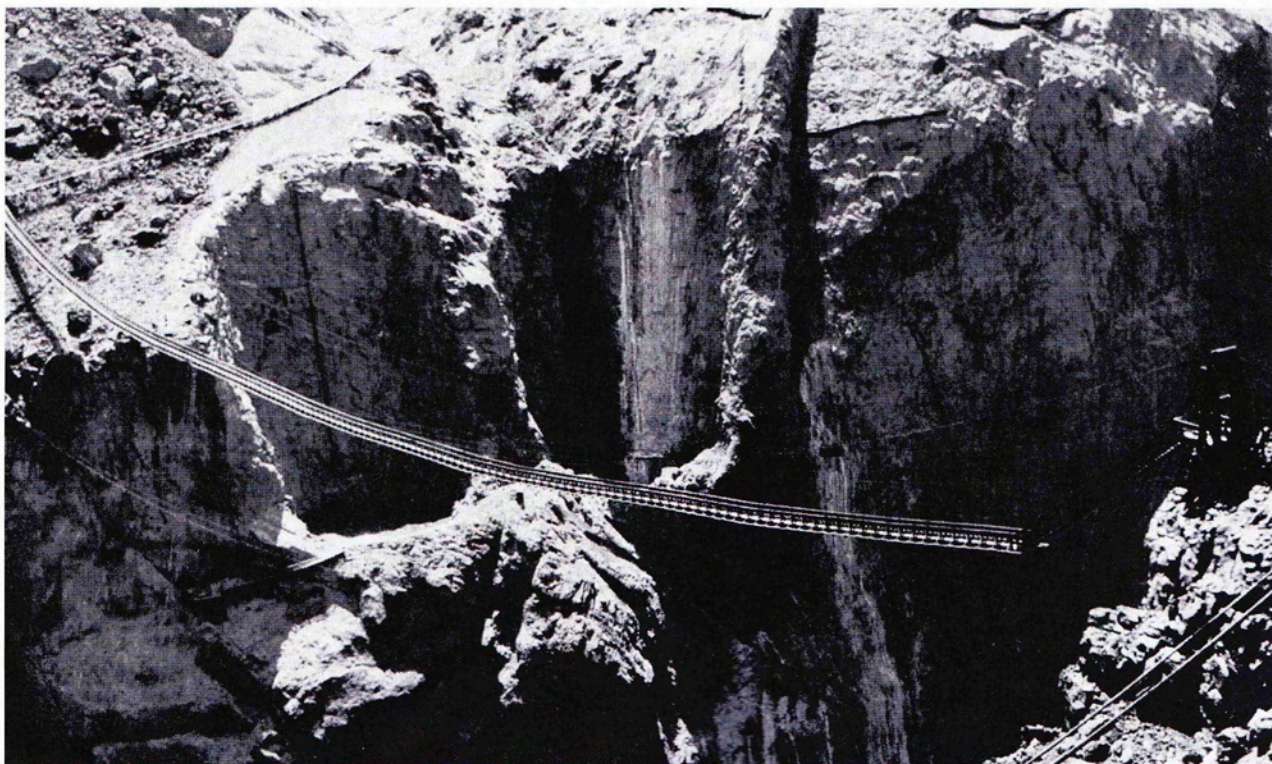
A daring catwalk suspension bridge was situated 650 ft above the river to enable workers to cross from the Nevada side to work on the Arizona spillway.
