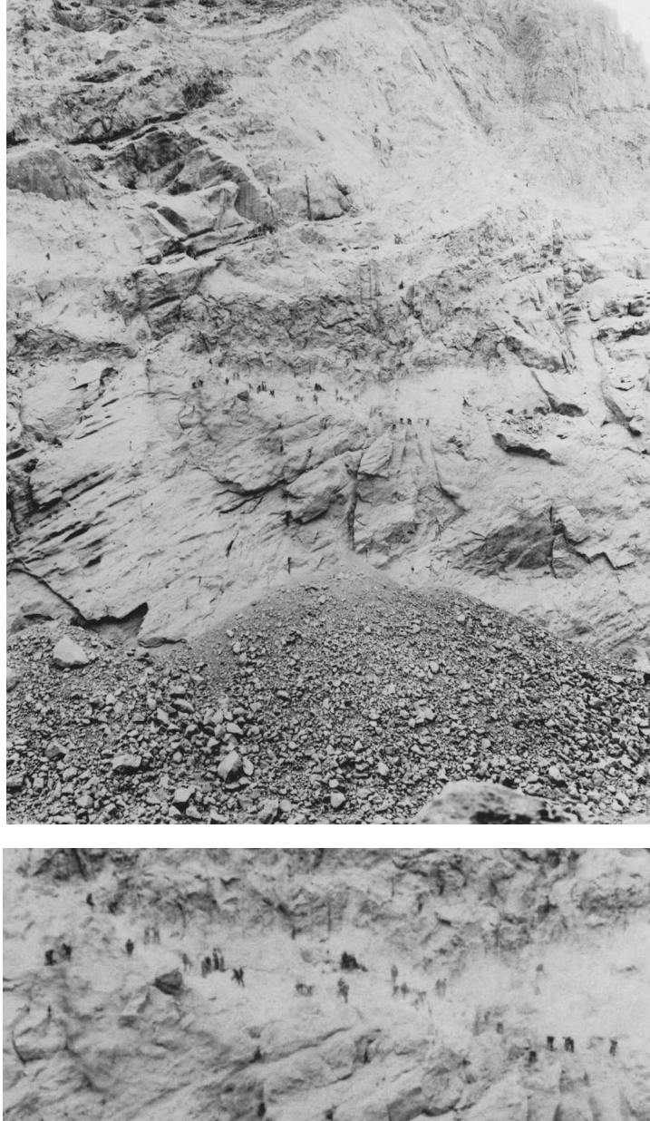
FIG. 15. Upper: High scalers working the lower portion of the dam's left abutment, on the Arizona side. Note the raw loose character of the freshly blasted rock and the sheer scale of the operation. Lower: Enlargement of the same image, showing the high scalers worked line abreast of one another (USBR).
