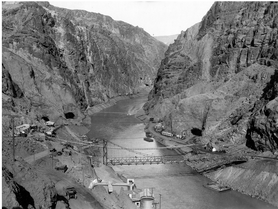
FIG. 9. Suspension bridges, roads, and rail spurs accessed the diversion tunnels and dam site at river level. Tunnel muck on the Nevada side was removed by rail while that from the Arizona tunnels was removed by truck. The Arizona tunnels were completed first and lined in late October 1932 (USBR).
