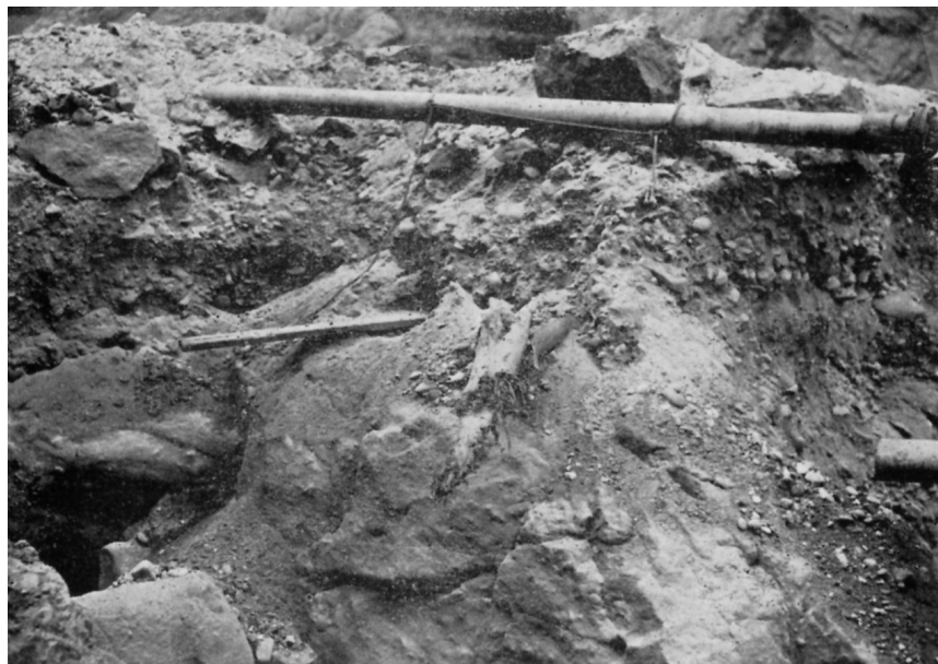
FIG. 19. Upper image shows excavation of the cobbles, boulders, sand, and gravels of the Colorado River on April 3, 1933 when crews began excavating the “inner gorge,” which extended much deeper into the andesite bedrock. This narrow trough was filled with boulders up to 12 feet in diameter. Lower image shows the 2 x 6 inch plank unearthed at a depth of 50 feet below the river bed, thought to have been deposited during the peak flows of June 1921, which reached 170,000 cfs (from USBR, 1950).
