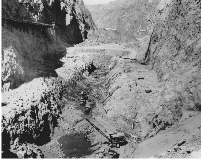
FIG. 20. View of the excavated ‘inner gorge’ of Black Canyon as it appeared on June 3, 1933. This inner gorge was filled with enormous subangular boulders, which had fooled drillers in thinking they had encountered ‘bedrock’ during the first two seasons of drilling, in 1922-23 (USBR).
