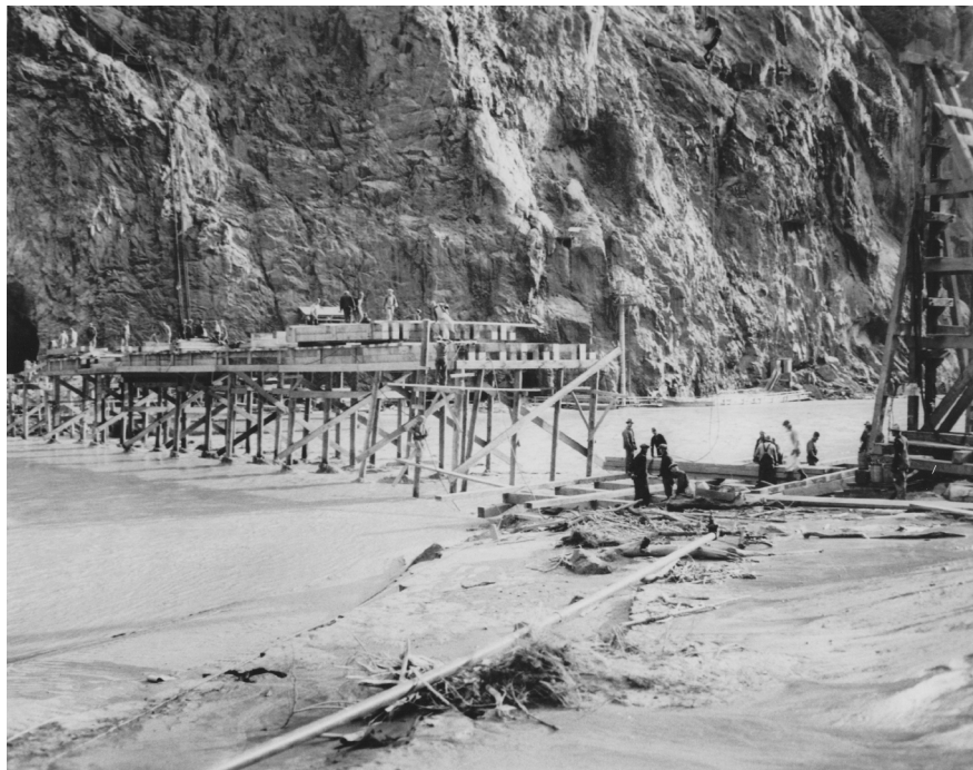
FIG. 5. Six Companies employed a variety of bridges to get workers and equipment across the channel. They began by driving timber piles to fashion simple timber trestle bridges such as that shown here, which replaced the span lost in the high water of February 10, 1932 (USBR).
