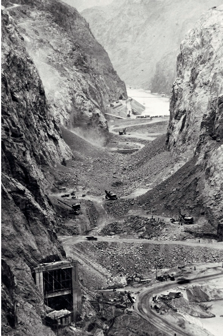
FIG. 18. View looking upstream from the Nevada abutment at the excavation work in December 1932 as the abutments were being trimmed back. The downstream cofferdam is taking shape in the foreground. The cofferdams had to be completed before they could begin excavating the channel gravels. All of the excavated materials had to be transported to disposal sites in steep side canyons upstream or downstream of the dam (USBR).
