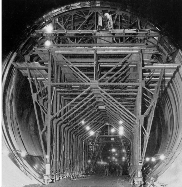
FIG. 12. Traveling slip-form used to line the crown of the diversion tunnels after pouring the invert and filling it with 15 feet of gravel, to serve as a road bed. This was the largest traveling slip form ever fabricated at the time (USBR).
