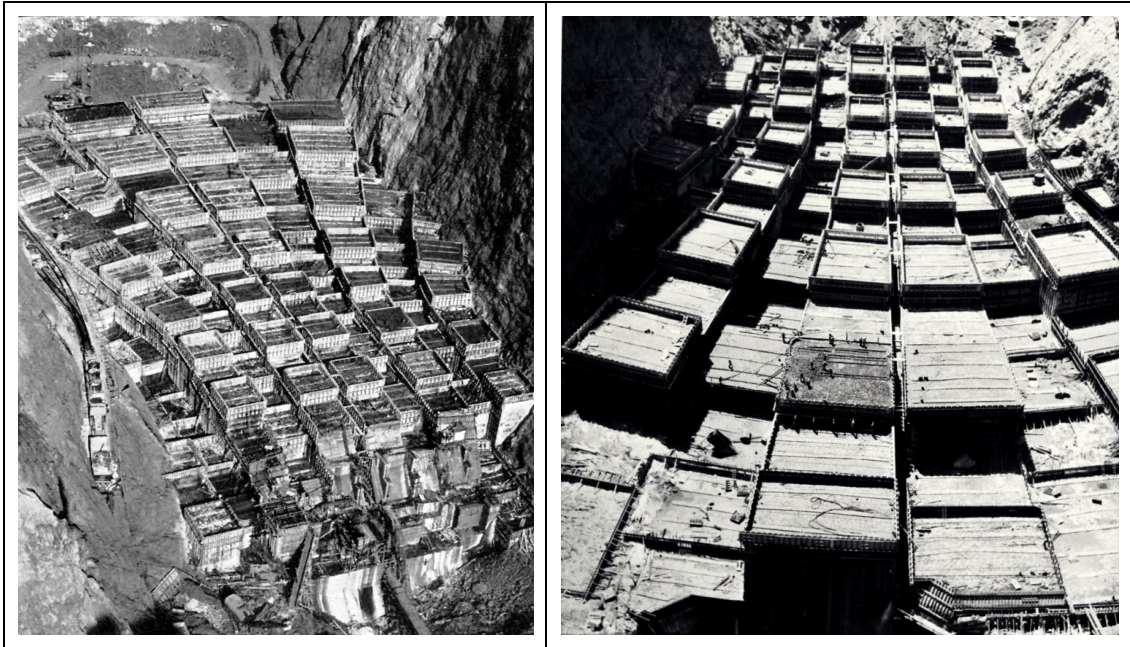
FIG. 29. Interlocking and convergent nature of the dam's basal blocks can be appreciated in these views, taken during construction. Left view looking upstream, while that at right looks downstream. The blocks were poured intermittently to enhance heat dissipation into the air immediately after placement, caused by the concrete's heat of hydration (USBR).
