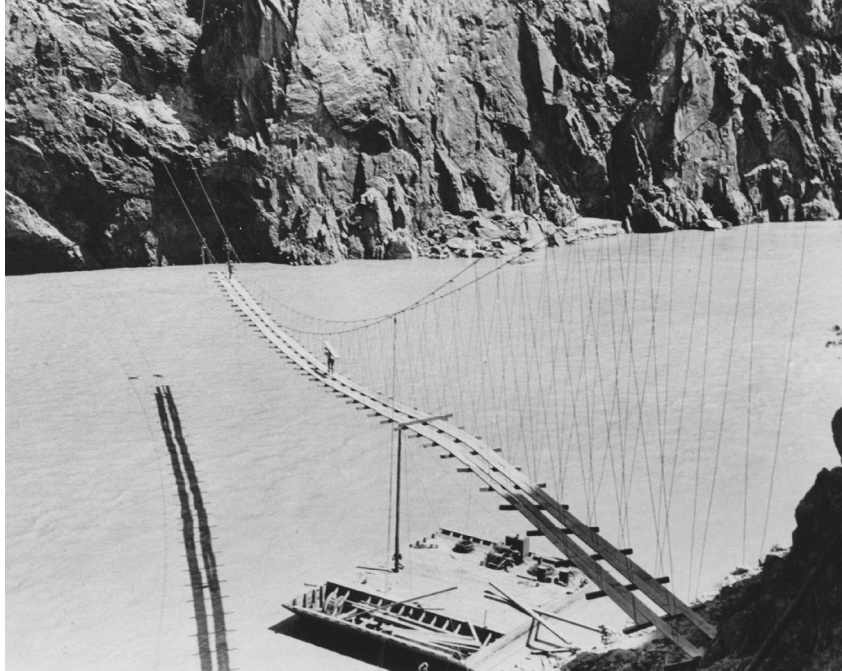
FIG. 4. Six Companies quickly built a series of suspended walkways like that shown here under construction to access the Arizona side of the river, to begin excavation of the two diversion tunnels underlying the dam's left abutment (USBR).
