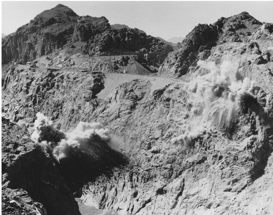
FIG. 14. Noontime production blasts on the Arizona abutment upstream of the dam. Tourists flocked to view the small blasts that accompanied the lunchtime breaks, when workers were cleared from the canyon floor.
