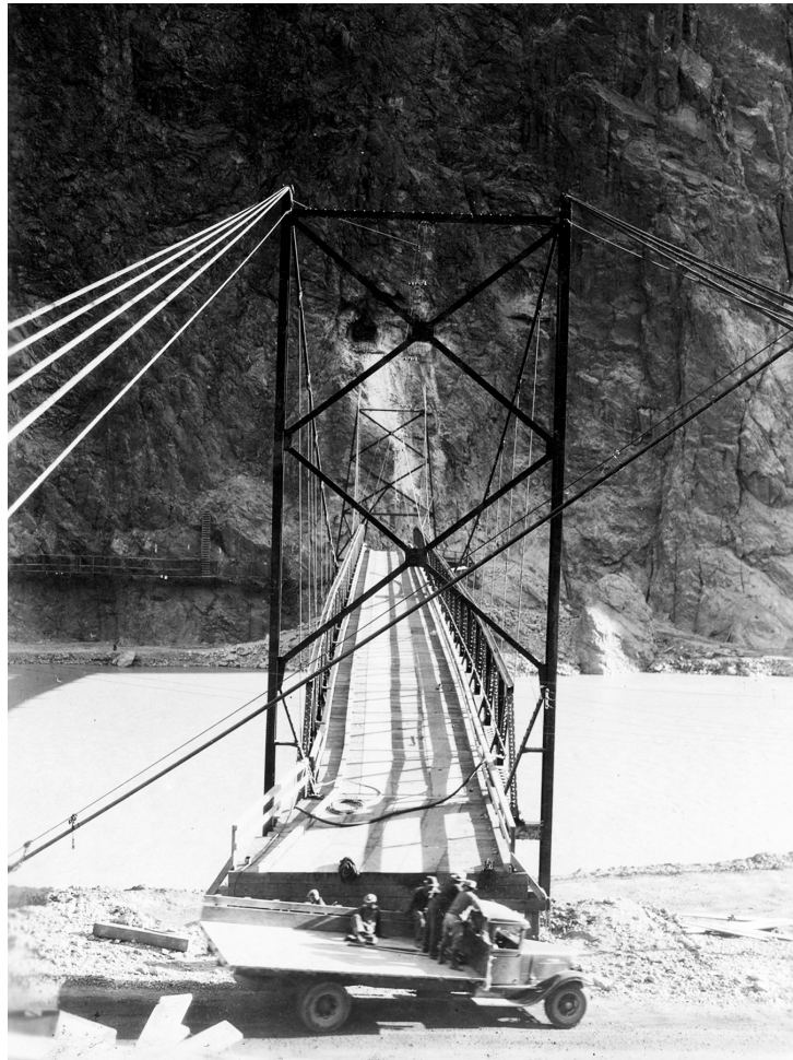
FIG. 7. Suspension bridge built by Six Companies just downstream of the dam site to allow access to 8 x 10 ft cross adits so they could drive multiple headings on the massive diversion tunnels. The portal on the Arizona side is clearly seen, about 50 feet above the bridge deck on the far side. Six Companies was not paid for constructing these additional tunnels, which greatly hastened the construction schedule (USBR).
