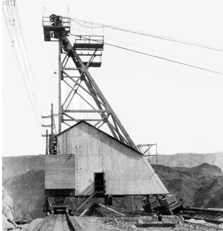
FIG. 2. One of the 20-ton cableway towers mounted on rails, which allowed it and another similarly configured unit on the opposite canyon wall, to be moved 500 ft up or down the canyon, to facilitate precise placement of the 8-cubic-yard concrete buckets (USBR).
