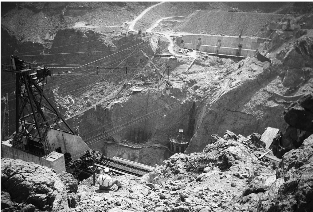
FIG. 50. Intricate network of overhead cableways and suspended catwalks just upstream of the dam. These were used to carry workers and convey buckets of concrete to the spillways and intake towers. High strength structural concrete was used on the intake towers (Preston Collection Boulder City Library).
