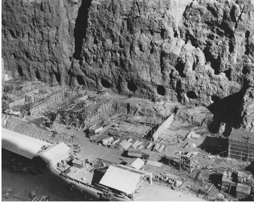
FIG. 22. Oblique view of the eight 21-foot finished diameter penstock feeder tunnels connecting to the Arizona power house, under construction. The steel penstocks are 11 feet in diameter (USBR).
