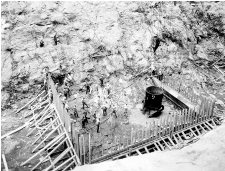
FIG. 6. Placing the first 8-cubic-yard bucket of concrete on the scrubbed bedrock surface of the inner channel on June 6, 1933. Note batter boards supporting forms. (USBR)
