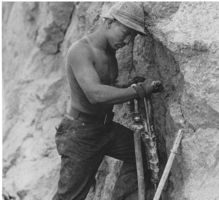
FIG. 33. One of the high scalers at Hoover Dam wearing a home-made ‘hard-boiled hat’ fashioned by overlapping two baseball caps and dipping them in tar and chilling or brushing leather hats with shellac (USBR).
