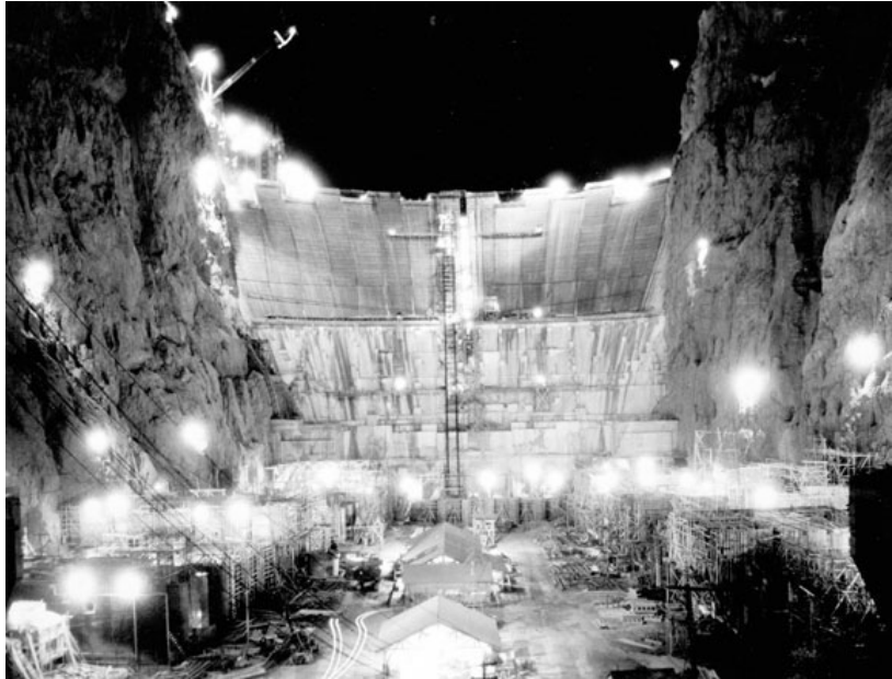
FIG. 11. Concrete placement was carried out around-the-clock, and the night shifts were a welcome respite during the summer. This time exposure shows the formwork for the powerhouses in the foreground with the dam in the background (USBR).
