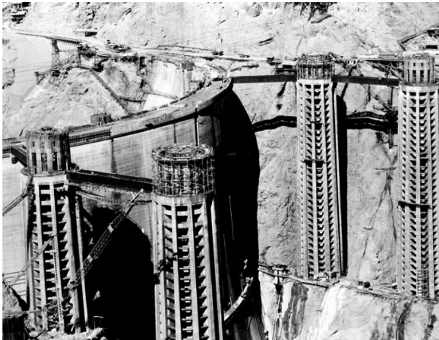
FIG. 18. Overview of the four intake towers approaching completion, as seen on March 26, 1935. The towers rise above the dam crest and are just under 400 ft high (USBR).
