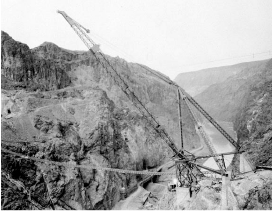
FIG. 17. Stiff-leg derricks were also erected on the Arizona abutment to place concrete to the Arizona intake towers. Taken on December 27, 1933 (USBR).
