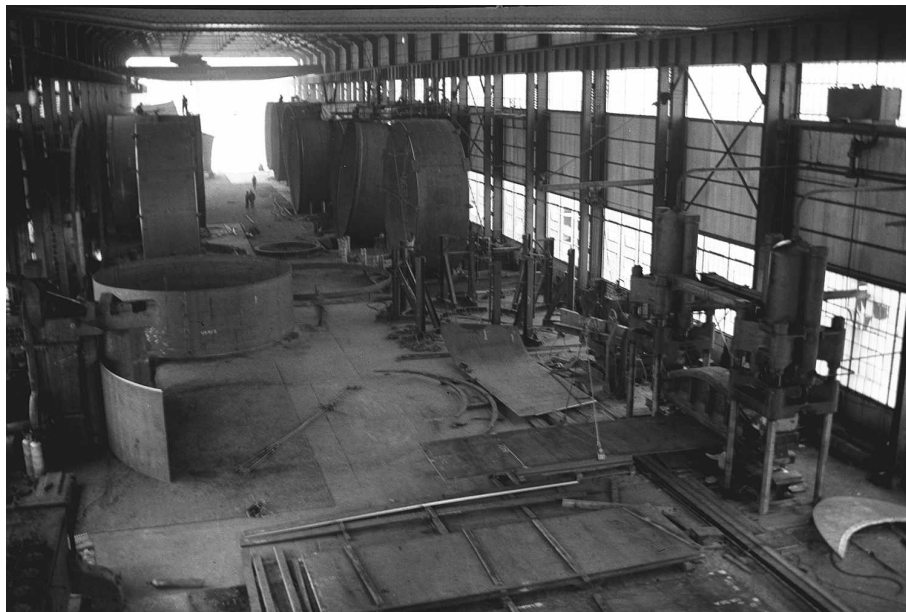
FIG. 26. 11-foot-long sections of the 37-foot-diameter penstocks being bent and conjoined by arc-welding inside the Babcock & Wilcox Steel Fabrication Plant (Preston Collection-Boulder City Library).
