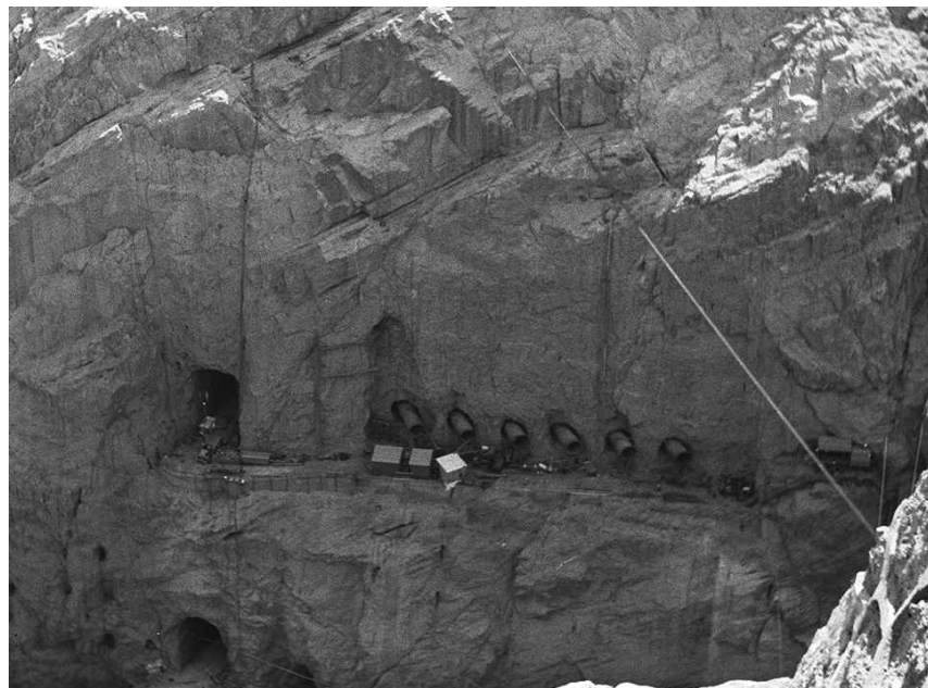
FIG. 23. Oblique view of the canyon wall valve house outlet works tunnels. The conduits were 7 ft in diameter and the tunnels 11 ft in diameter with a horseshoe shape. These tunnels were lined after the 102-inch-diameter outlet pipes were placed (Preston Collection-Boulder City Library).
