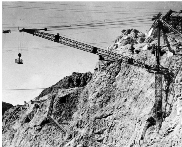
FIG. 5. Another 20-ton capacity stiff-leg derrick in its precarious perch on the dam's right abutment to continue handling of concrete buckets coming from the Low-Level Mixing Plant after the dam rose 150 ft above the river bed. (USBR)
