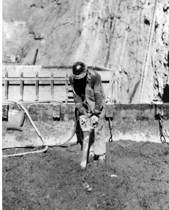
FIG. 9. Workman using pneumatically powered concrete vibrator to remove some of the entrained air from wet concrete in one of the dam's blocks (USBR).
