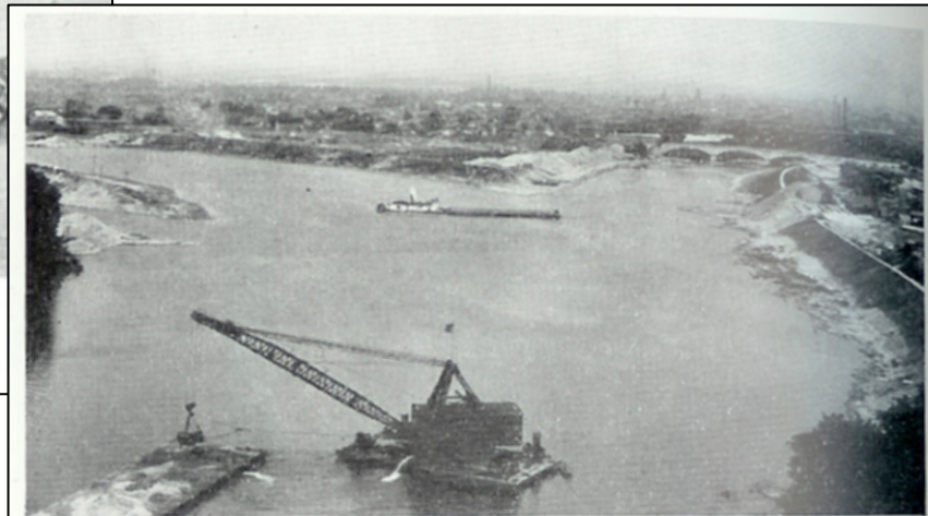
Dragline at Dayton. Mounted on a barge in the Miami River, the dragline loads another barge with material excavated from the channel. In the distance the steam tug "Dorothy Jean" is moving a loaded barge to be unloaded at the spoil bank or for building a levee.
