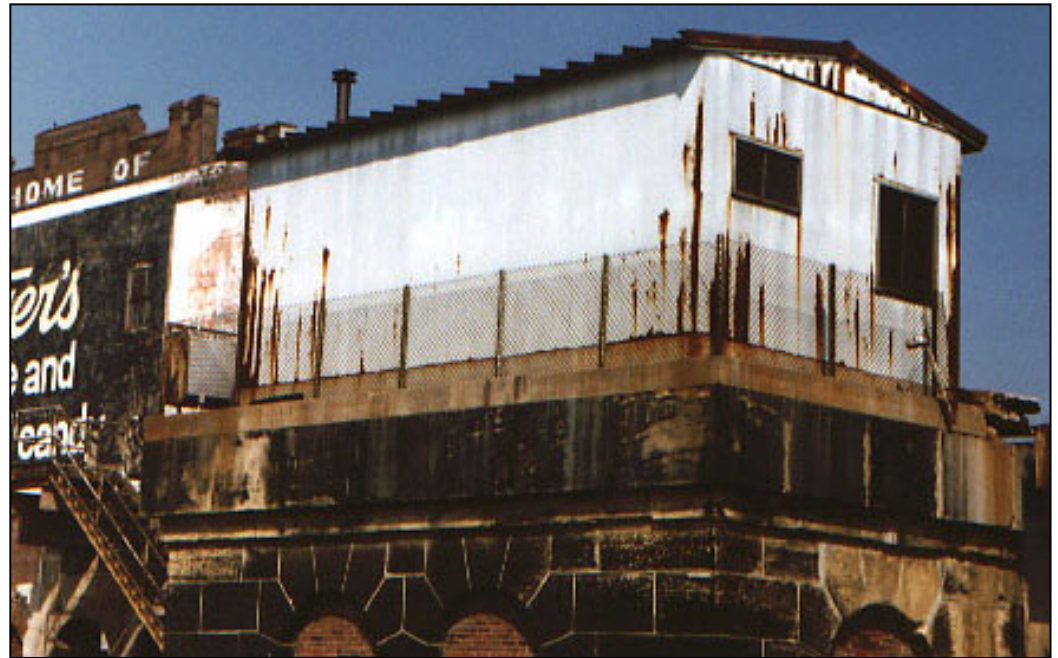
Rusting Toll Booth
