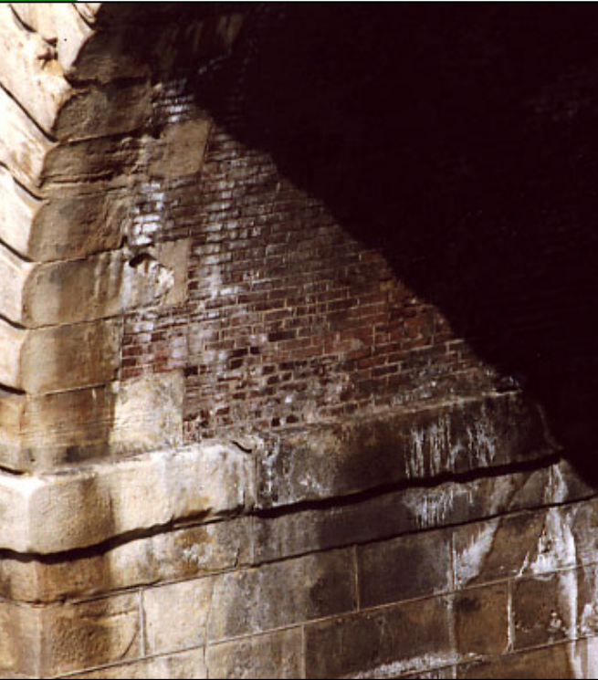
Deterioration of Abutment Masonry
