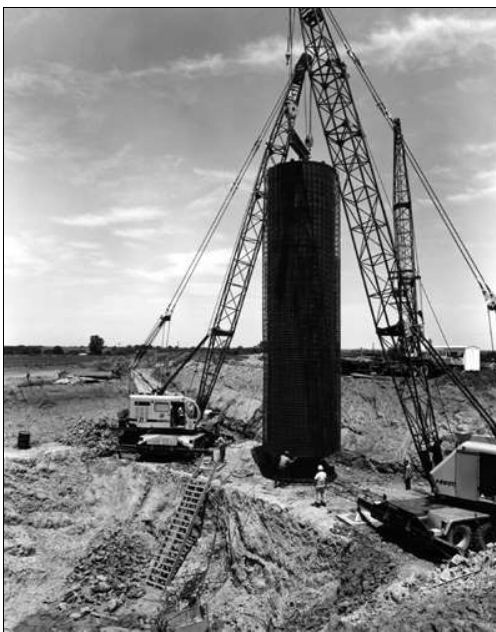
Construction of Minuteman Launch Silo B-11 at Whiteman AFB, MO on June 18, 1962
