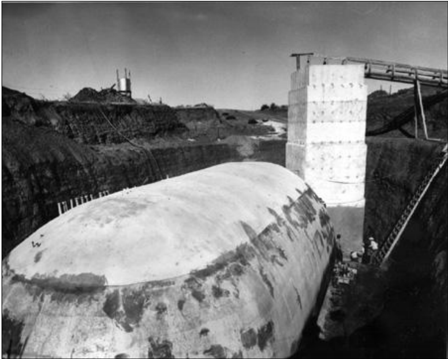
Close up of Launch Control Capsule under construction at Ellsworth AFB, SD in Sept.1962
