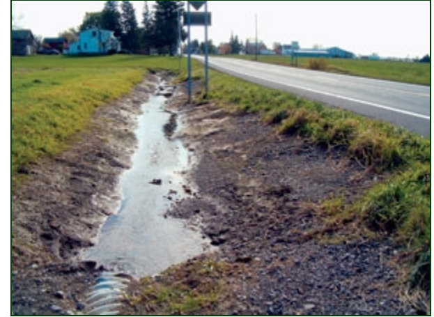
Unlined ditches often degrade, clogging culverts
