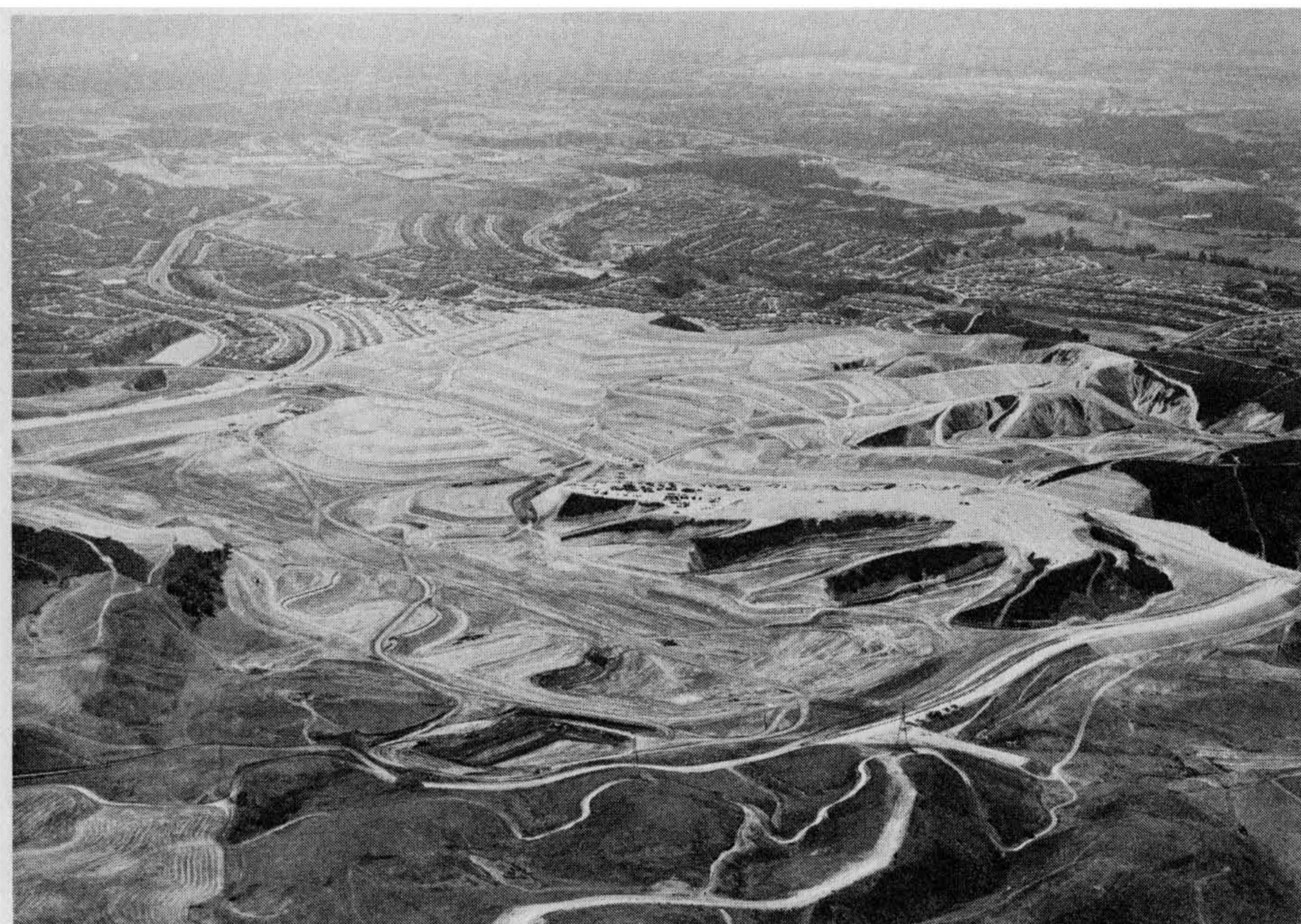
Figure 2.8 The Lake Mission Viejo grading completed as shown on September 1, 1976. The future Mallorca condominium site, in center with equipment, has been graded. Photograph by Aerial Eye Inc., courtesy of the Mission Viejo Company.
