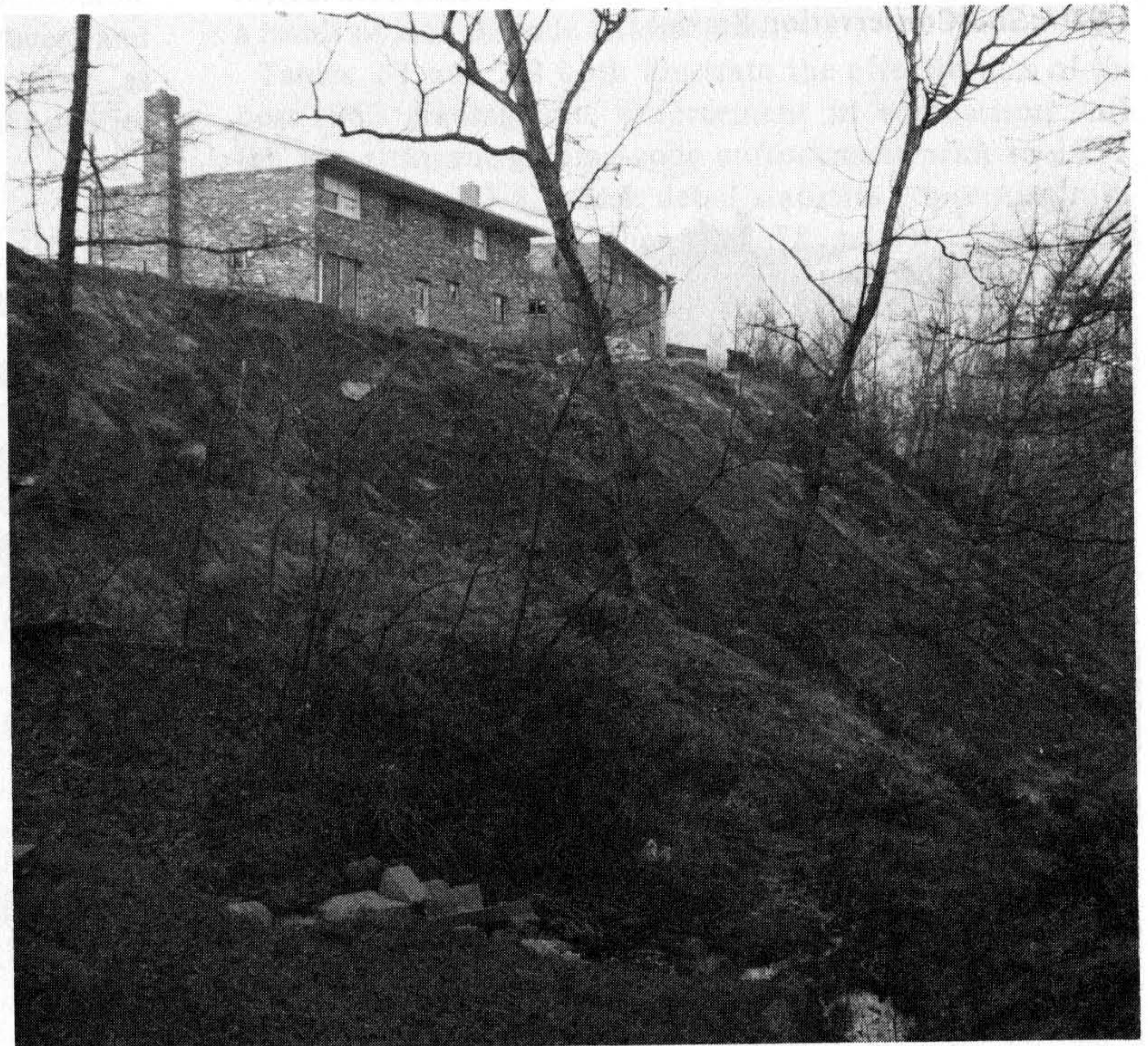
Figure 2.11 Uncompacted loose fill shown drifted over the slope at rear of residences in Silver Springs, Maryland. These houses have failed structurally due to differential settlement. Occupancy permits have been denied. (Montgomery Soil Conservation District. Photography by J. F. Hazen, courtesy of USDA-Soil Conservation Service (Montgomery Soil Conservation District.)
