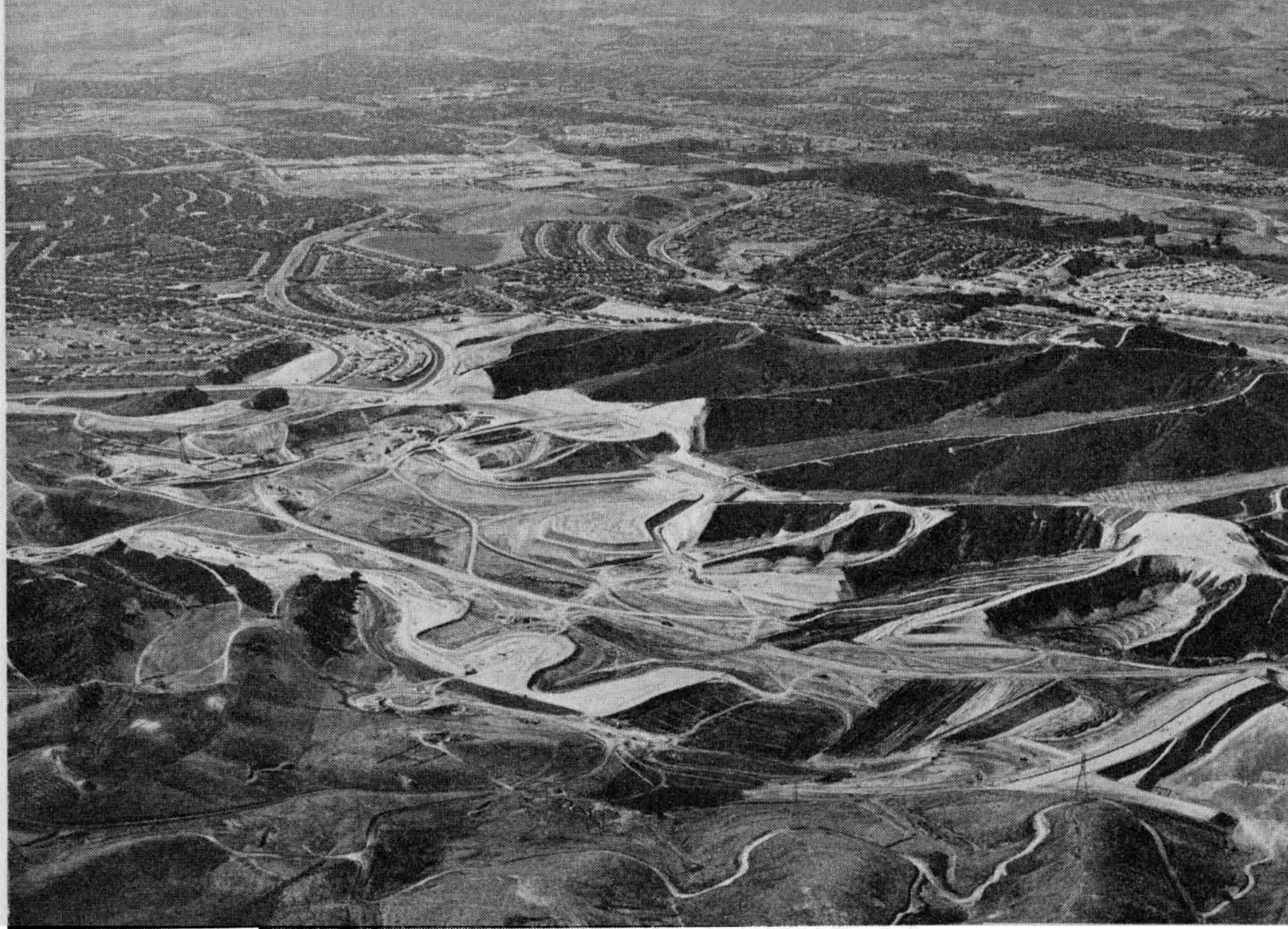
Figure 2.7 Lake Mission Viejo grading construction in progress on November 12, 1975. Note the extensive canyon clean-out and compressible soil removal. The slurry trench is being excavated in the left center. Photograph by and courtesy of the Mission Viejo Company.
