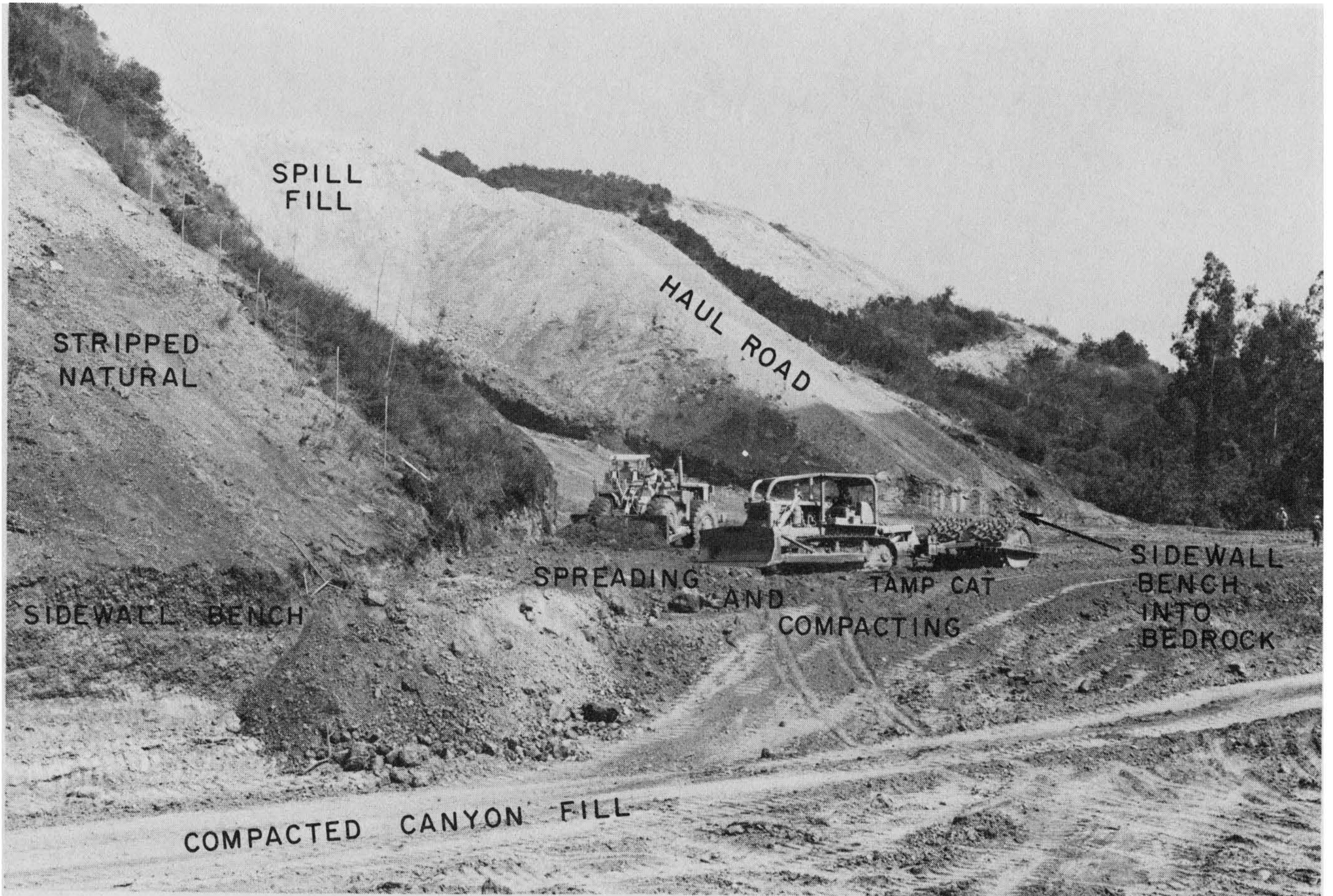
Figure 5-17 Canyon filling-in progress. The sidewall benches are narrowing as fill is almost lapping onto the near surface soils. The slope on the left needs to be rebenched. Notice the spill fills adjacent to the haul roads. These loose fills were inadvertently spilled during hauling and must be removed prior to fill placement. Photograph courtesy of the Dept. of Building & Safety, staff photographer John Shadle.
