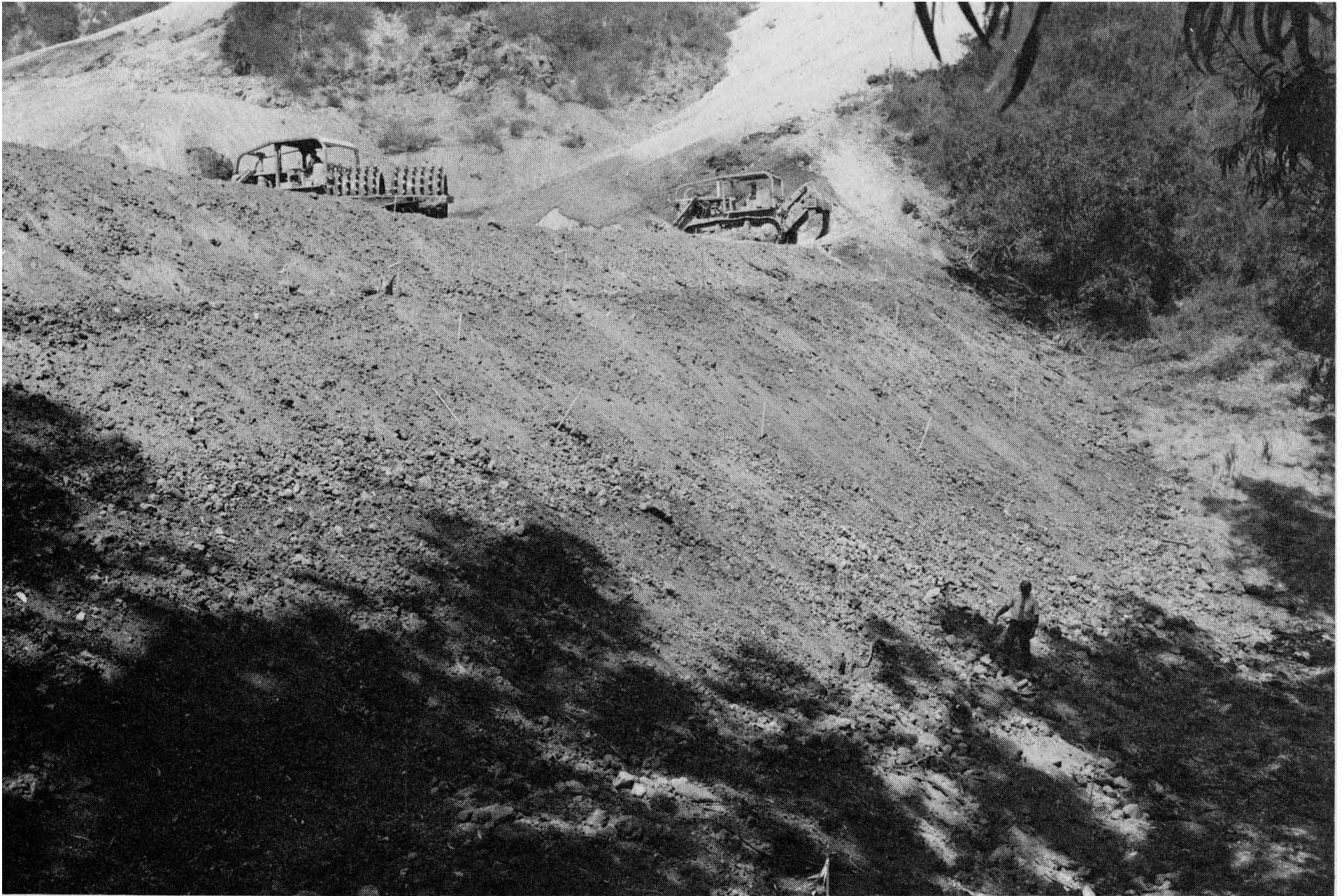
Figure 5-36 Canyon-fill slope construction in progress. This fill appears to be 8-10 ft. above the lowest terrace drain. Loose spill fill overlays the surface and must be removed or compacted during finish grading. The inspector is walking along the toe-of-fill slope. Photograph courtesy of the Dept. of Building & Safety, City of Los Angeles, staff photographer John Shadle.
