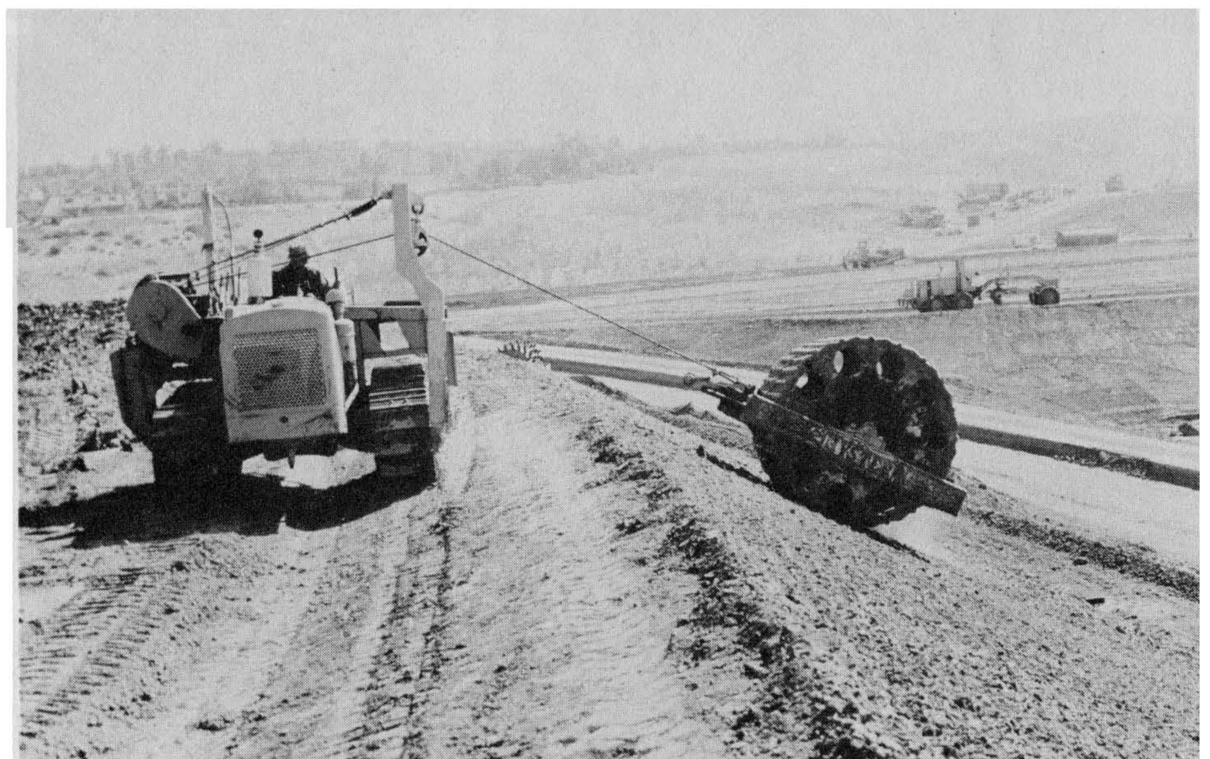
Figure 5-41 Notice the wide berm at the top of this fill slope. A wide berm is constructed to prevent drainage from going over the slope and to channel drainage away from the slope. Photograph by C. Michael Scullin.
