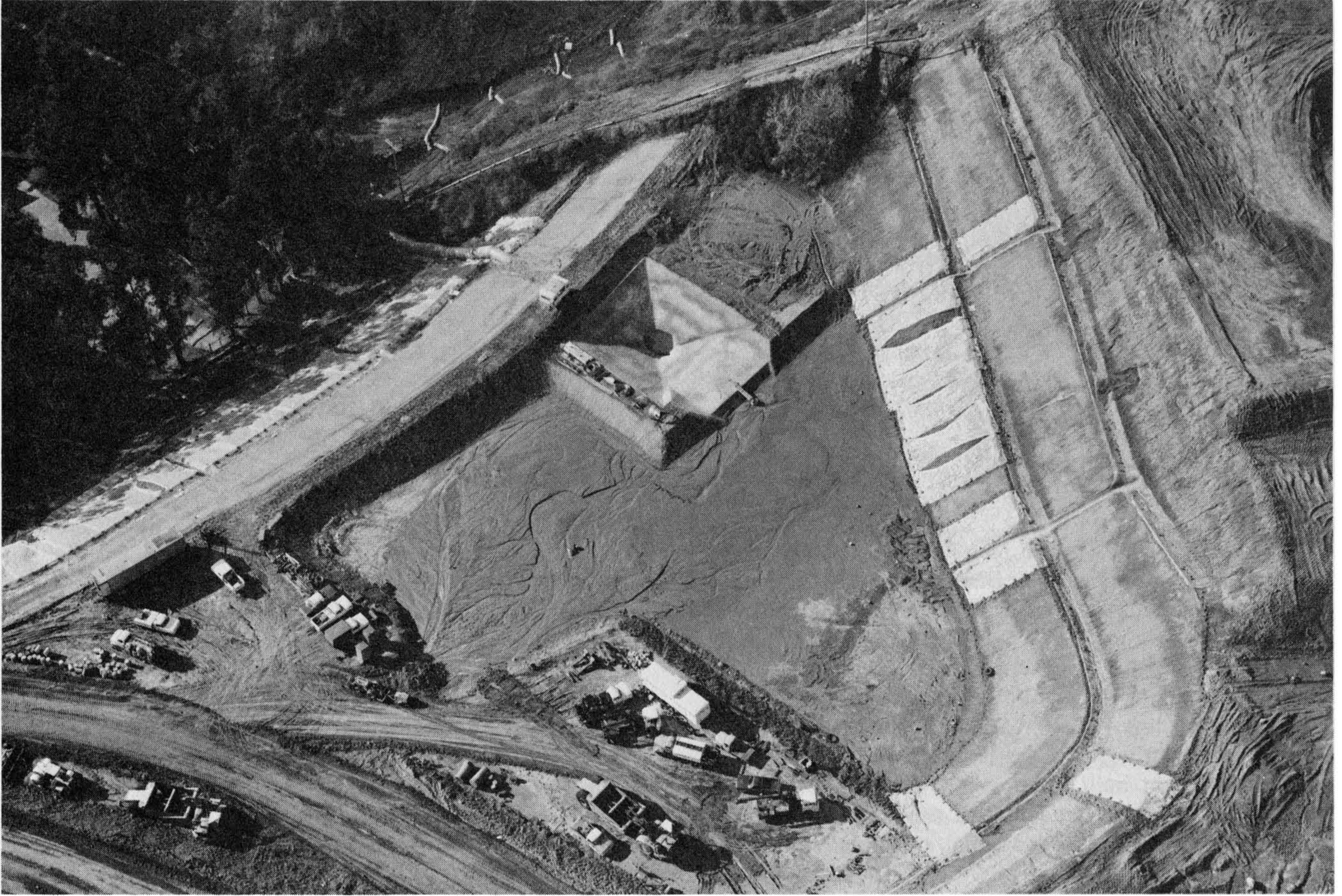
Figure 5-61 This large desilting basin at low end of tract will collect silt runoff and protect adjacent property down slope during rough grading and before street and storm drain construction. Photograph courtesy of the Dept. of Building & Safety, City of Los Angeles, staff photographer John Shadle.
