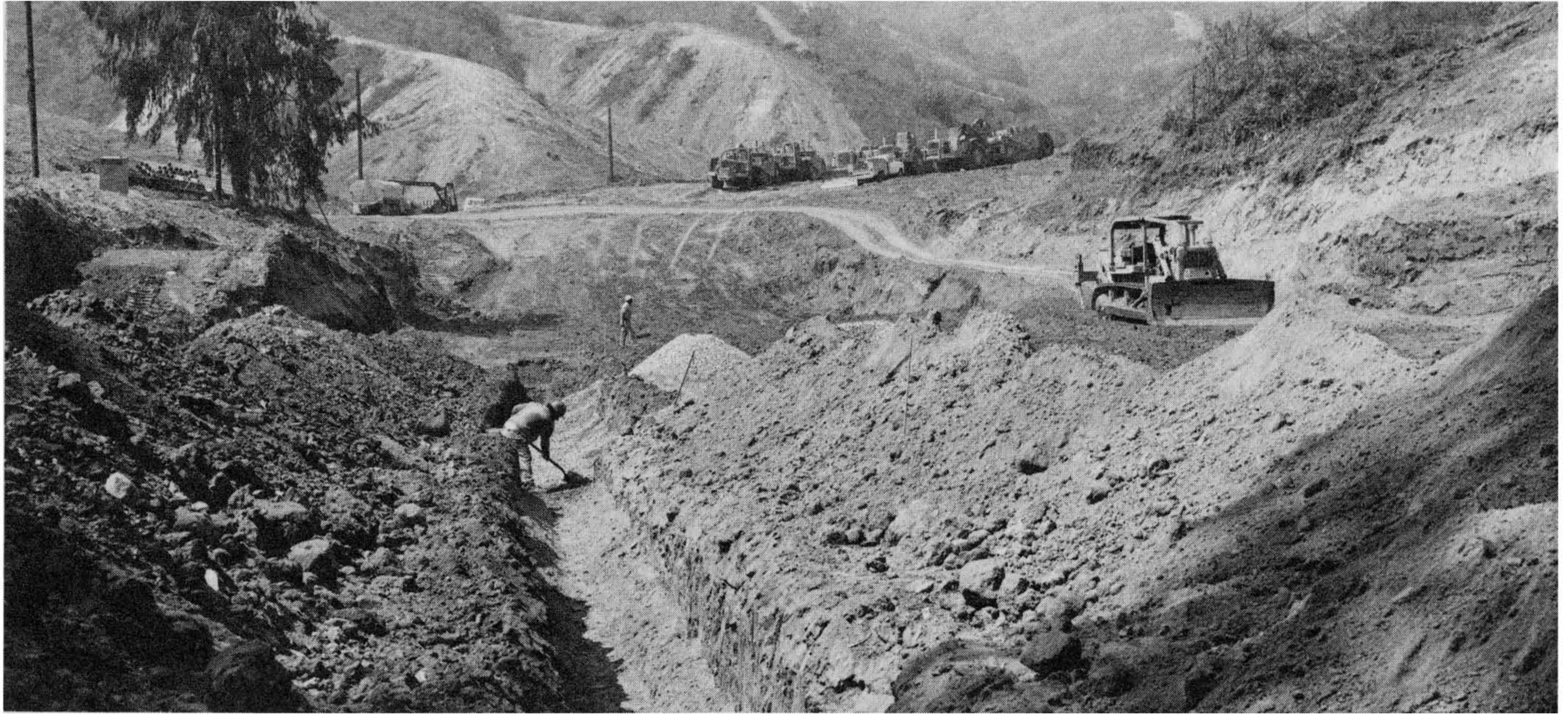
Figure 5-6 Subdrain excavation in progress within the main canyon. Equipment in the background awaits completion of subdrain construction prior to filling the canyon. Photograph courtesy of the Dept. of Building & Safety, City of Los Angeles, staff photographer John Shadle.
