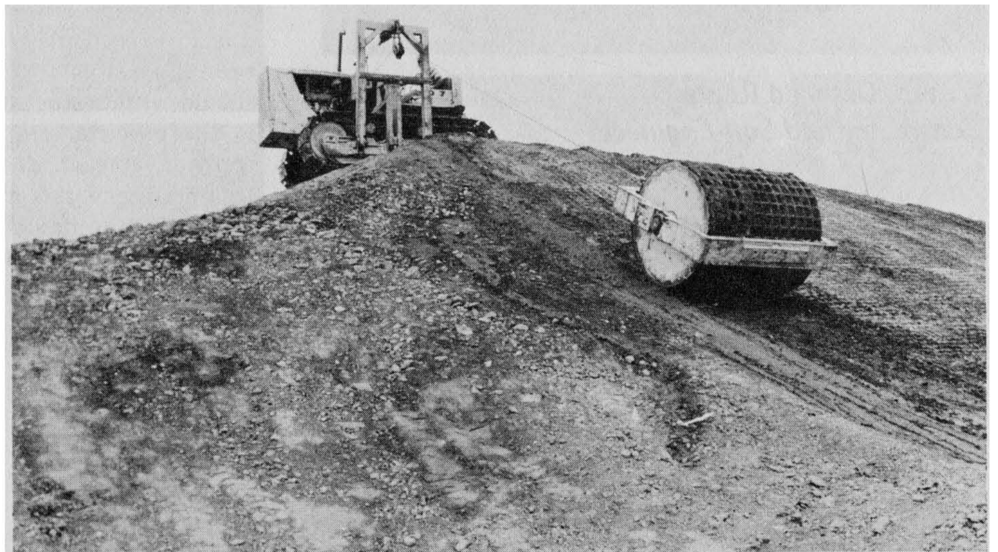
Figure 5-40 Gridrolling the fill slope after tractorwalking or sheepsfoot rolling compacts the outer 2-3 inches of the slope to form a crust which helps shed water rapidly. Photograph by C. Michael Scullin.
