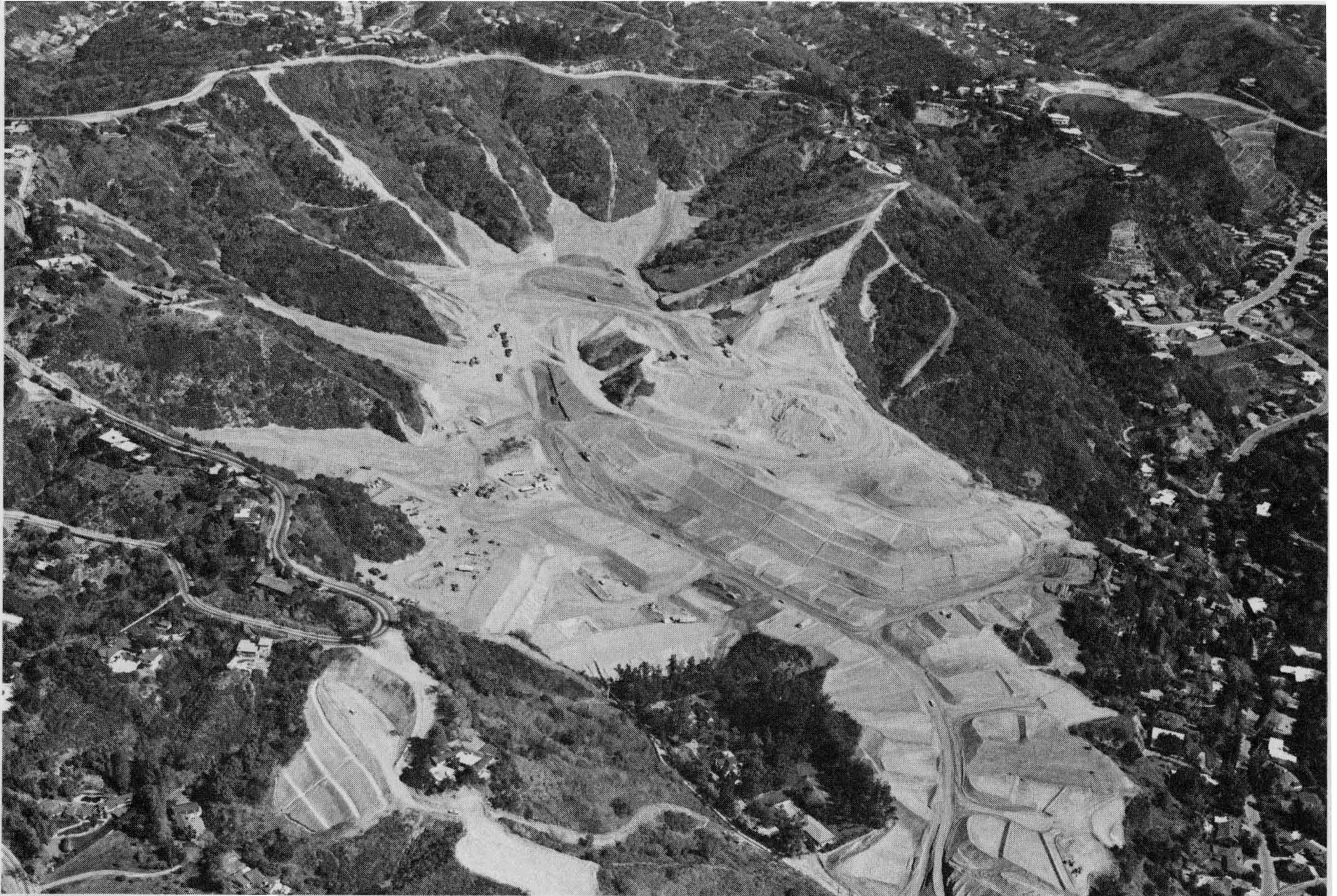
Figure 5-37 This grading operation is nearing rough-grade stage. Lot pad and streets are shown roughed out, slope terrace and down drains are paved, fill slopes are trimmed back and grid-rolled, and the desilting basin is roughed in. Photograph courtesy of the Dept. of Building & Safety, staff photographer John Shadle.
