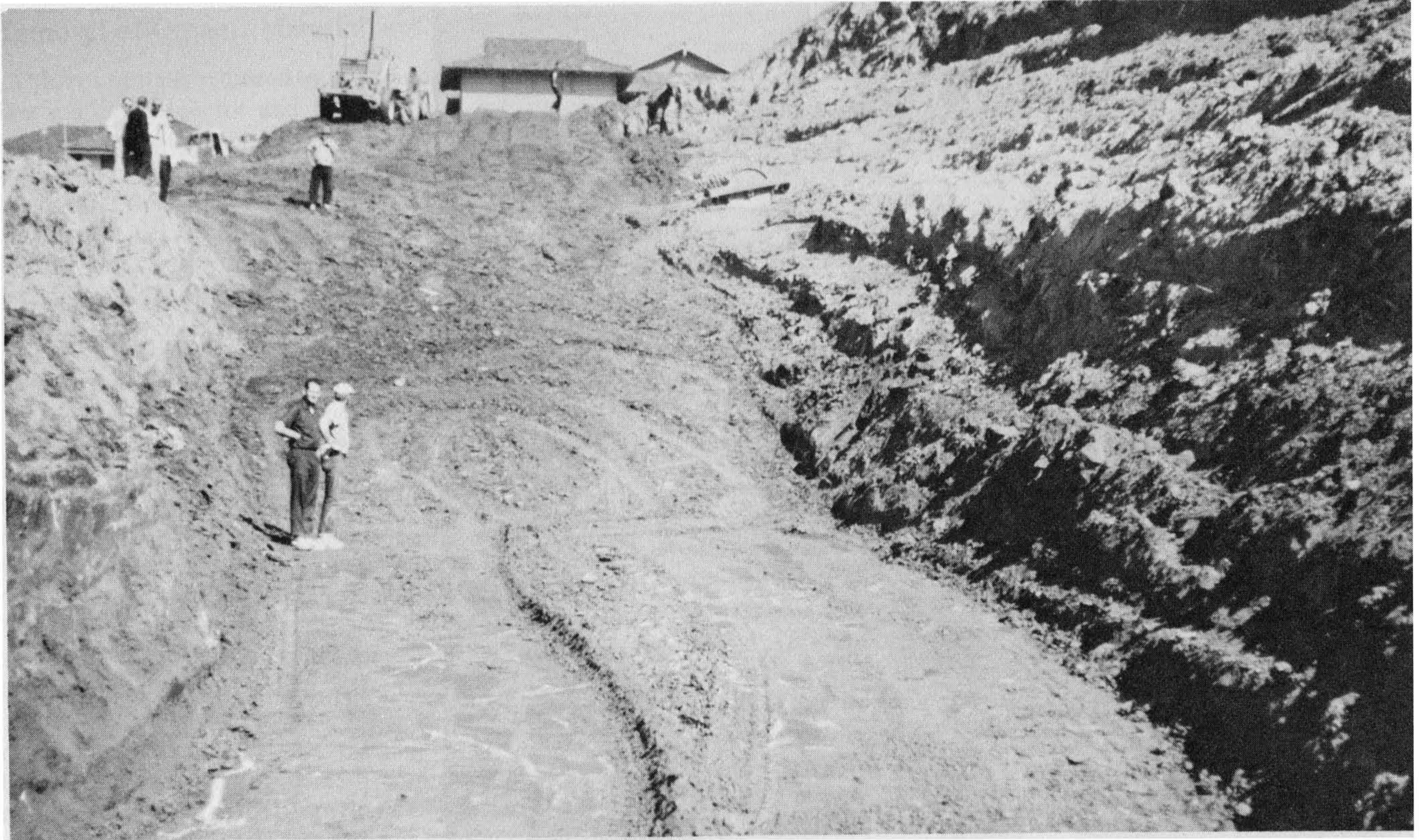
Figure 5-31 A lime stabilization buttress key excavation in gypsiferous siltstone is shown here. Notice the white gypsum seams and the gypsum-filled joints. Grading inspector Burdette Sanders, dark shirt, is shown inspecting the key. Photograph by and courtesy of Robert W. Ross.
