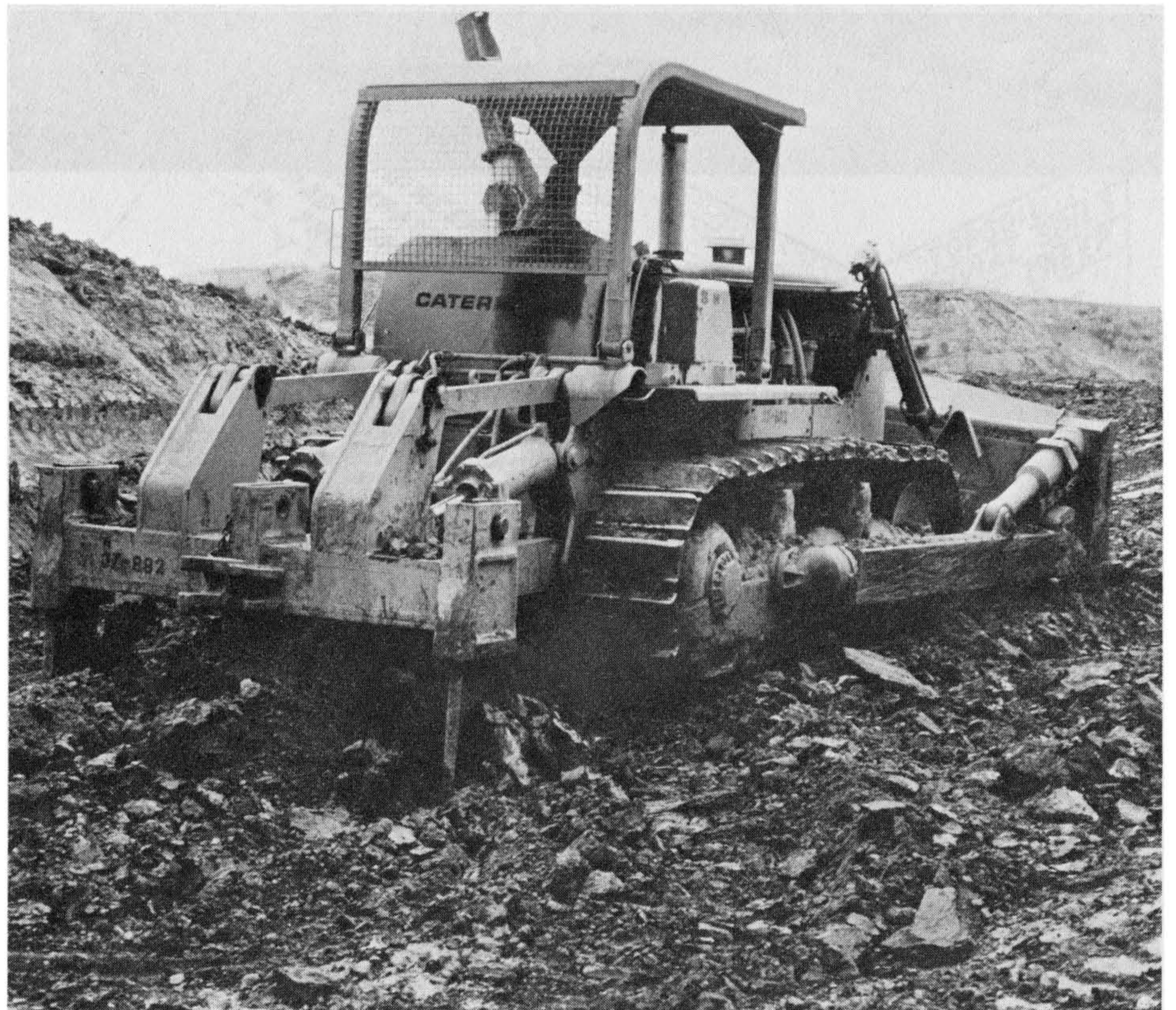
Figure 5-20 Ripping the cut area with double shank rippers. Photograph by C. Michael Scullin.
