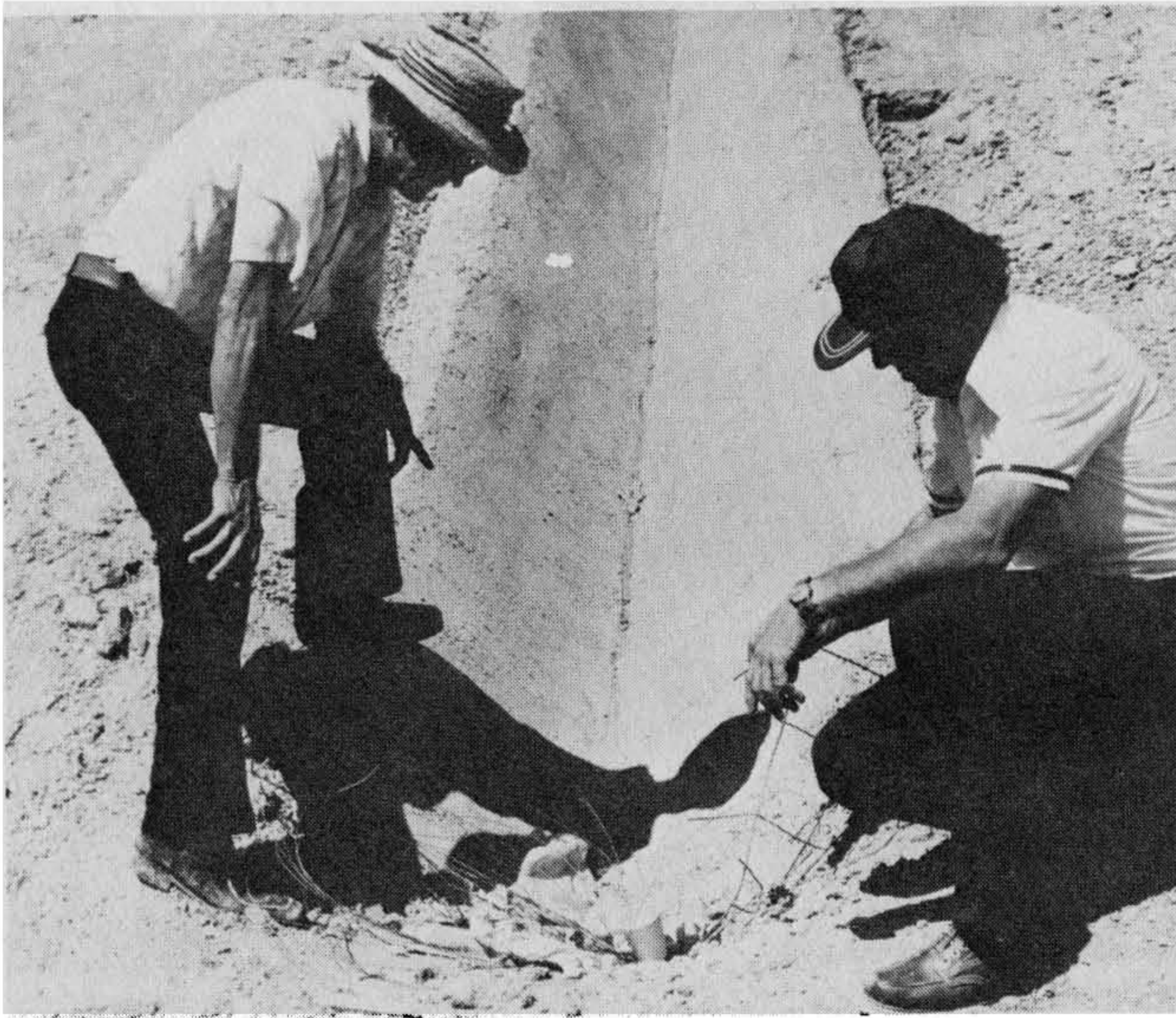
Figure 5-52 Robert J. Guilmette, senior grading inspector (left), and Sam Lawmaster, district grading inspector (right) County of Orange, CA, inspect this down drain construction. Photograph by C. Michael Scullin.
