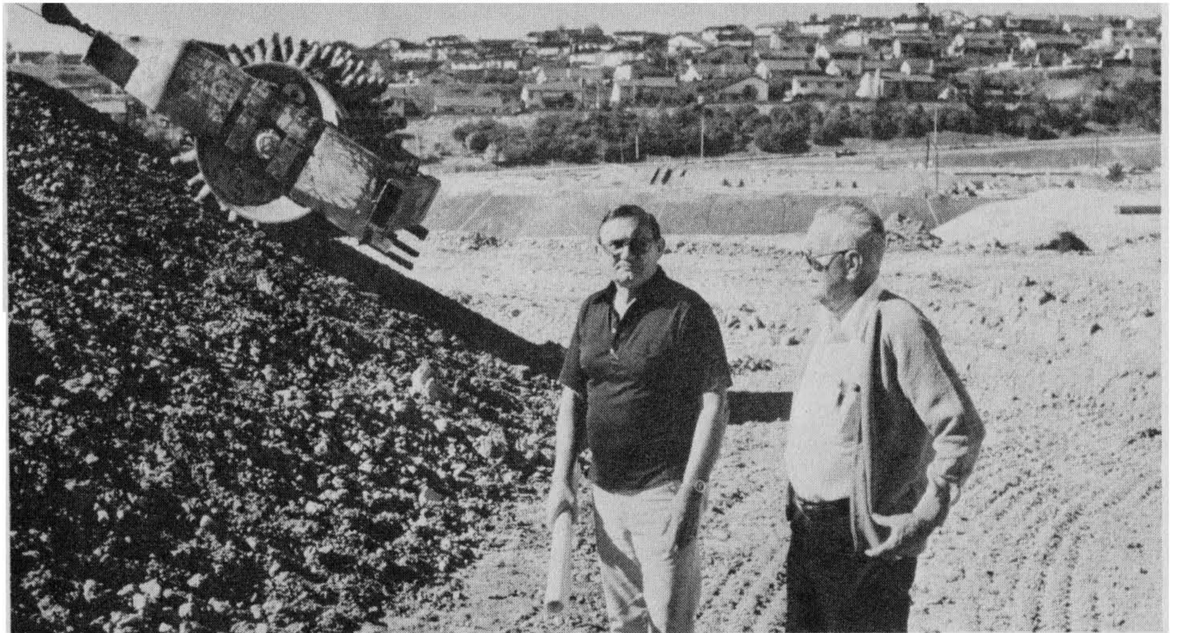
Figure 5-39 Jess Riddle, left, general superintendent of earthwork construction, Mission Viejo Company, and John H. Douglas, right, district grading inspector, County of Orange, California, inspect this slope-rolling operation. A sheeps-foot roller is cabled up and down the slope here prior to grid-rolling. Photograph by C. Michael Scullin.
