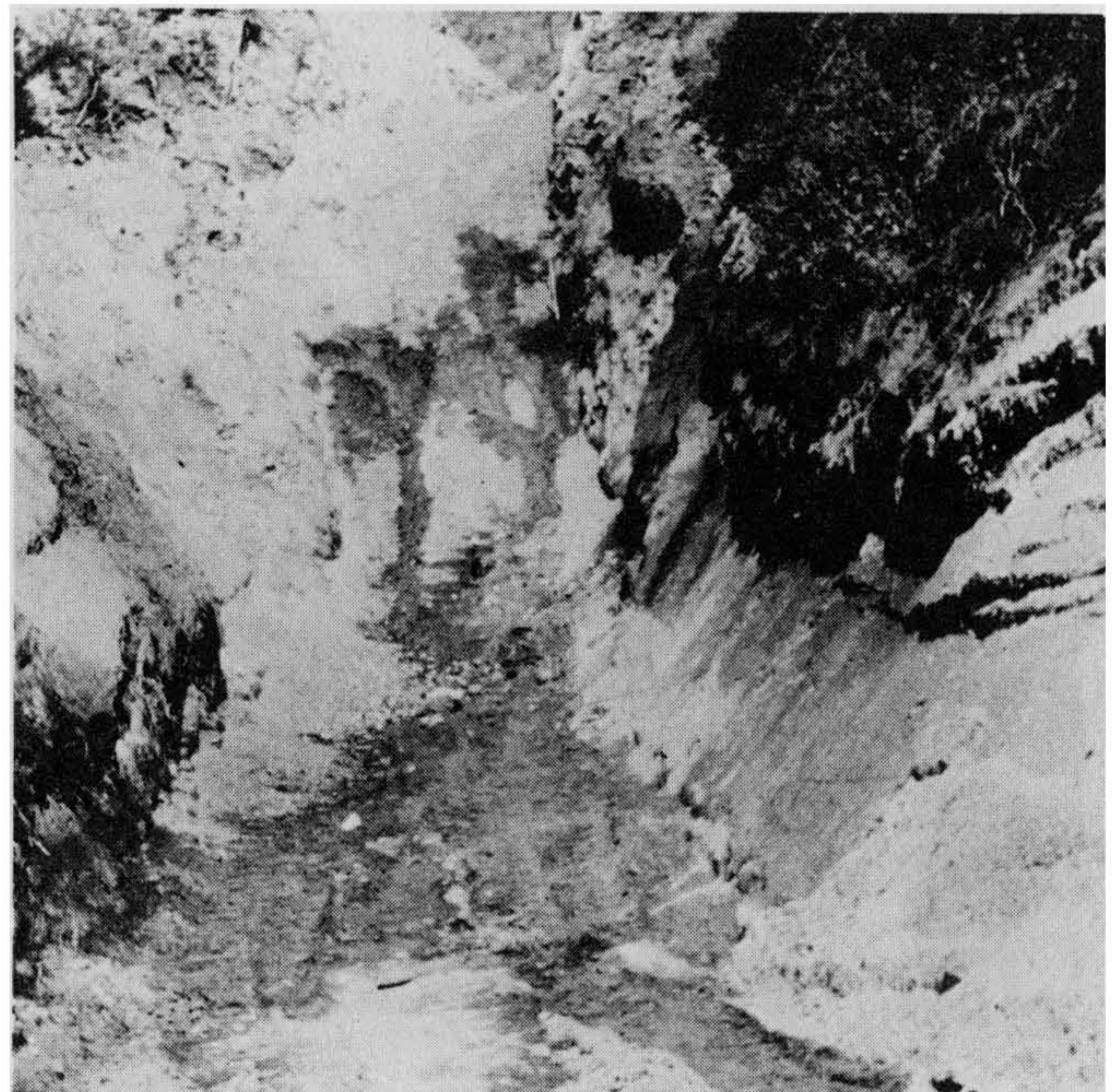
Figure 5-8 Seepage build-up during lateral canyon clean-out requires subdrain construction. Photograph by and courtesy of James E. Slosson.
