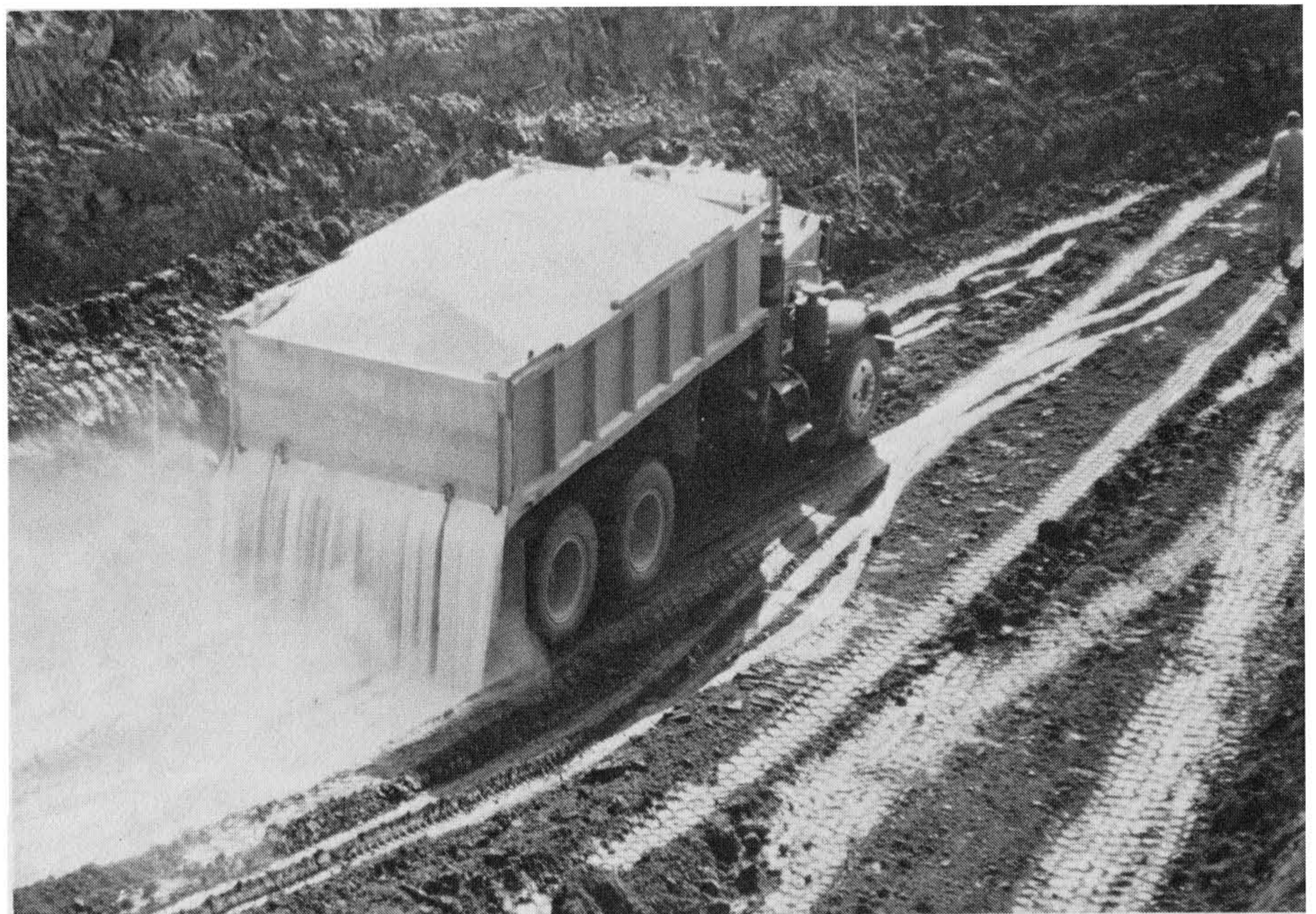
Figure 5-32 Laying lime in the buttress key. Photograph by and courtesy of Robert W. Ross.
