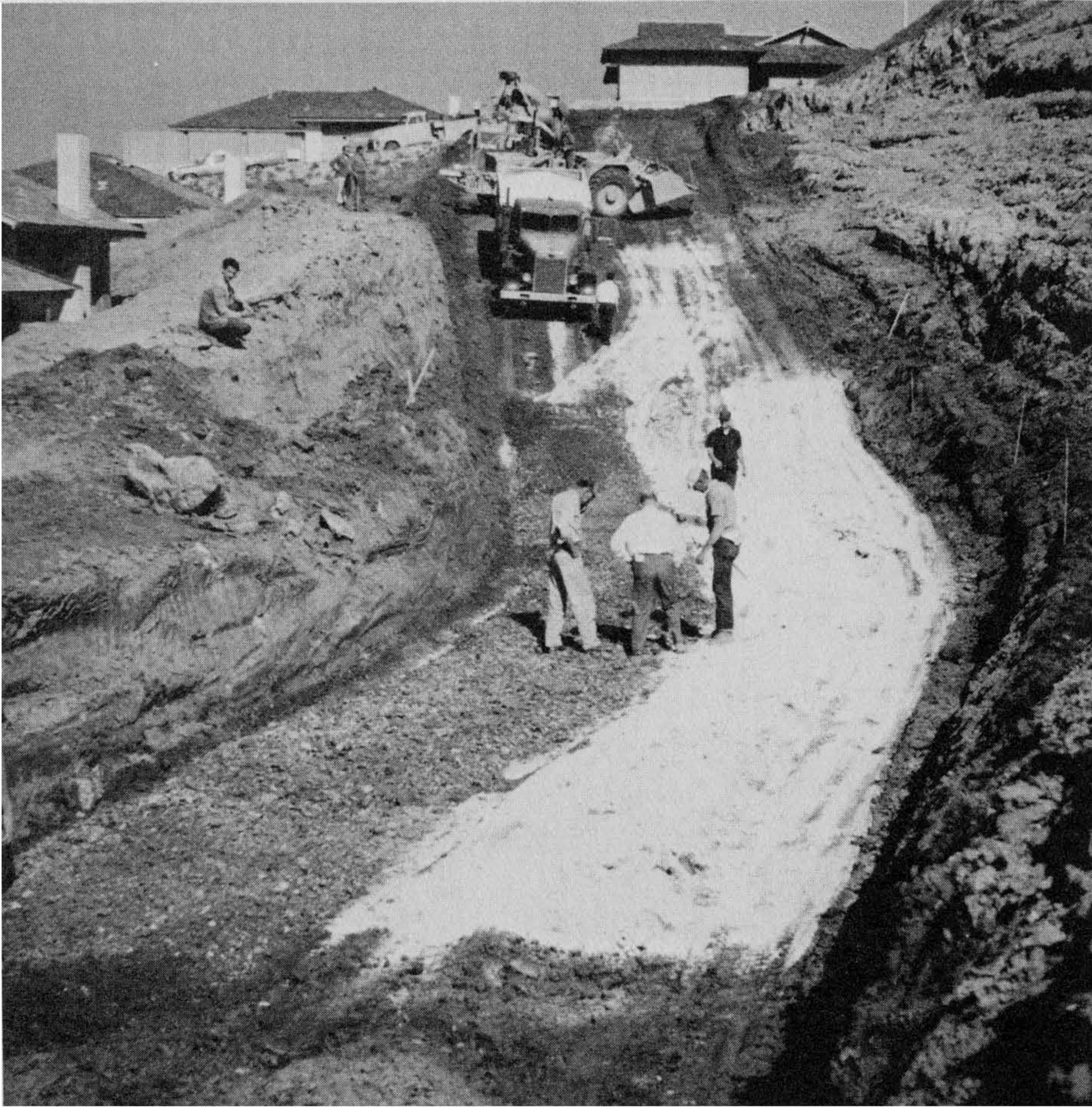
Figure 5-33 Grading contractor, James E. Stephenson, Anaheim, CA, and the soil engineer check the thickness of lime in the key. Photograph by and courtesy of Robert W. Ross.
