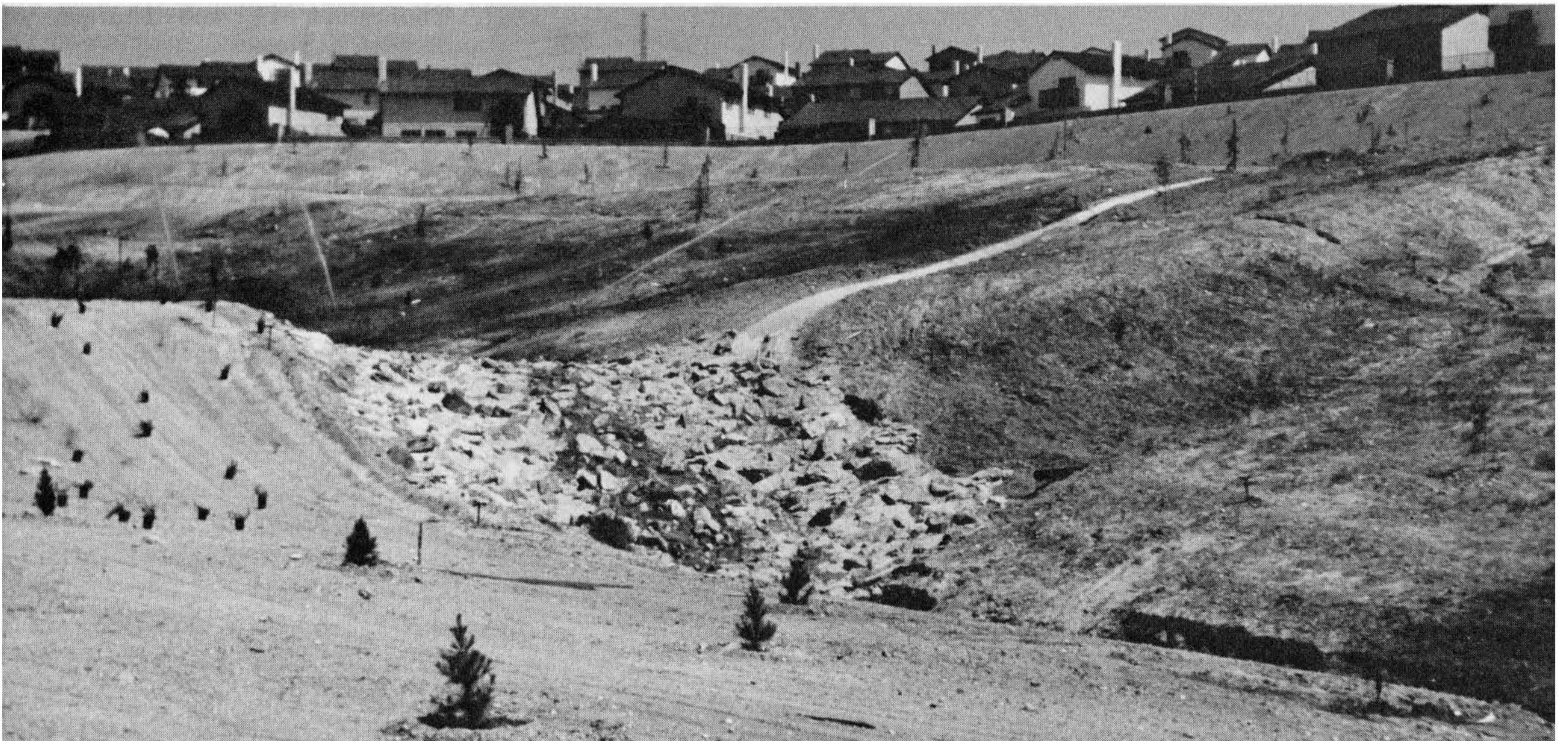
Figure 5-62 Canyon bottom drop structure composed of concreted rip rap. Sideslope and right-of-way landscaping are in progress. Photograph by C. Michael Scullin.
