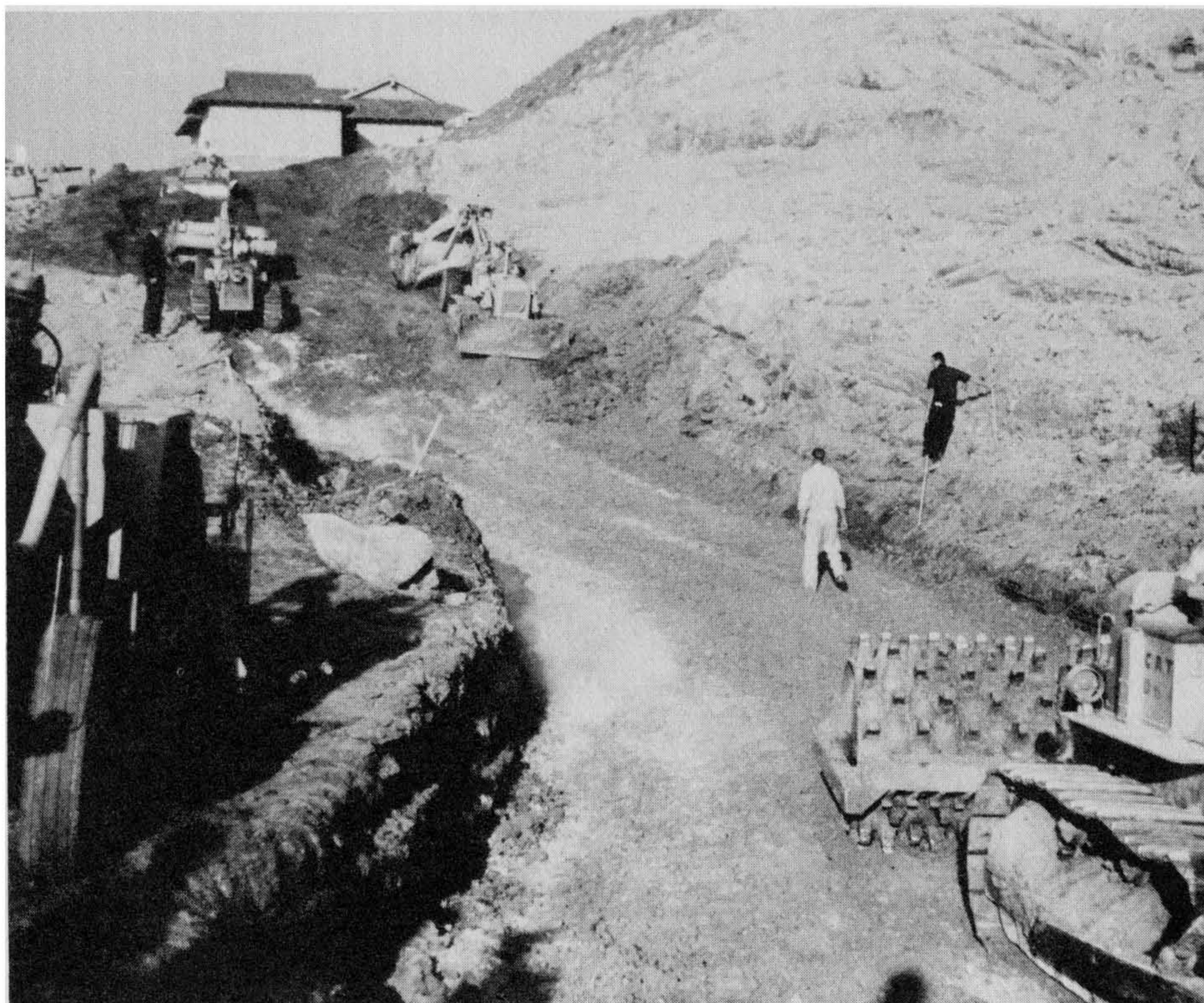
Figure 5-34 Mixing and compacting backfill and lime in the buttress key. Photograph by and courtesy of Robert W. Ross.
