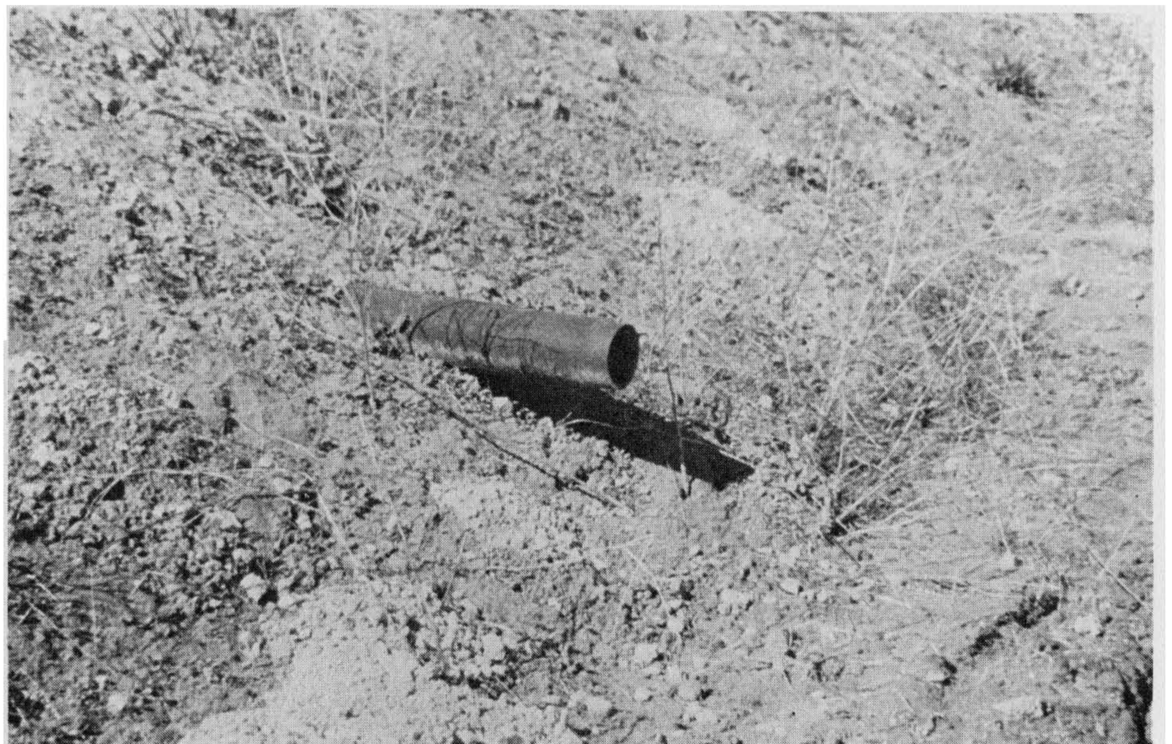
Figure 5-35 Subdrain outlet at the toe of a rough-graded fill slope. This fill slope needs to be finished; however, the subdrain outlet is properly exposed with an outlet above the toe of slope. Photograph by C. Michael Scullin.
