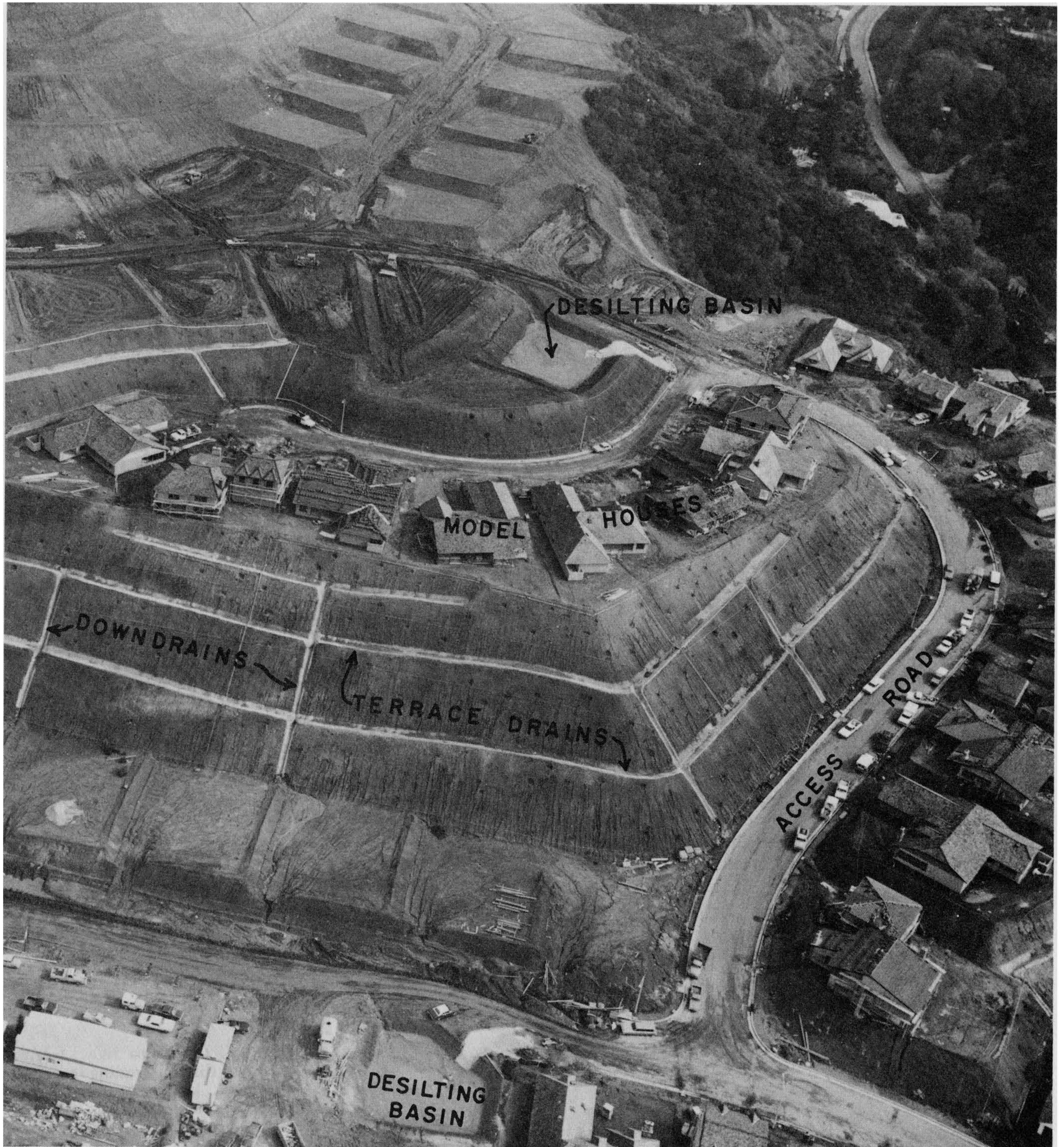
Figure 5-60 Rough-grade stage nears completion. Slope terrace and down drains are complete except for outlet structures. The model houses are under construction; the access road is paved; smaller desilting basins are complete and slope planting is in progress. Photograph courtesy of the Dept. of Building & Safety, City of Los Angeles, staff photographer John Shadle.
