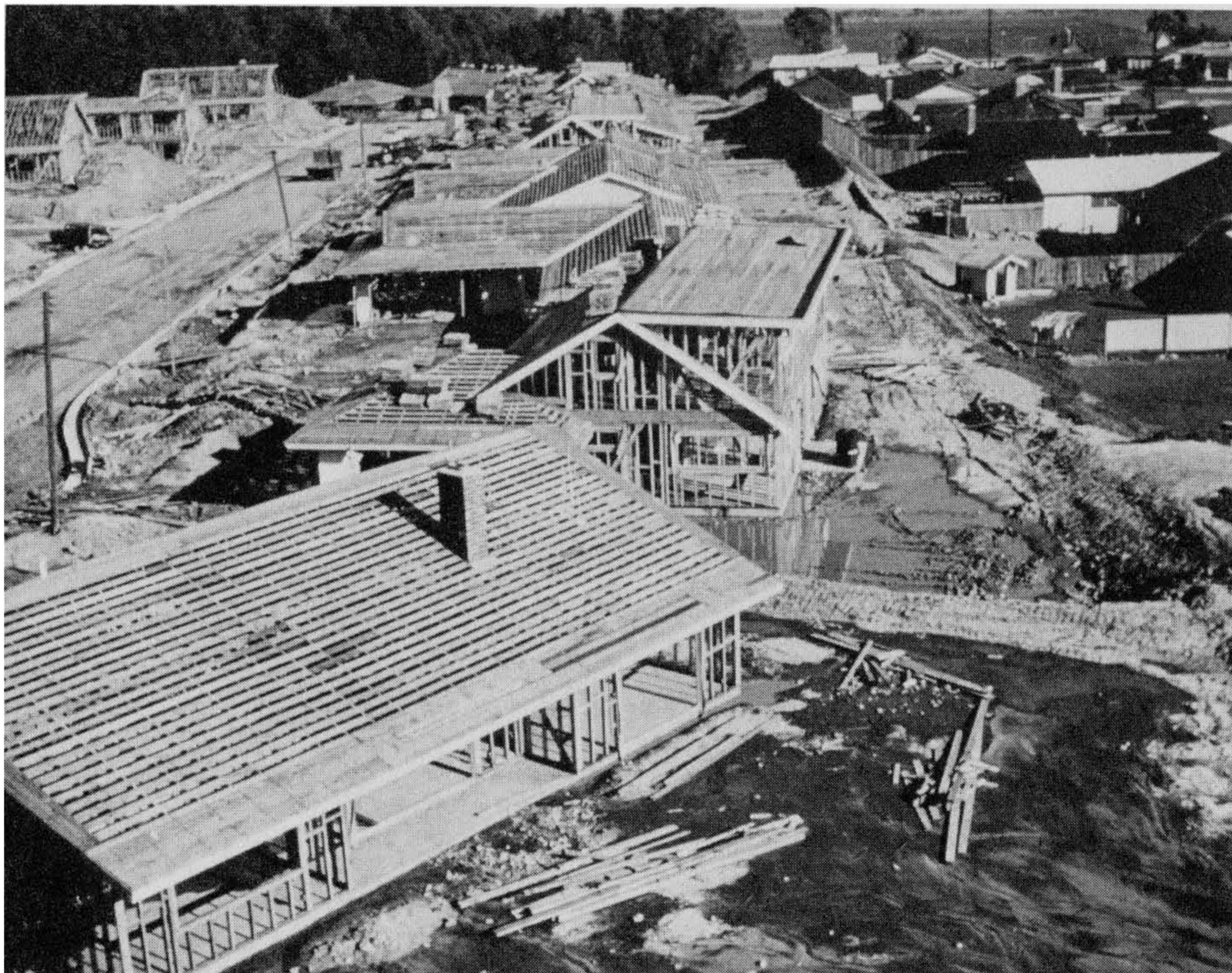
Figure 5-63 Poor drainage control during house construction is shown here. Water is ponding in the rear, front, and side yards and next to the footings. Utility trenches are eroding in the front yards. This is a good example of poor drainage control during house construction. Photograph by and courtesy of Robert W. Ross.
