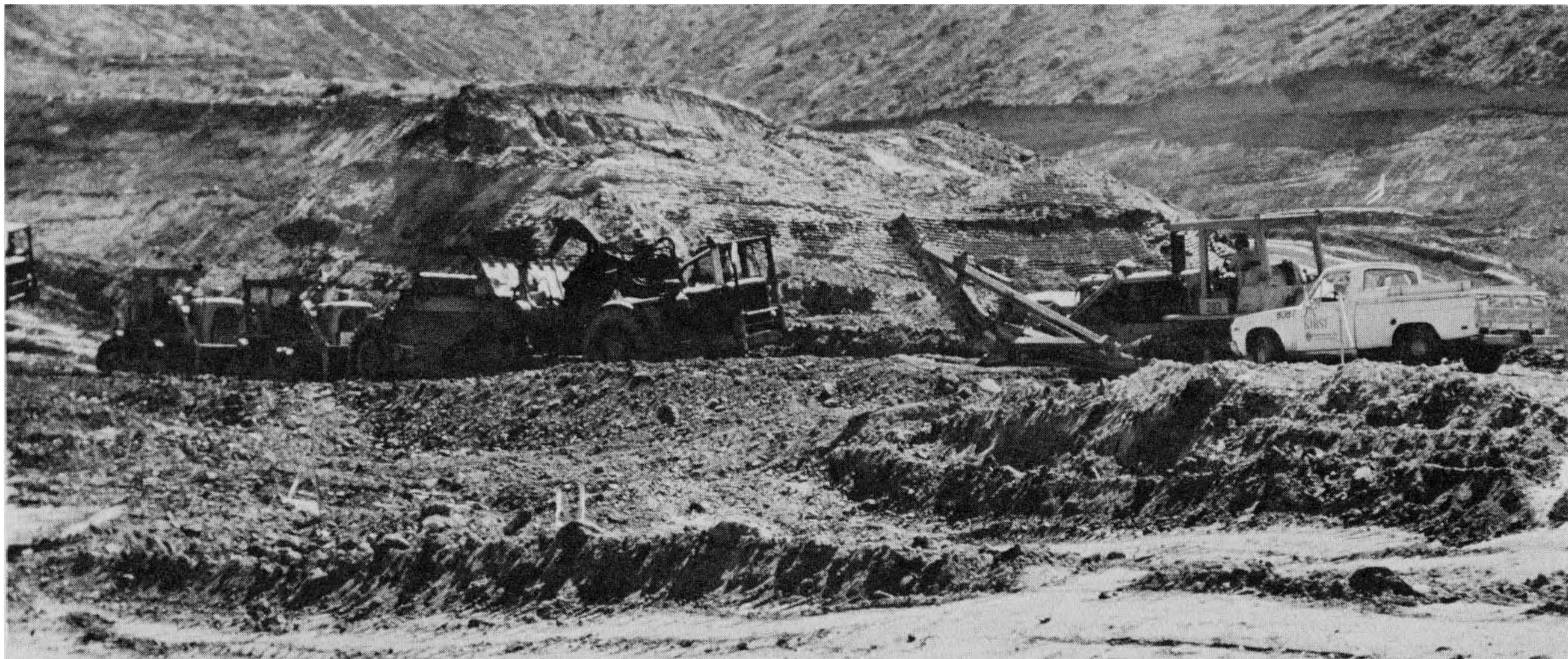
Figure 5-14 Sidewall benches are being excavated during canyon cleanout. These sidewall benches are 15-20 ft. high and are well into competent bedrock. At right, the dozer with a slope-bar is cutting the sidewall benches while scrapers load the material. Photo by C. Michael Scullin.
