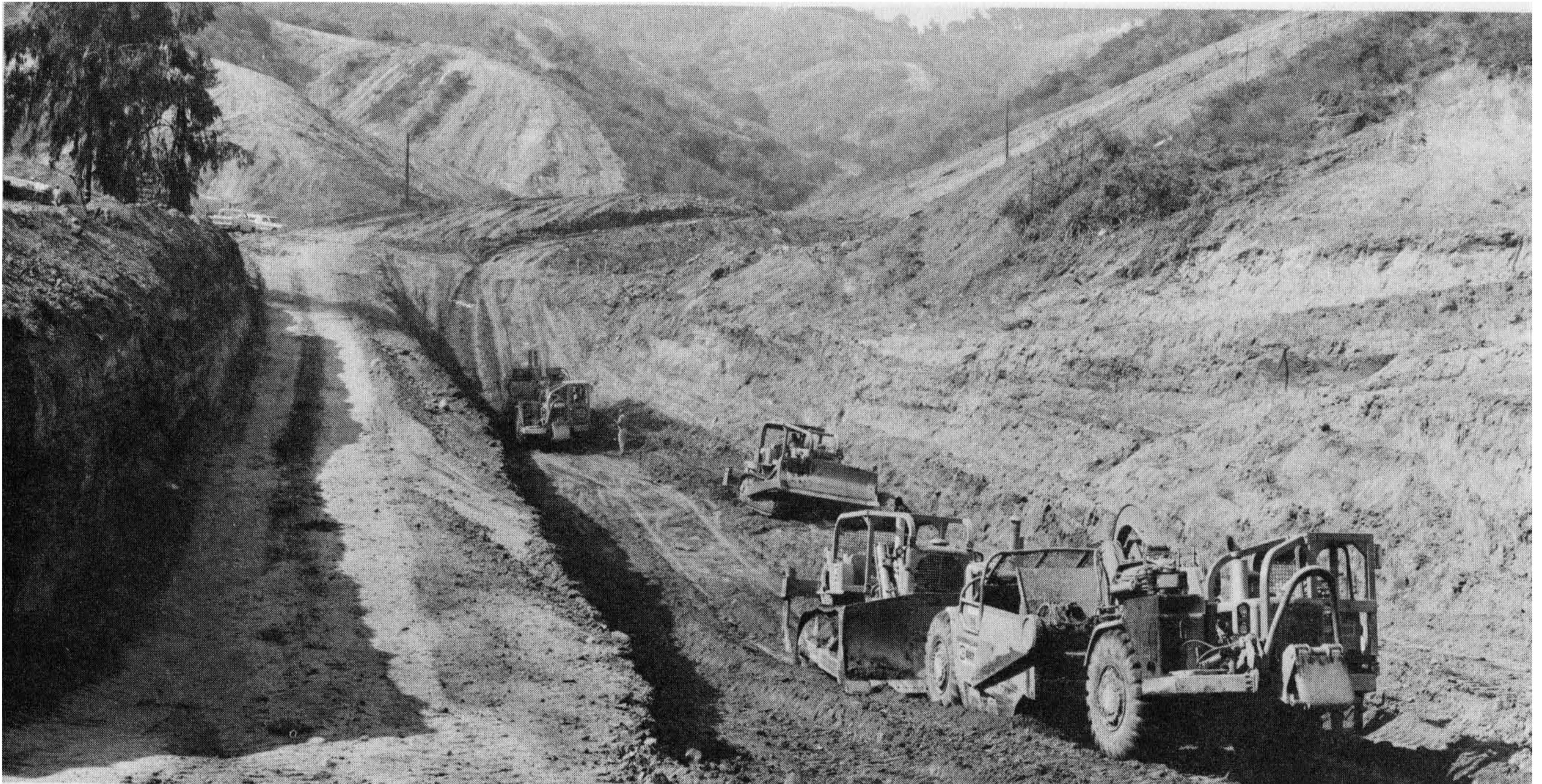
Figure 5-3 Canyon bottom clean-out continues, using ripper-cats and scrapers to remove compressible soils. Photograph courtesy of the Dept. of Building & Safety, City of Los Angeles, staff photographer John Shadle.
