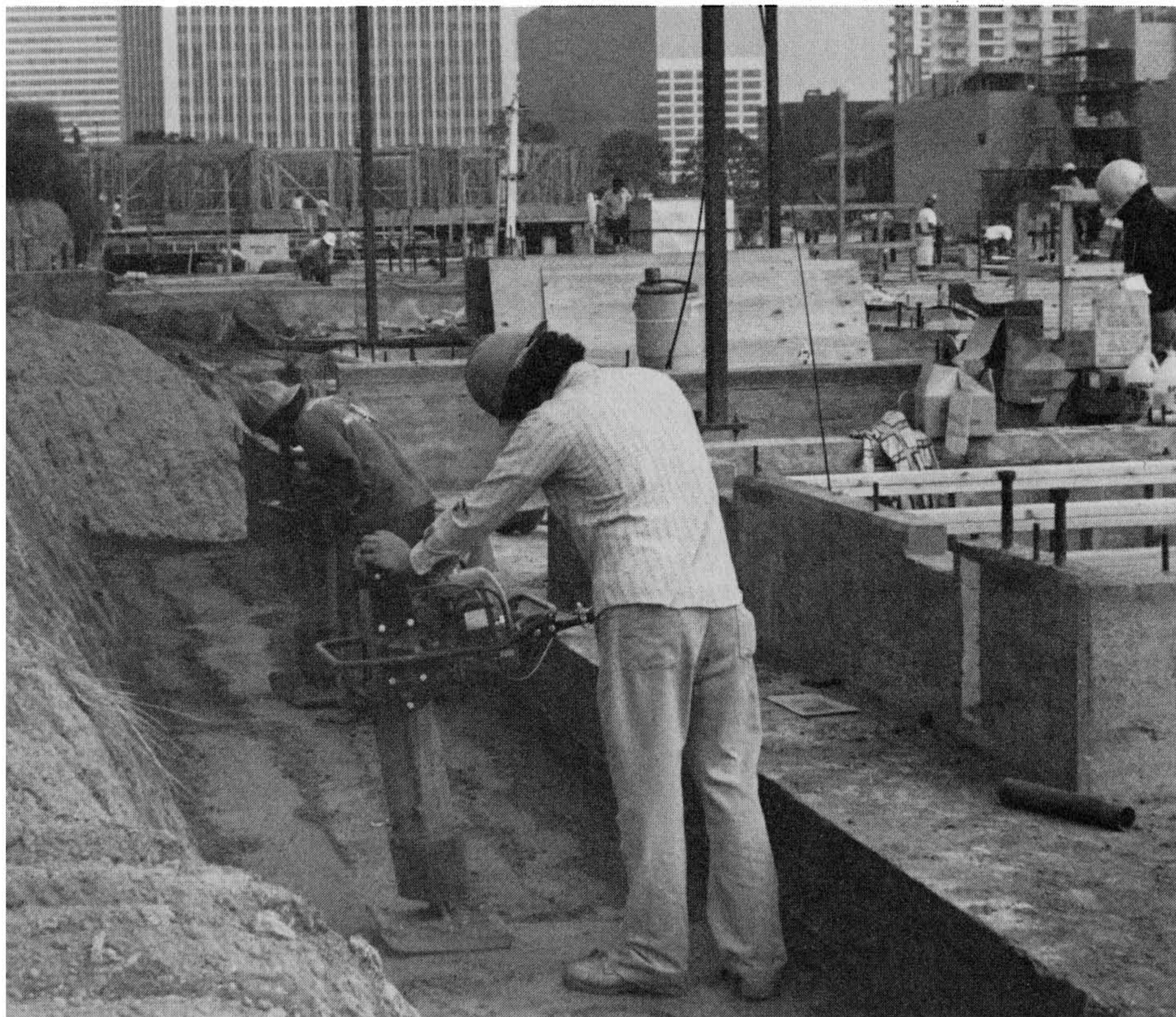
Figure 5-42 A Barco compactor is used here to compact or "tamp" backfill at the rear of a basement-wall. Photograph by Leopold Hirschfeldt, courtesy of LeRoy Crandall & Associates.
