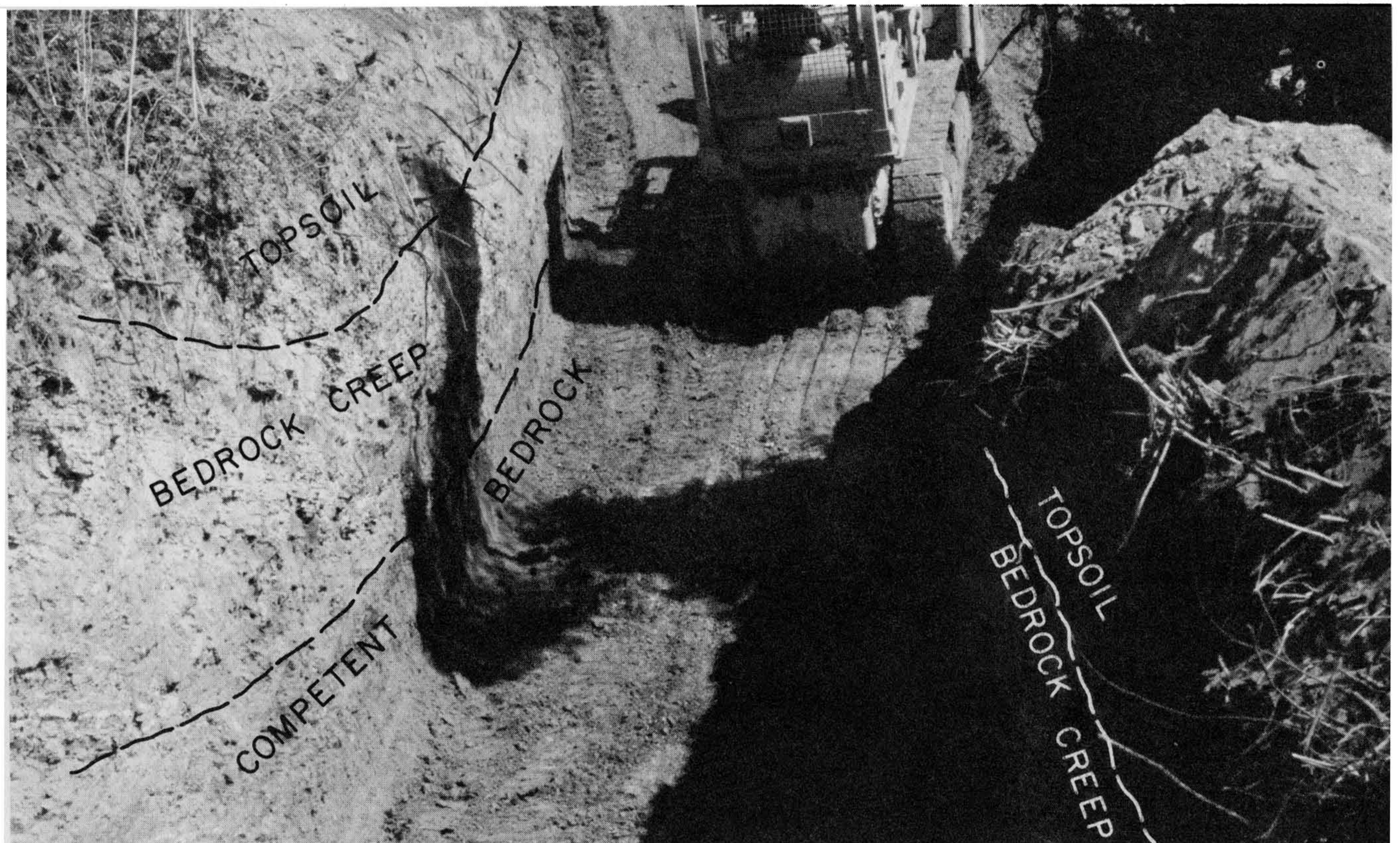
Figure 5-28 Toe-of-fill key excavation in progress for a sidehill fill. Both photos by C. Michael Scullin.
