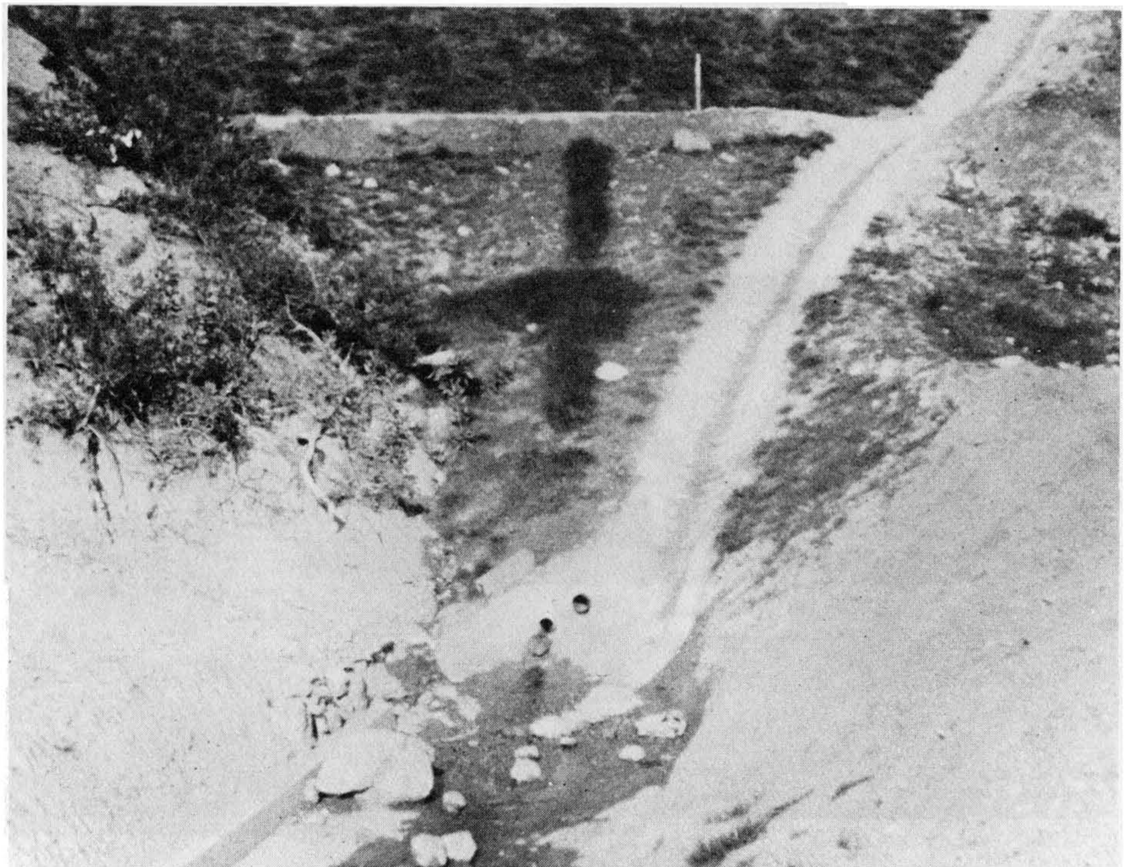
Figure 5-56 A completed lateral canyon fill slope is shown with paved terrace drains and a down drain constructed down the "day-light" line of the fill. Note seepage from subdrains into the drainage channel. Photograph by and courtesy of James E. Slosson.
