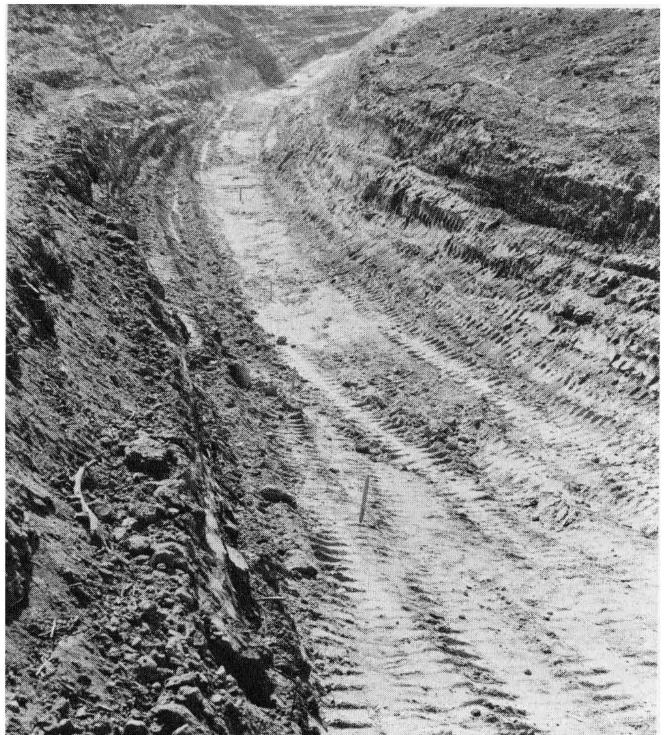
Figure 5-5 This lateral canyon has been cleaned out and staked for subdrain trenching. Photograph courtesy of the Dept. of Building & Safety, City of Los Angeles, staff photographer John Shadle.
