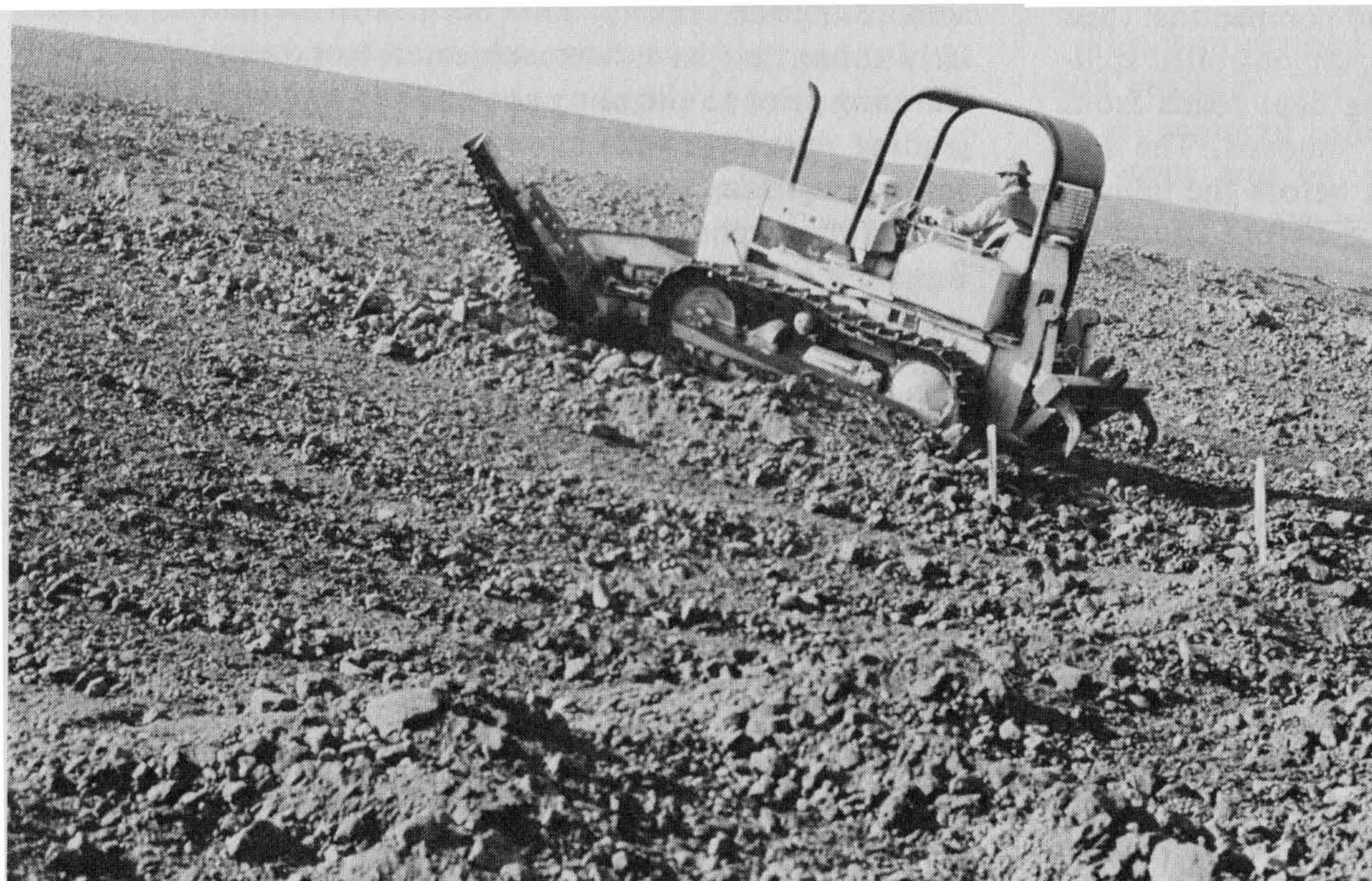
Figure 5-38 Here a bulldozer is "tractor-walking" the fill slope to trim loose material and compact the surface. This operation is followed by side-booming a sheeps-foot roller, then grid-rolling to tighten the surface of the slope. Photograph by C. Michael Scullin.
