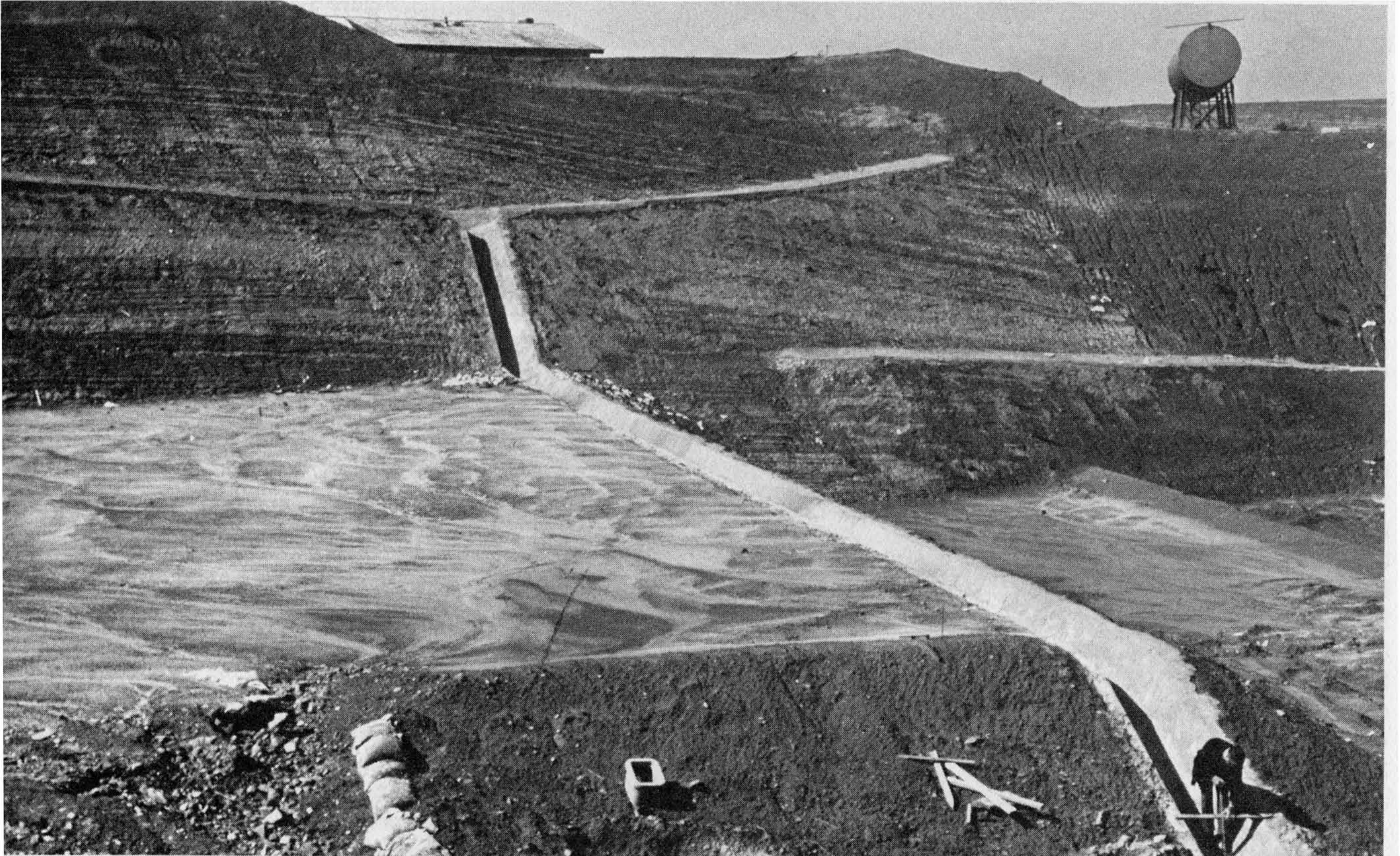
Figure 5-55 Kenyon H. Carr, senior grading inspector, West Los Angeles office, inspects and measures the width and depth of a slope down drain at rough grade stage. Photograph by Alex Bruce, senior building inspector, City of Los Angeles, CA.
