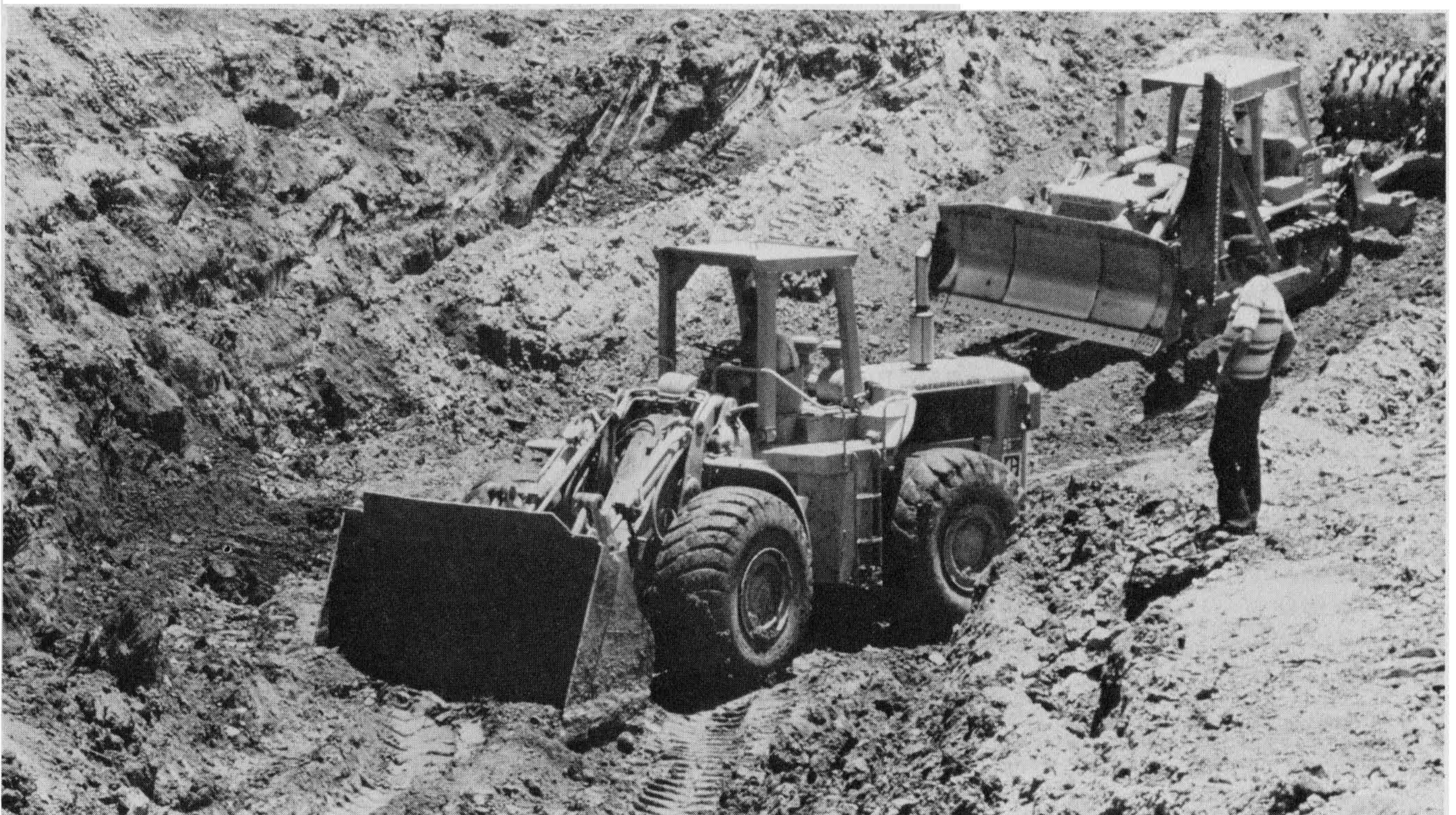
Figure 5-11 Toe-of-fill key backfill in progress. A rubber-tired loader is spreading fill material while compaction is accomplished by a sheepsfoot roller as a soil technician watches. Photograph by C. Michael Scullin.
