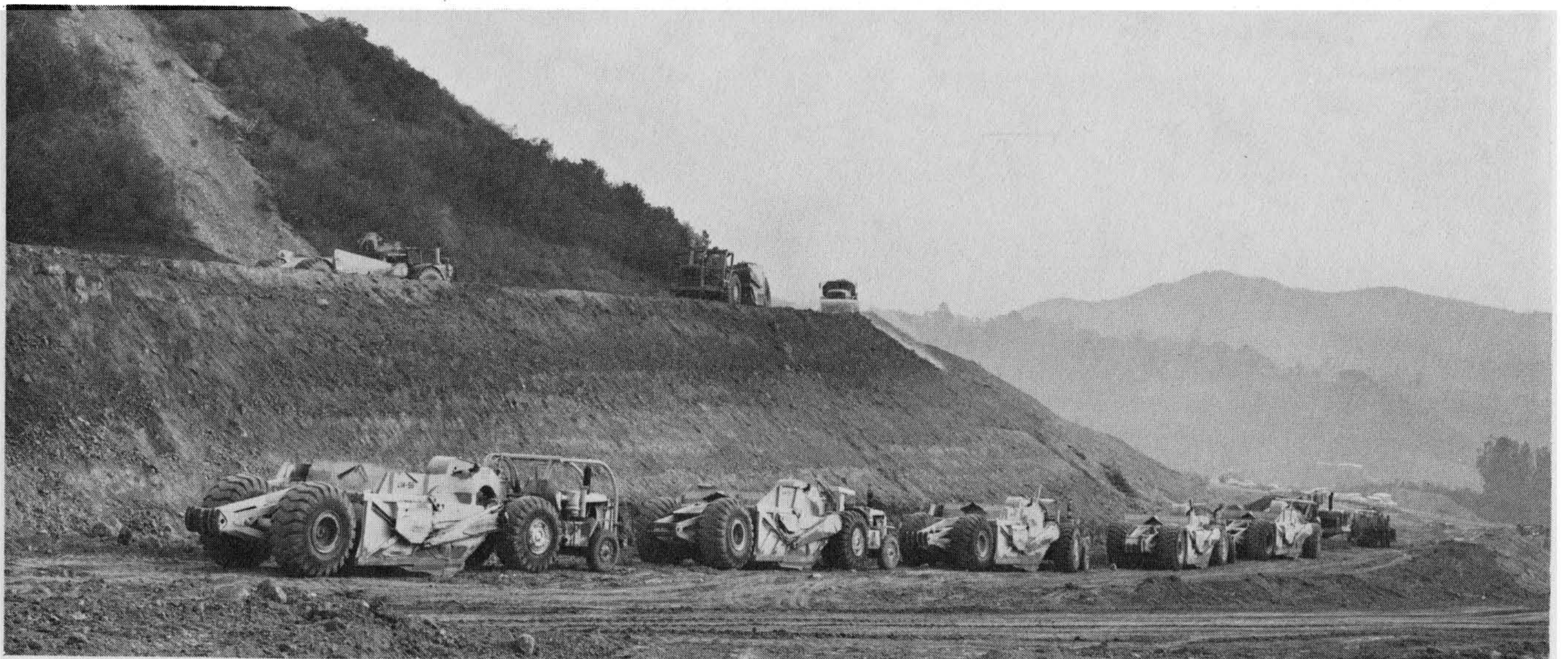
Figure 5-18 Fill-slope construction in progress. Scraper on the upper left is empty and is returning to the cut. The scraper upper center is hauling dirt to the fill site. The water truck is watering the slope. Photograph courtesy of the Dept. of Building & Safety, City of Los Angeles, staff photographer John Shadle.
