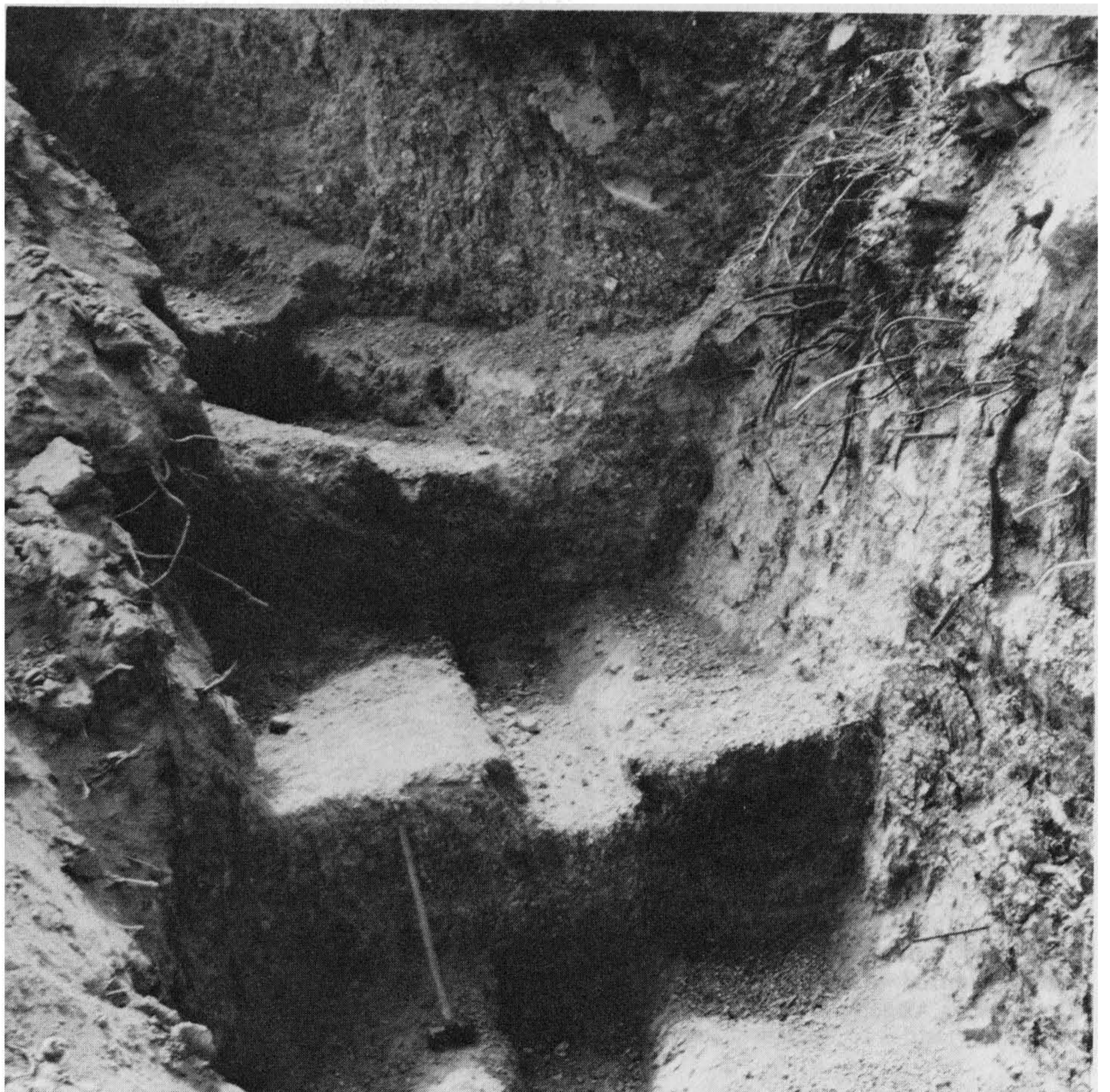
Figure 6-8 A retaining wall footing excavation is shown extended through loose soils and creep and founded on firm bedrock. Photograph by C. Michael Scullin.
