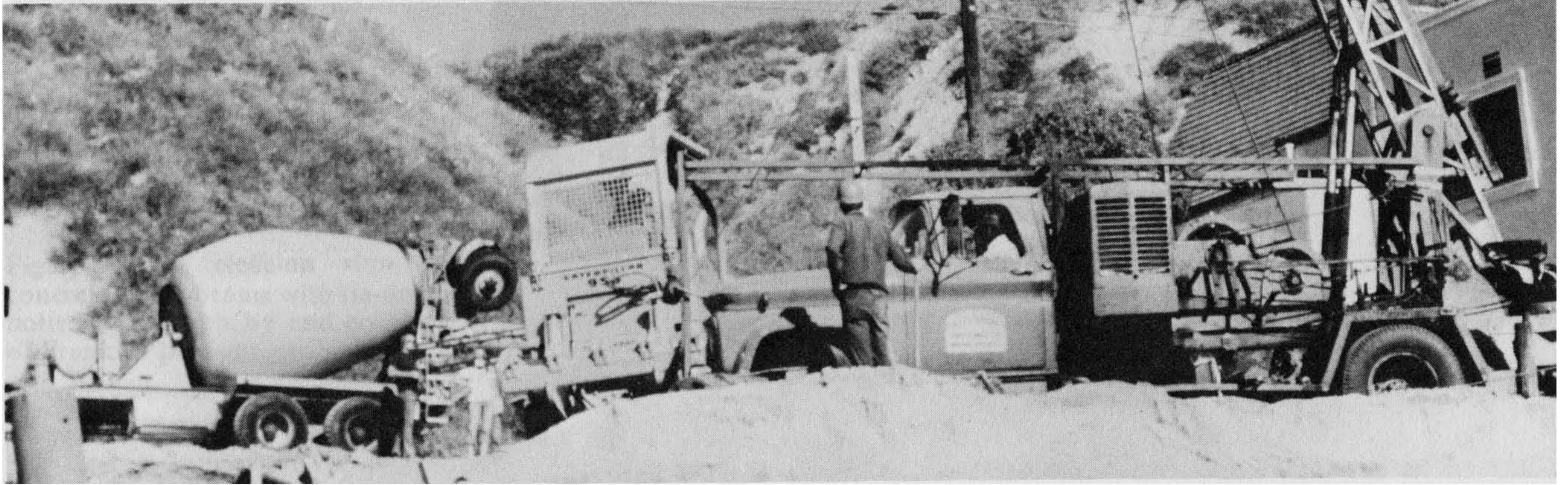
Figure 6-14 Constructing beachfront cast-in-place foundations. The bucket-auger drill rig (right) is pulling away from a completed hole. The concrete truck (left) is carrying a friction-pile cage. A temporary sand-fill has been graded for a work surface. Photograph by and courtesy of Frank E. Denison, geologist.
