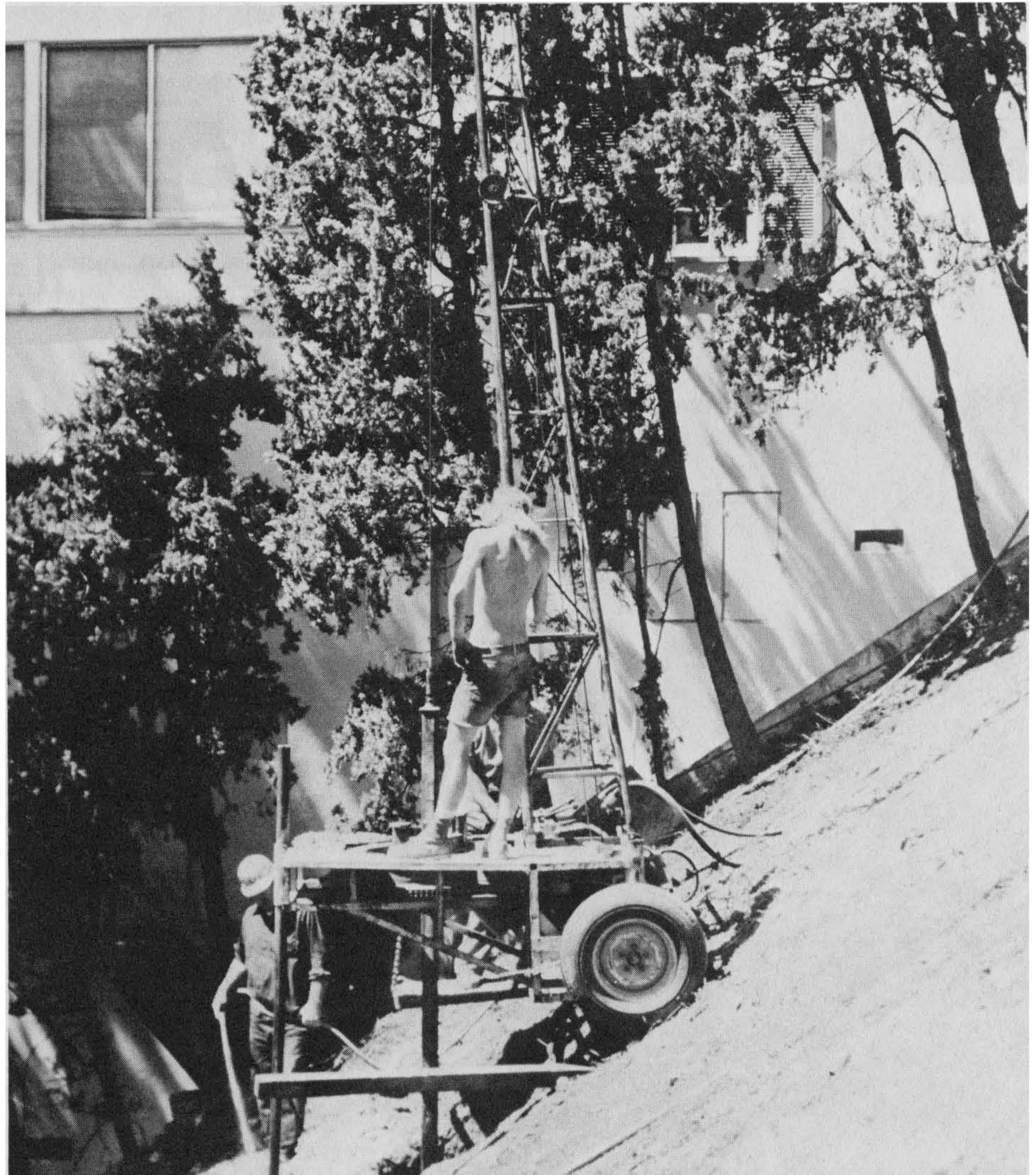
Figure 6-21 An improved hillside bucket-auger drill rig, driven by hydraulic fluid, is lowered downhill by hand and leveled with a “third leg.” The driller may add water to the cutting spoils to keep them from “running” out of the bucket. Photograph by and courtesy of Frank E. Denison, geologist.
