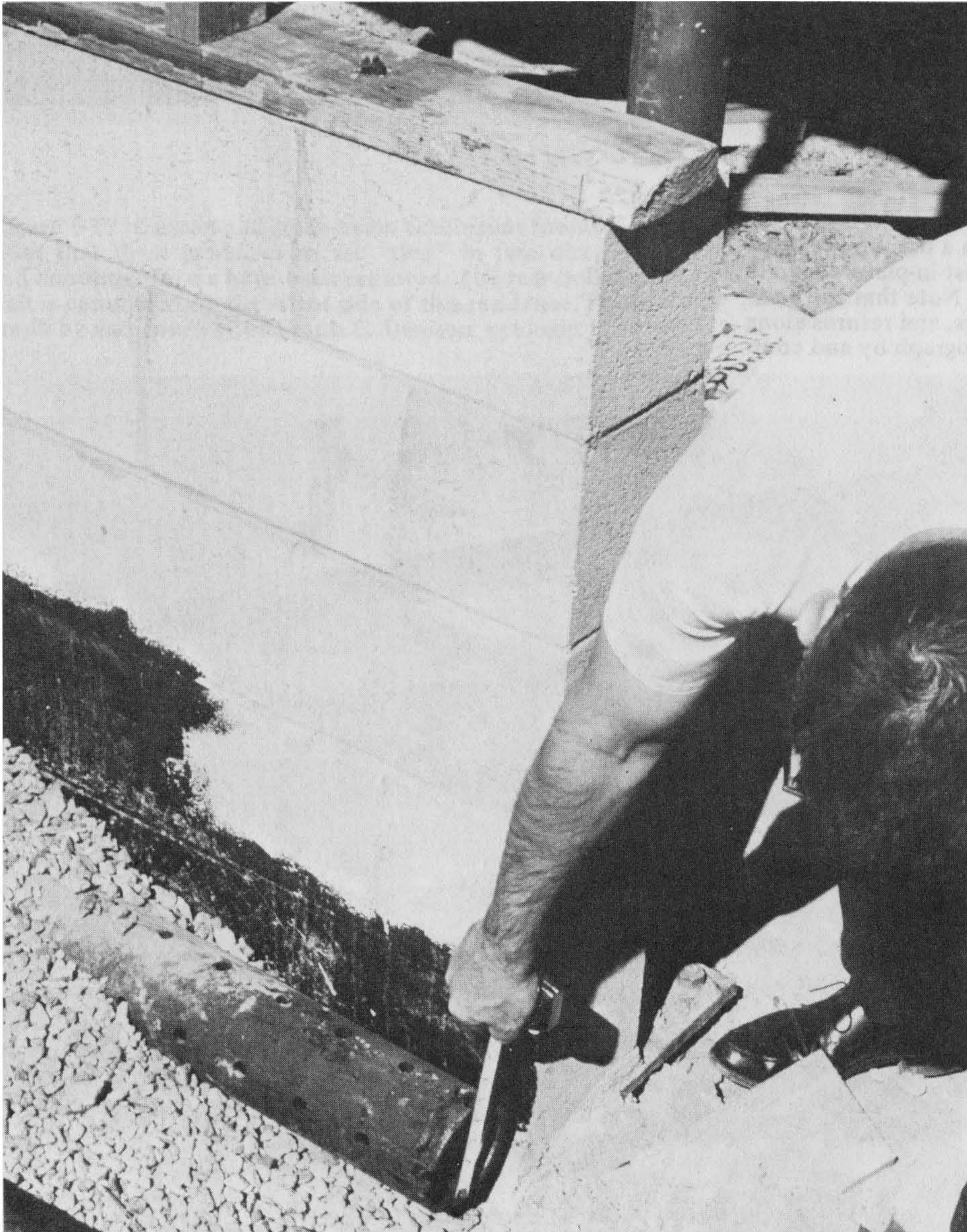
Figure 6-20 Subdrain along the sidewall of a residence. The wall and the cold joint between the wall and the footing must be sealed prior to placement of the subdrain. Subdrain pipe perforations should be faced downward . This photo shows the perforations up, which allows too much water to build up before draining and encourages siltation inside the pipe. Photograph by and courtesy of Alex Bruce, senior building inspector, City of Los Angeles.
