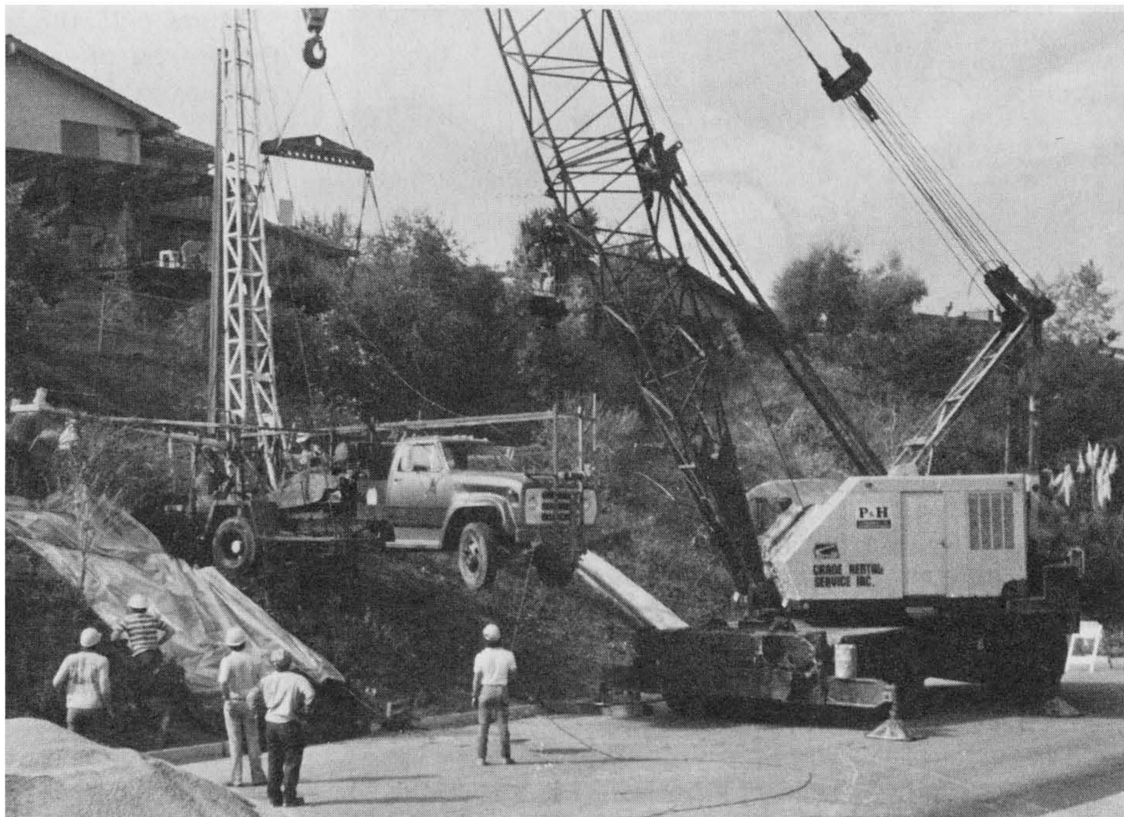
Figure 6-28 (a) A crane is used to lift a truck-mounted bucket-auger drill rig into position to drill a slope. The rig is held in place by the crane during drilling. (b) The dewatering casing (white) and slope indicator casing (dark) are being hoisted into the drill hole. They are held in place vertically and backfilled with pea gravel for permanent use. Photographs by and courtesy of Delmar D. Yoakum, GeoSoils, Inc. (c) The slope indicator casing (dark) and dewatering casing (white) are shown in place and capped for future use. Photographs by and courtesy of Delmar D. Yoakum, GeoSoils, Inc.
