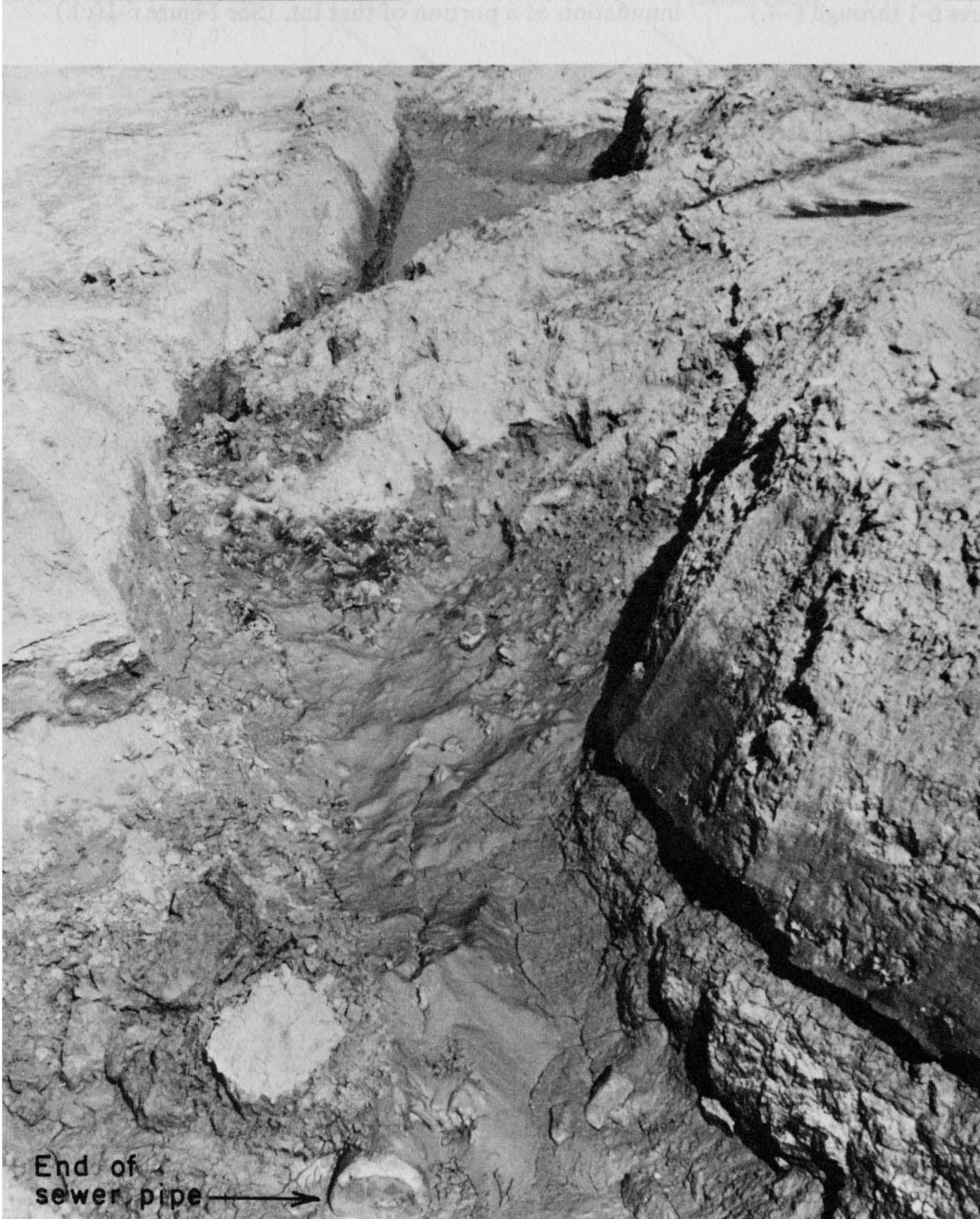
Figure 6-4 Loosely dumped backfill in sewer line trenches laid in the street area. These backfills are often compacted by water jetting which is rarely sufficient for adequate compaction and usually allows subsequent settlement. Photograph by C. Michael Scullin.
