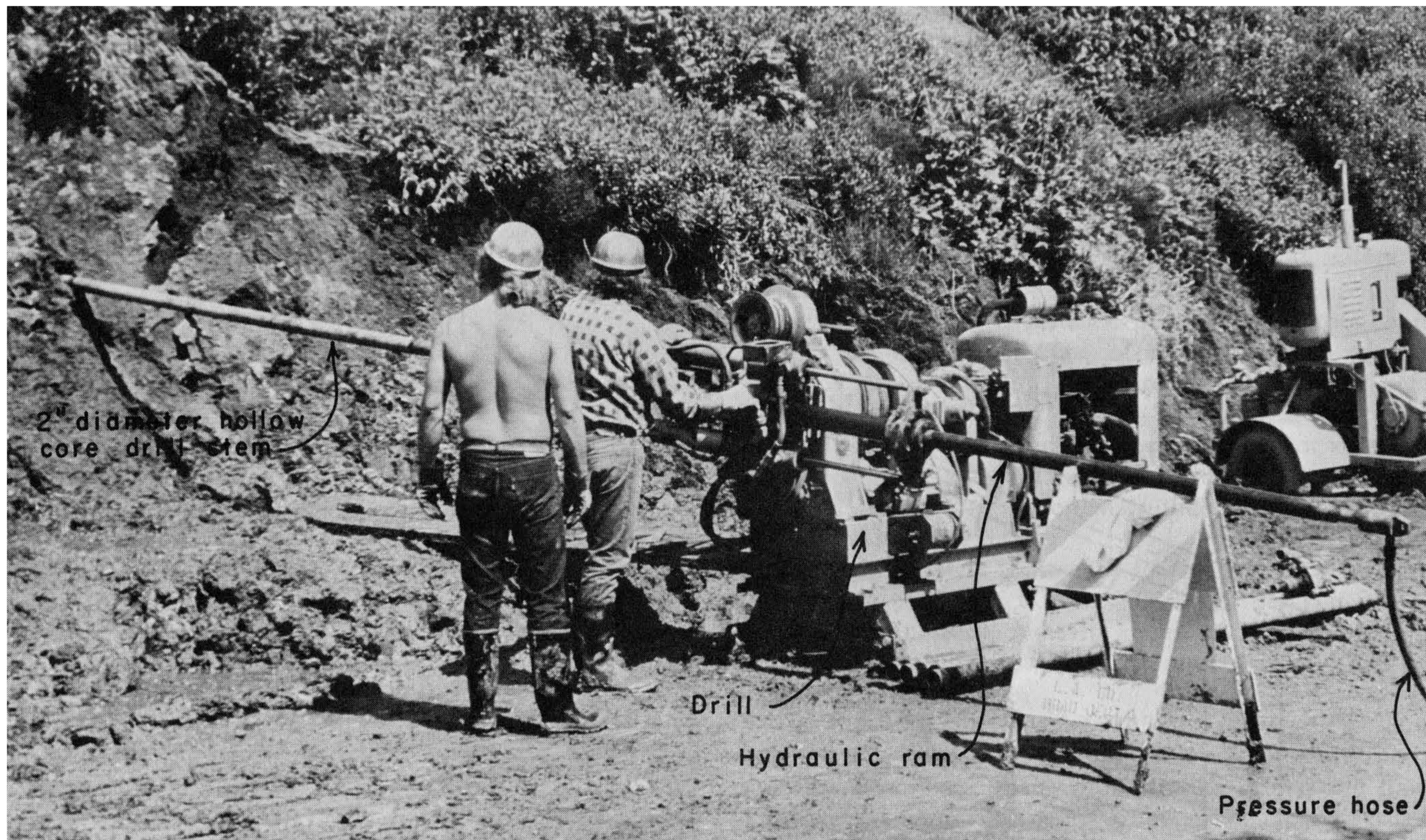
Figure 6-23 Drilling horizontal drains with a 2-in. diameter hollow-core drill stem and hydraulic ram. Water is used to advance the drill stem. Photograph by and courtesy of Frank E. Denison, geologist.
