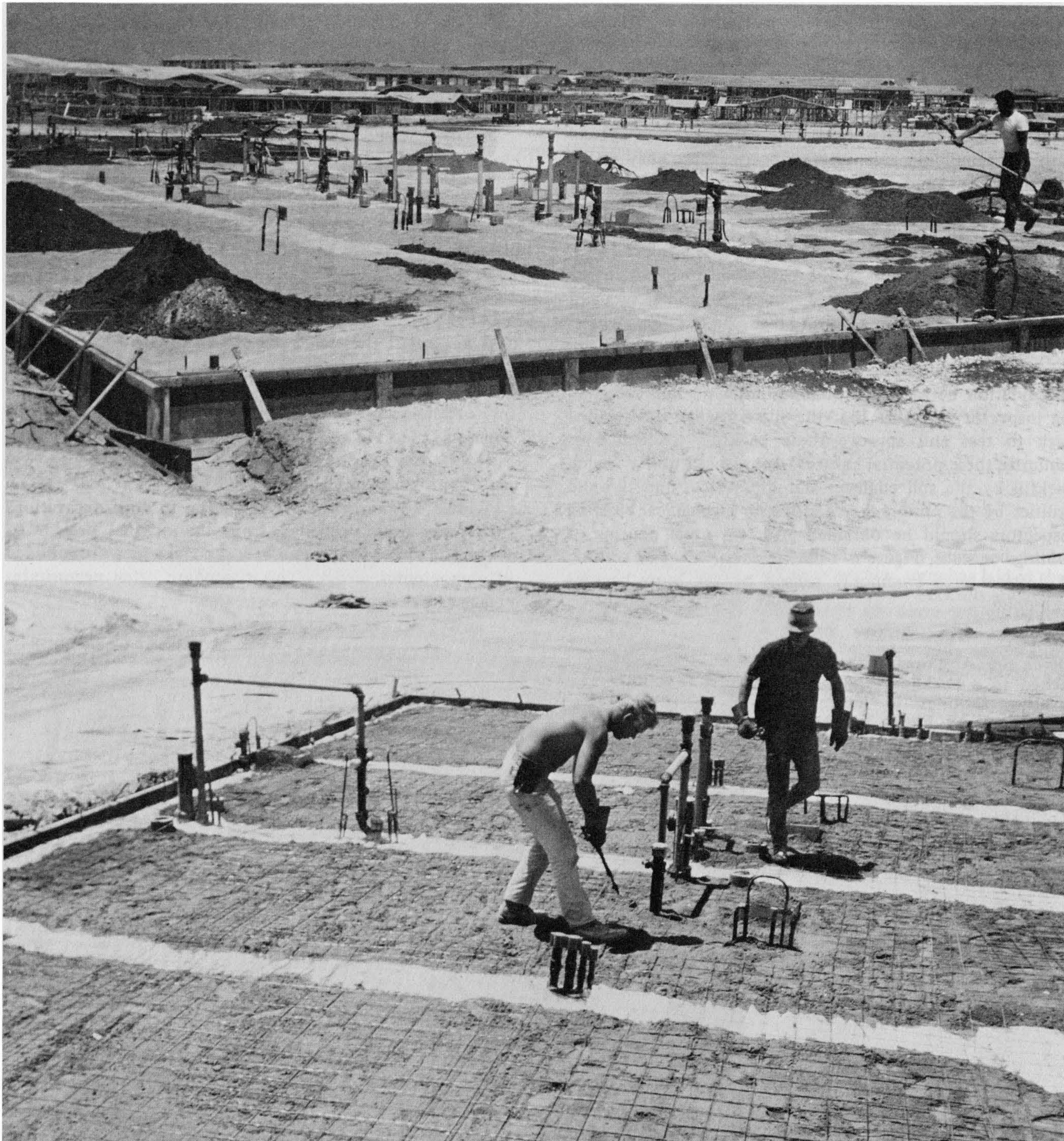
Figure 6-6 (a) An underslab area prior to paving. Underground utilities are shown in place and stubbed off for future connection. Plastic sheets cover the soil, and sand is stockpiled for spreading. (b) The underslab area is ready for the concrete pour. First, sand is spread over the plastic sheets; then wire mesh reinforcement is put in place. The wire mesh must yet be raised and seated on blocks or rock to assure that it is not pushed down to the bottom when the concrete is poured. Photograph by C. Michael Scullin.
