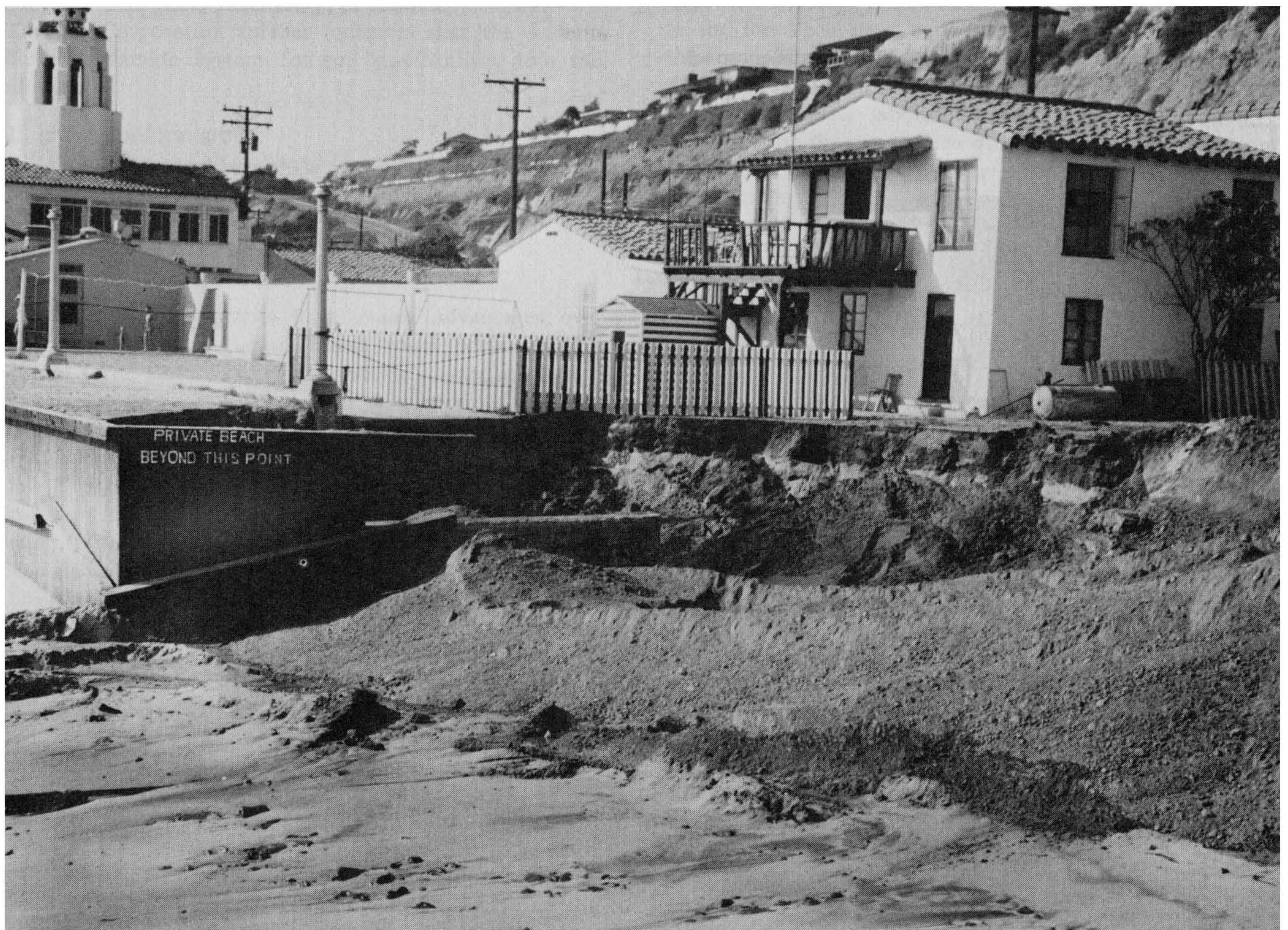
Figure 6-37 This seawall return does not extend back into the lot far enough. A high-sea, high-surf combination has surged the sand out from behind the wall. If the condition is not corrected immediately, this will become a standing wall that can be knocked down by subsequent waves. Photograph by and courtesy of Robert W. Ross.
