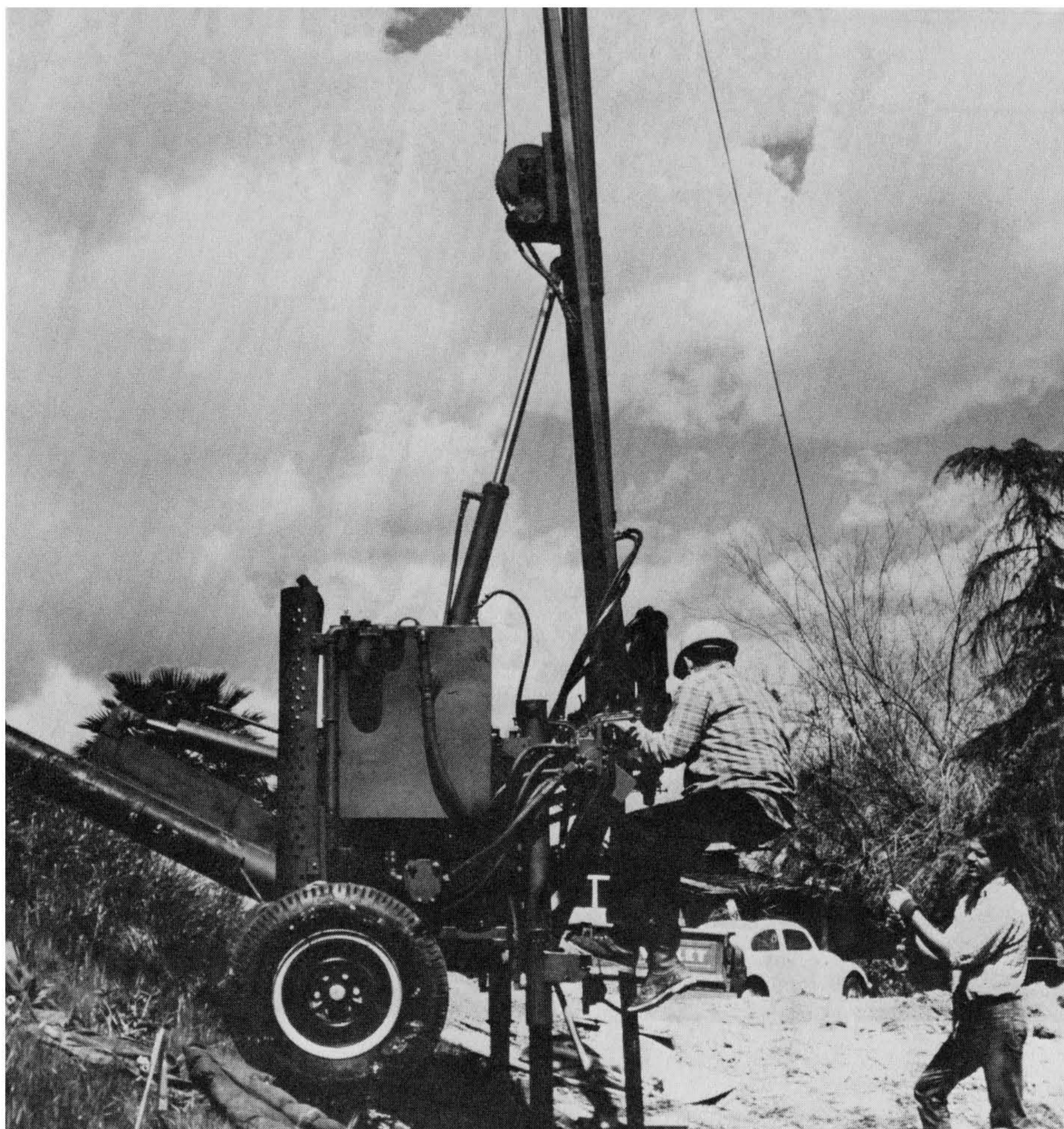
Figure 6-22 (a) A boom-mounted hillside auger rig with 20-ft. hydraulic ram. The driller must change drill stems at each 15 ft. increase in depth. (b) A close-up view of the boom-mounted hillside auger with the operator at the controls. Two stabilization jacks provide support, and the Kelly bar is in the hole. Photographs by and courtesy of Frank E. Denison, geologist.
