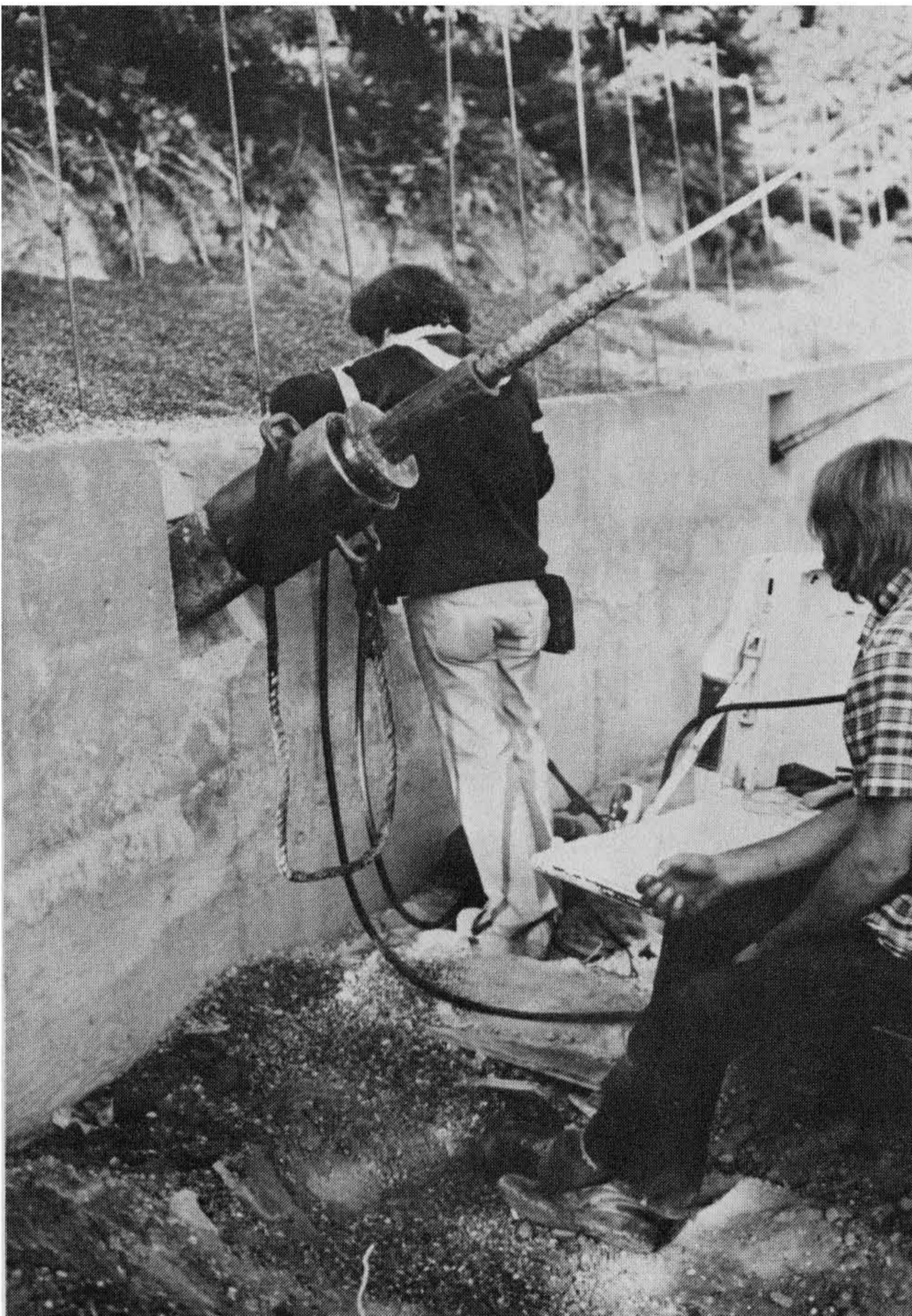
Figure 6-27 Testing tie-backs and measuring movement between plate and jack. The tie-back is mounted on a vertical soldier pile and a horizontal grade beam. Note the gravel and steel above for a proposed 4-ft. high retaining wall. Photograph by and courtesy of Frank E. Denison, geologist.
