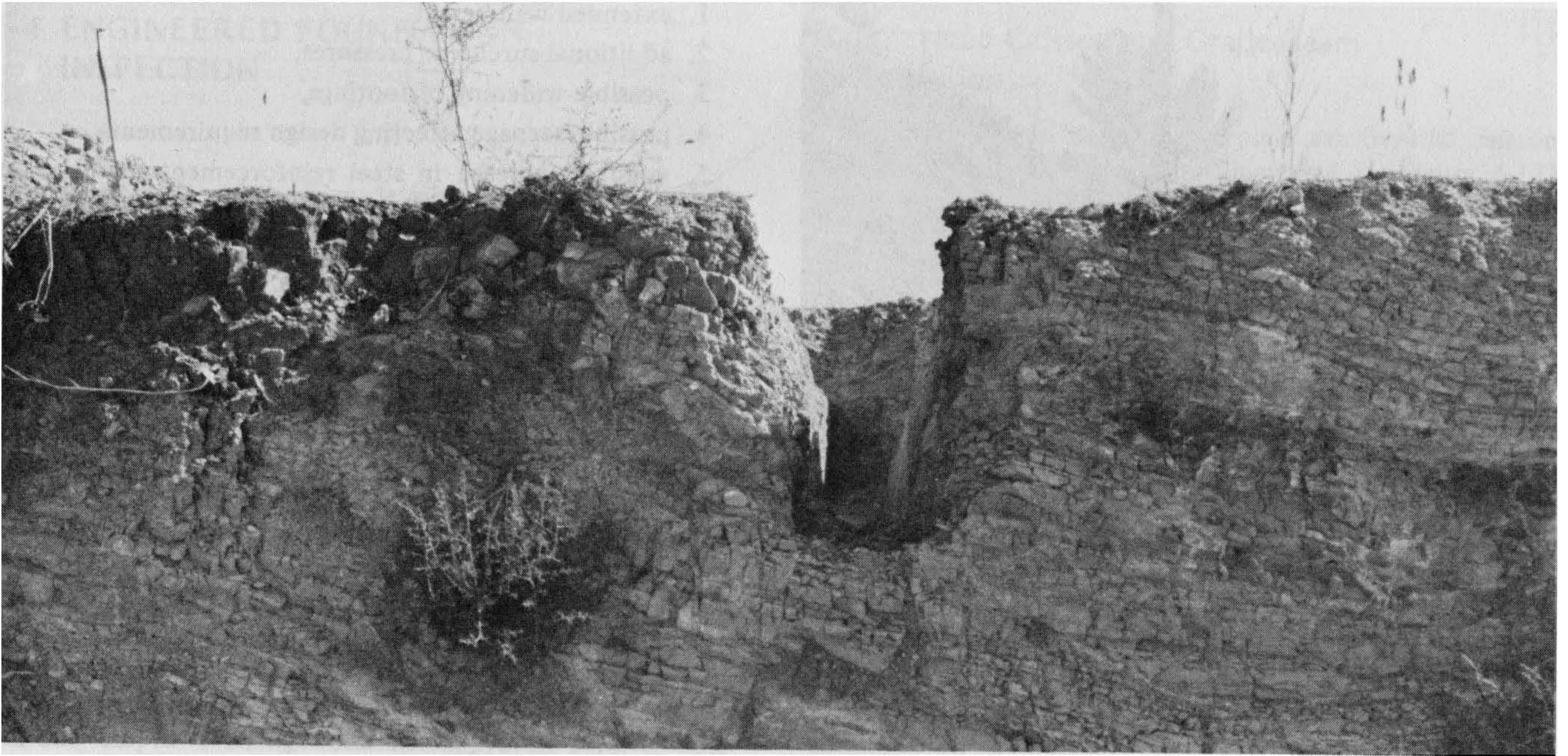
Figure 6-7 Footing excavation has been deepened through the near surface bedrock creep and is founded on competent bedrock. Photograph by C. Michael Scullin.
