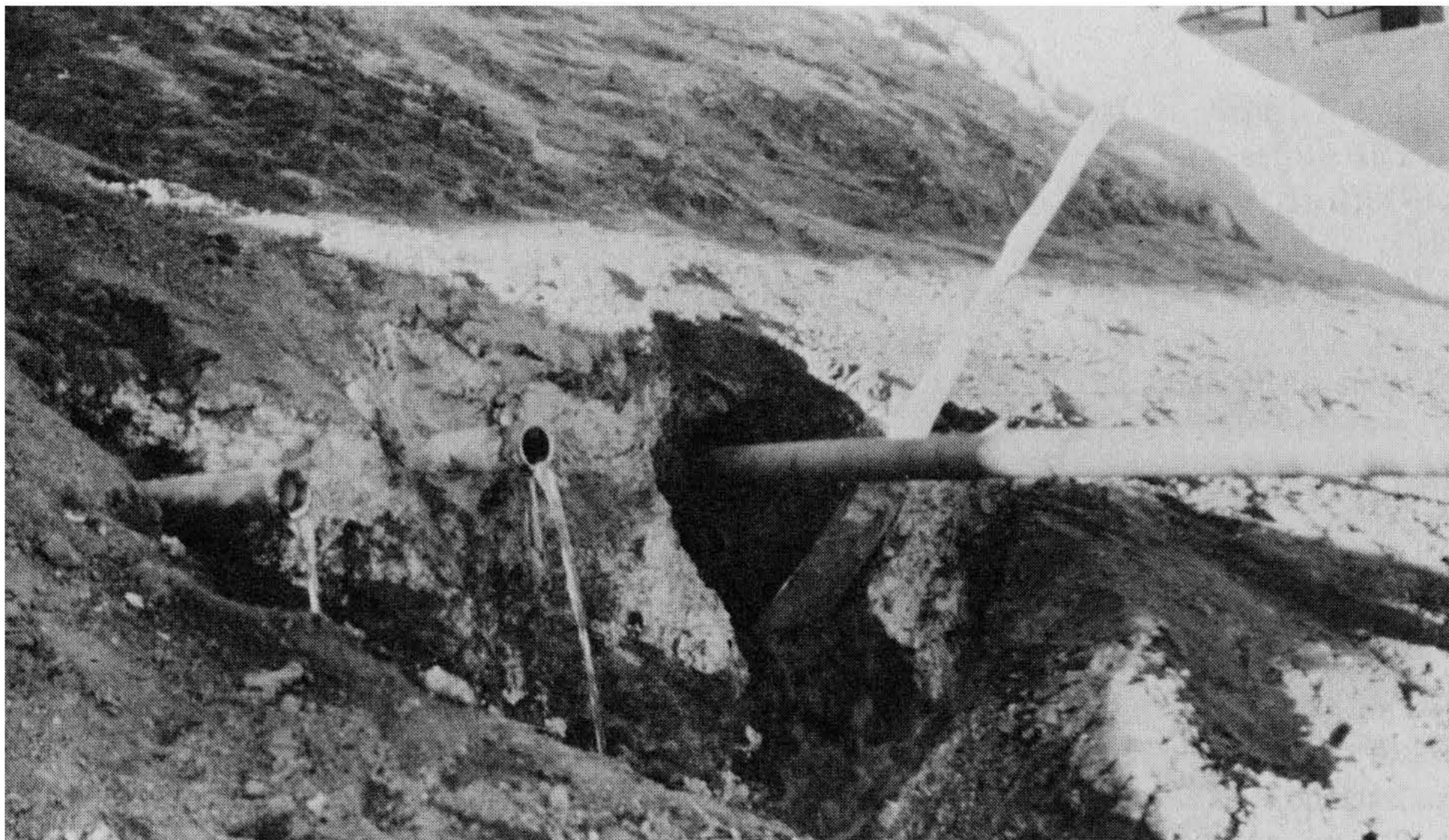
Figure 6-24 These horizontal sub-drains are functioning as intended. The drain on the right is being drilled. Photograph by and courtesy of James E. Slosson.
