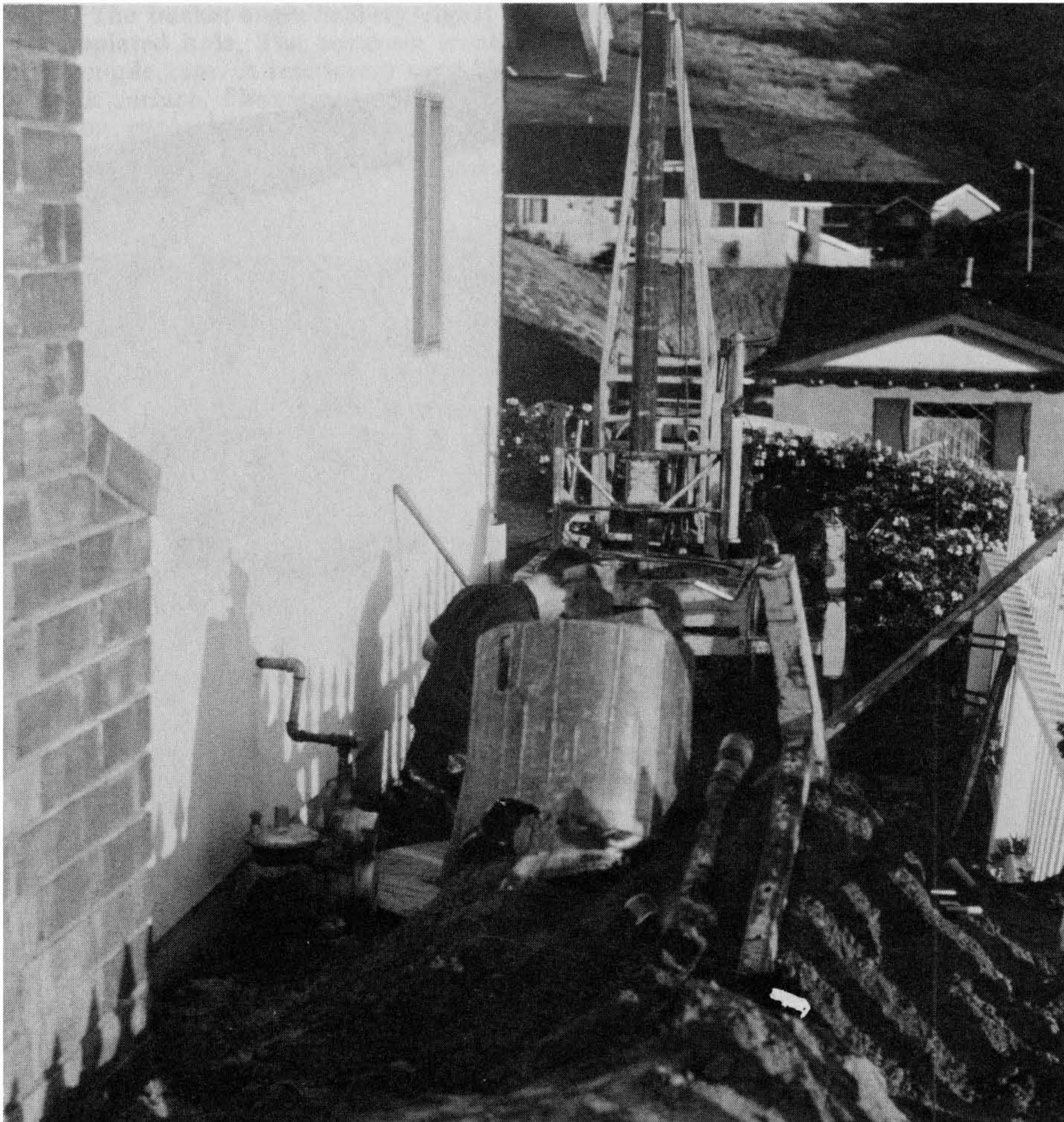
Figure 6-11 Drilling to underpin the rear foundations of an existing residence using a detached hillside bucket-auger drill rig. Photograph by and courtesy of Robert W. Ross.
