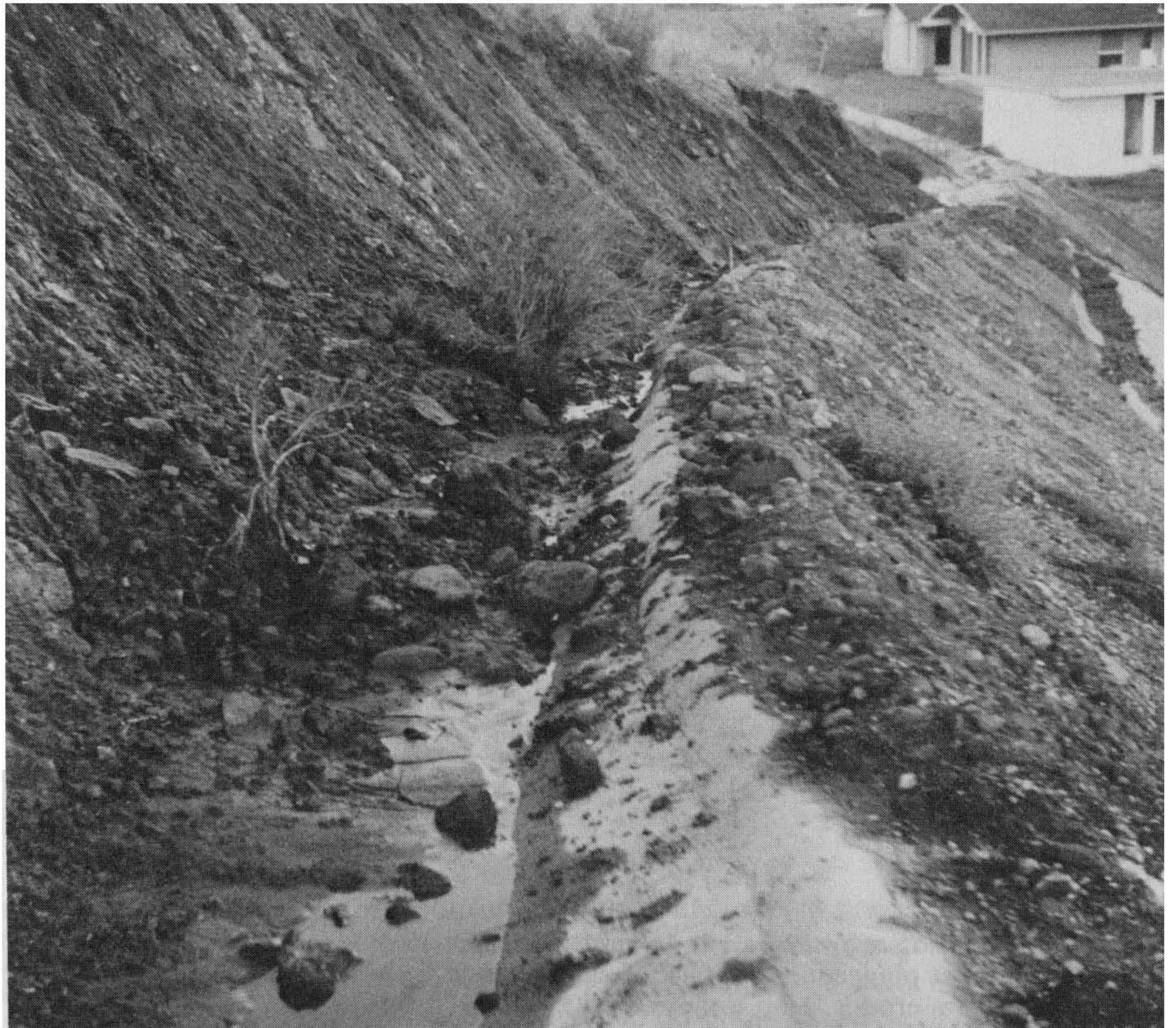
Figure 9-9 Colluvial soils and stream terrace gravel materials slumping and rilling into slope drains. These terrace slope drains have minimum gradients of 2%-4% which are insufficient for self-cleansing or removal of heavy slump materials. Photograph by C. Michael Scullin.
