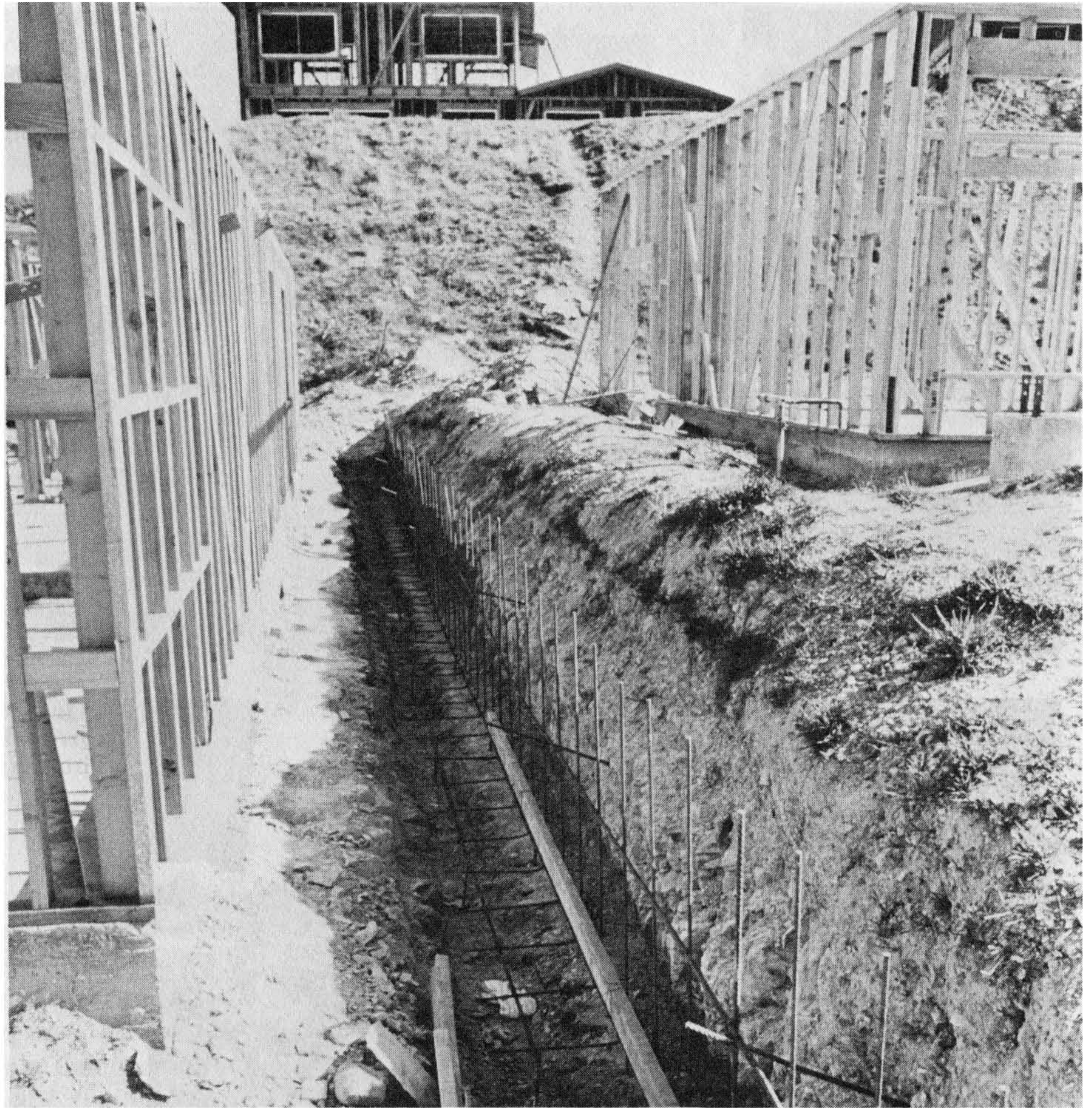
Figure 9-18 Retaining wall construction along a mutual property line. Notice the close proximity of the residence foundations to the property line and the narrow sideyard. Photograph by and courtesy of Alex Bruce, senior building inspector, City of Los Angeles.
