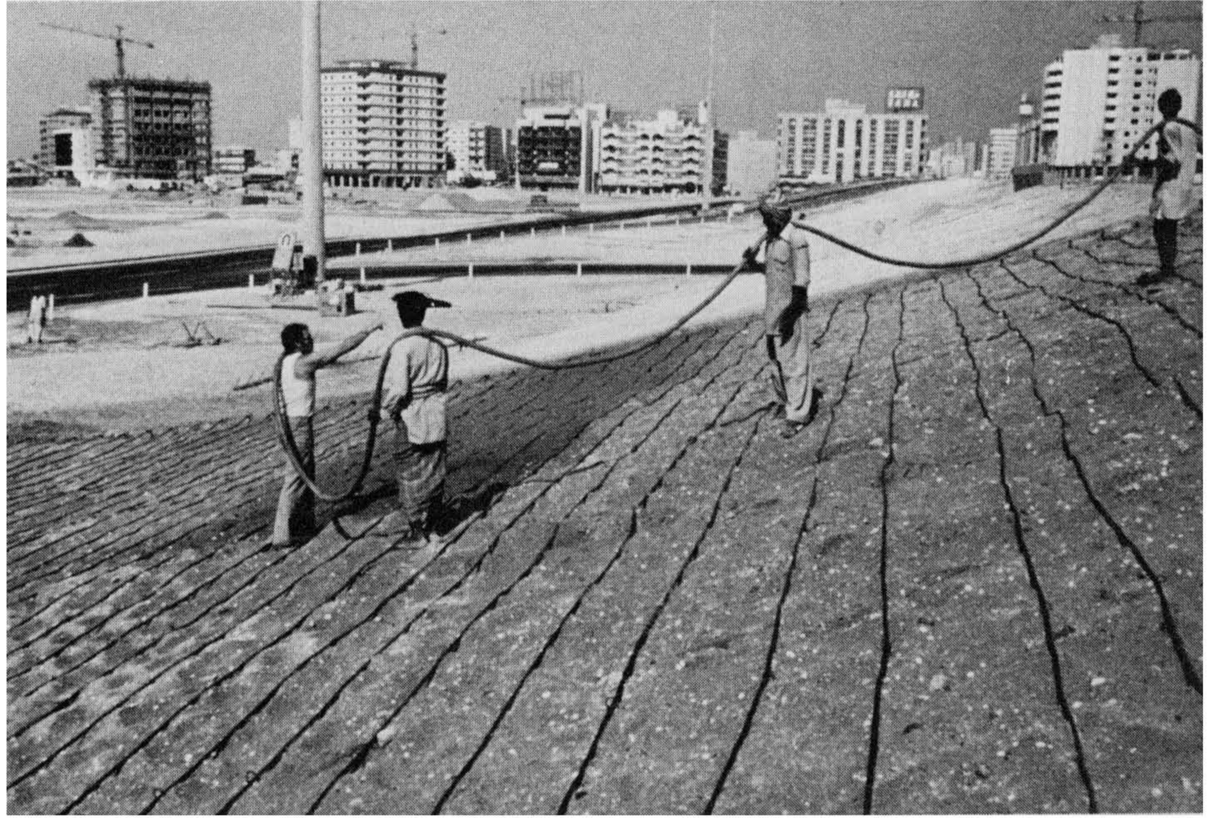
Figure 9-33 Hydroseeding installation at the El Khan Bridge Freeway Project, State of Sharjah, United Arab Emirates, November, 1978. This seedmixture was drilled into dredged sand via hydroseeding. Photograph by and courtesy of Ronald Pecoff.
