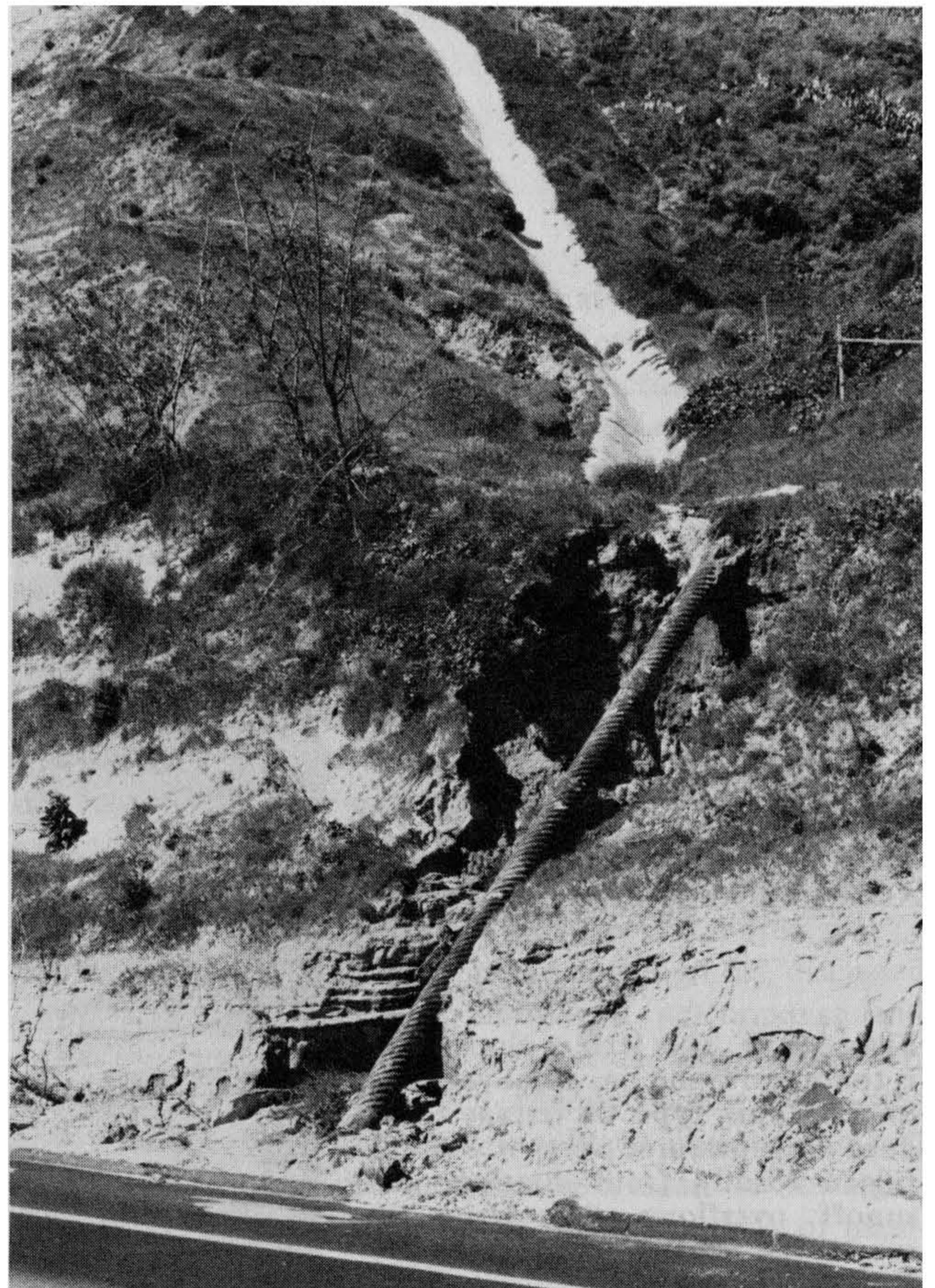
Figure 9-13 A pipe down-drain that has plugged up. The water has overtopped the slope and a gully has formed by erosion. An open channel down-drain would have performed better. Photograph by C. Michael Scullin.
