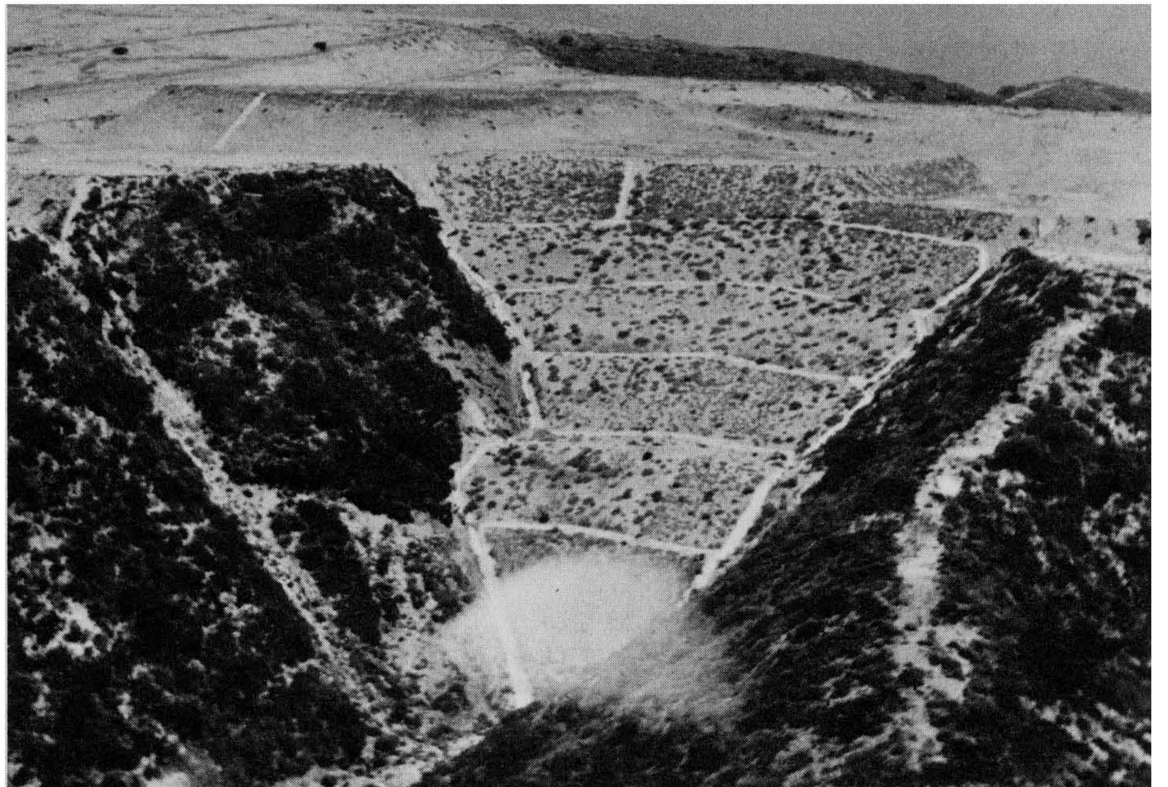
Figure 9-15 An engineered compacted fill in a V-shaped canyon with down-drains constructed along both daylight lines for good erosion control. Photograph by and courtesy of Robert W. Ross.
