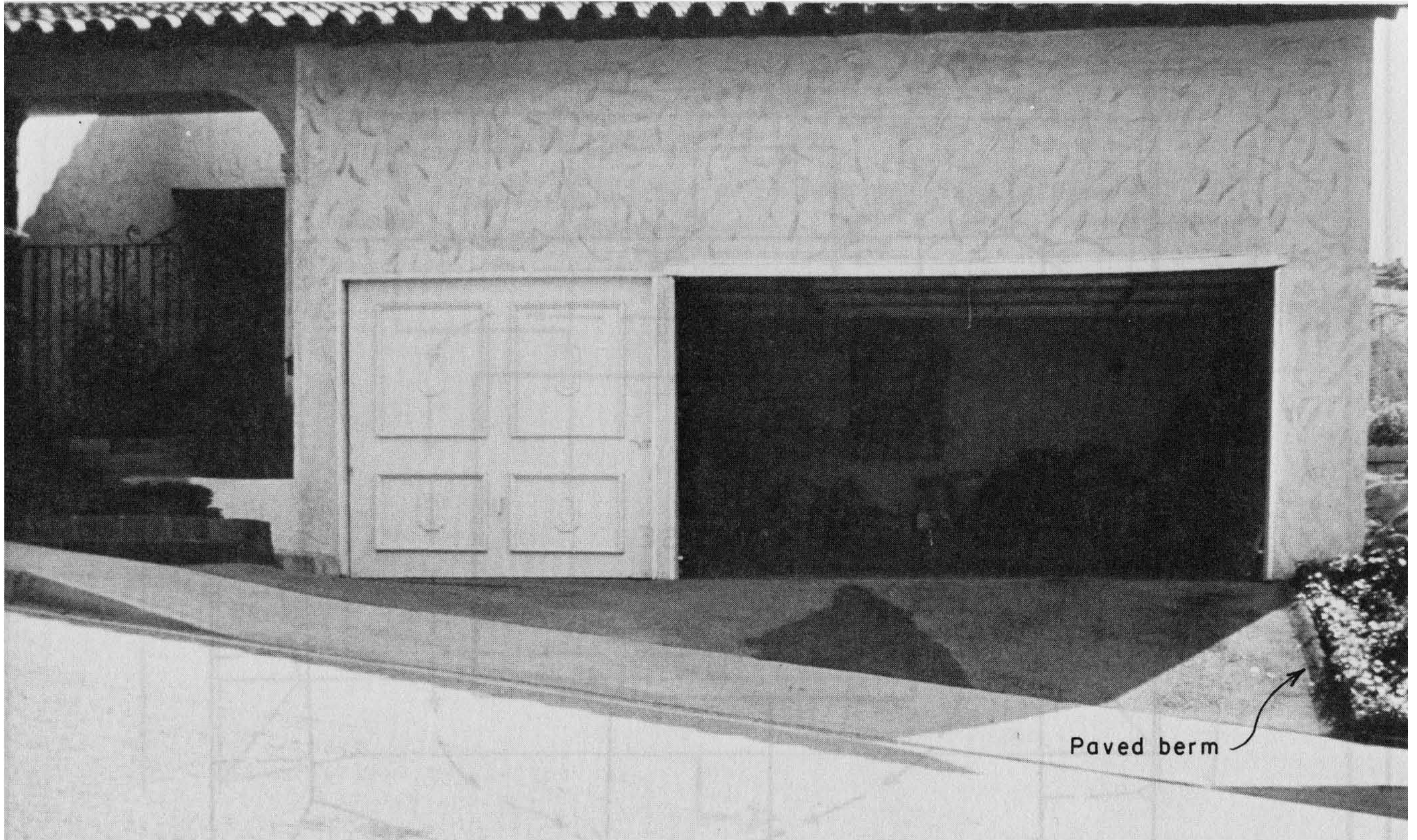
Figure 9-8 Lot drainage onto a steep street. Notice the asphalt berm on the right side of the driveway to assure that drainage stays in paved area. Photograph by and courtesy of Alex Bruce, senior building inspector, City of Los Angeles.
