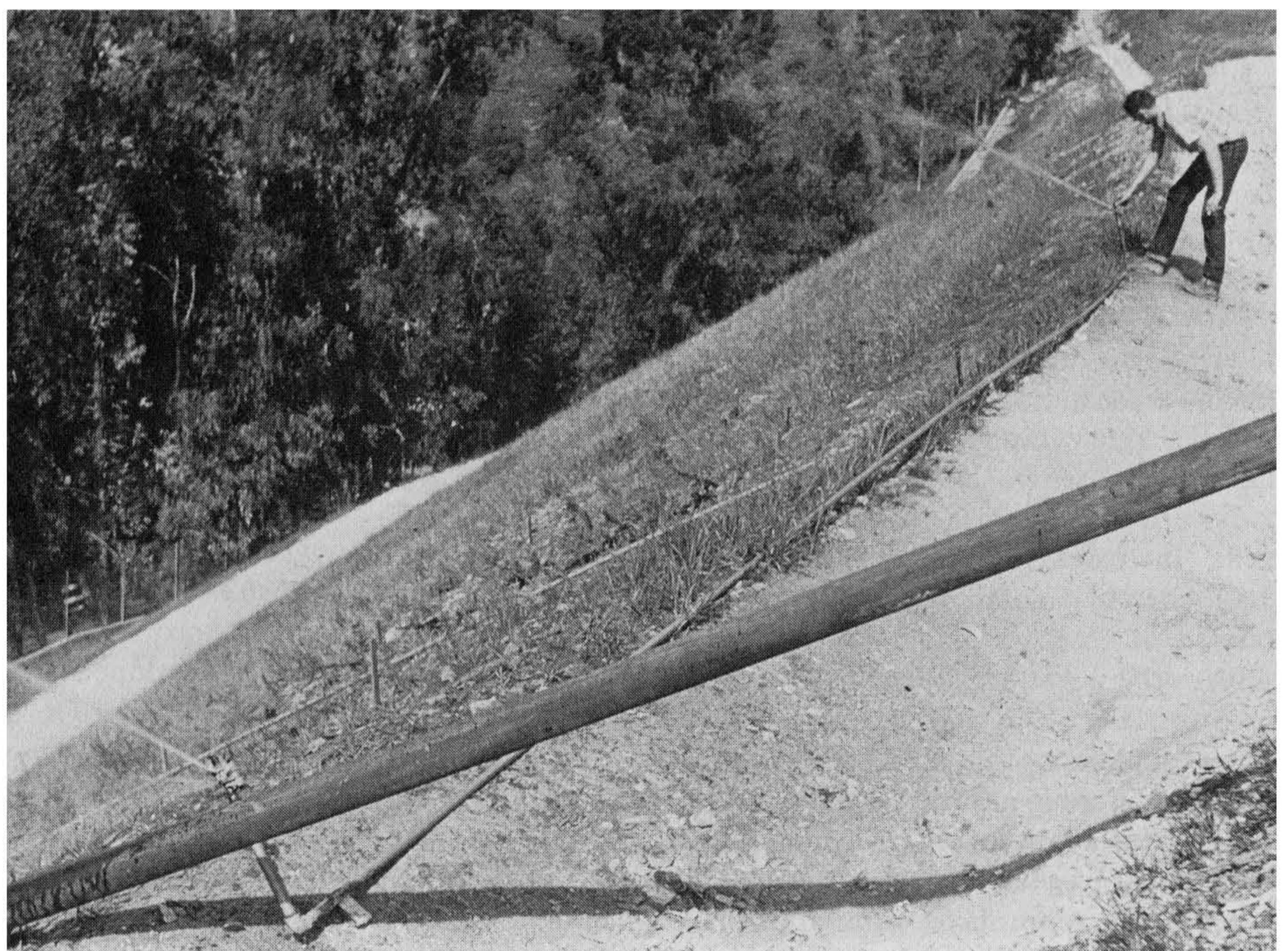
Figure 9-24 Checking sprinkler heads and "rainbird" performance. Close maintenance of watering devices is necessary to minimize oversaturation. Photograph by and courtesy of Alex Bruce, senior building inspector, City of Los Angeles.
