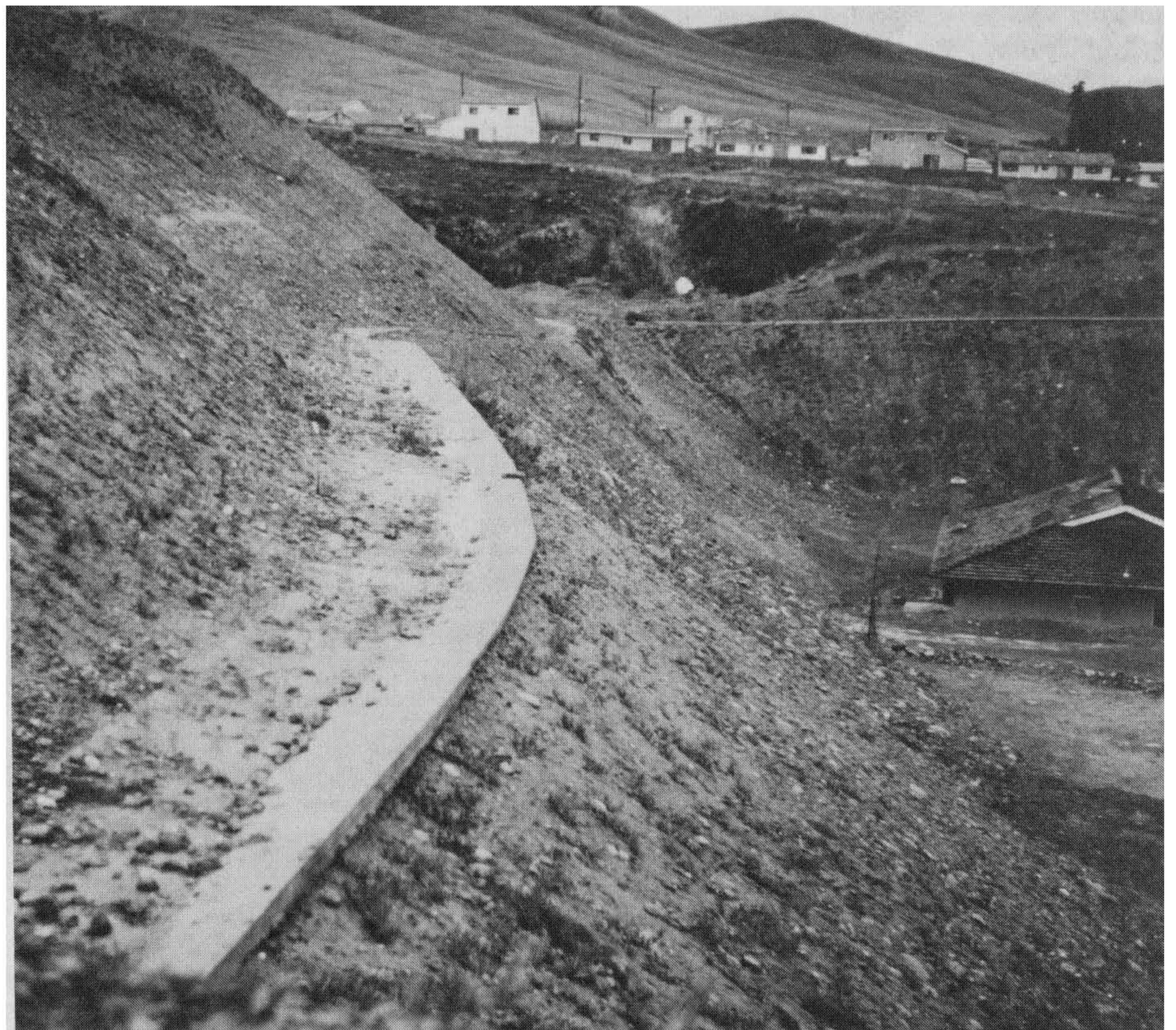
Figure 9-10 This terrace slope drain is too narrow and has a flat gradient of 2%. This type of terrace drain does not perform very well as it fills-in readily from siltation, and runoff overflows the drains to erode the slopes. Photograph by C. Michael Scullin.
