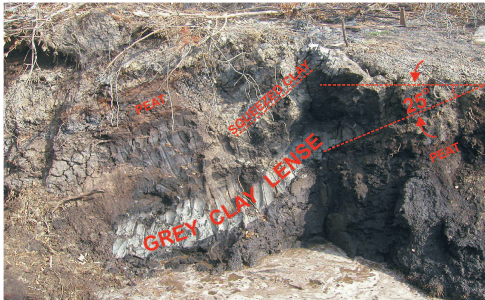
Fig. 13. (Color) Annotated photo of trench excavated into south end of displaced 17th St. canal levee (photo taken from IPET 2006). Thicker seam or gray lacustrine clay approximates position of thrust between base of levee embankment and Thrust sheet 3, noted as small box labeled Fig. 13 on Section No. 6 of Fig. 12. This lense dips about 25° west, back towards canal.
