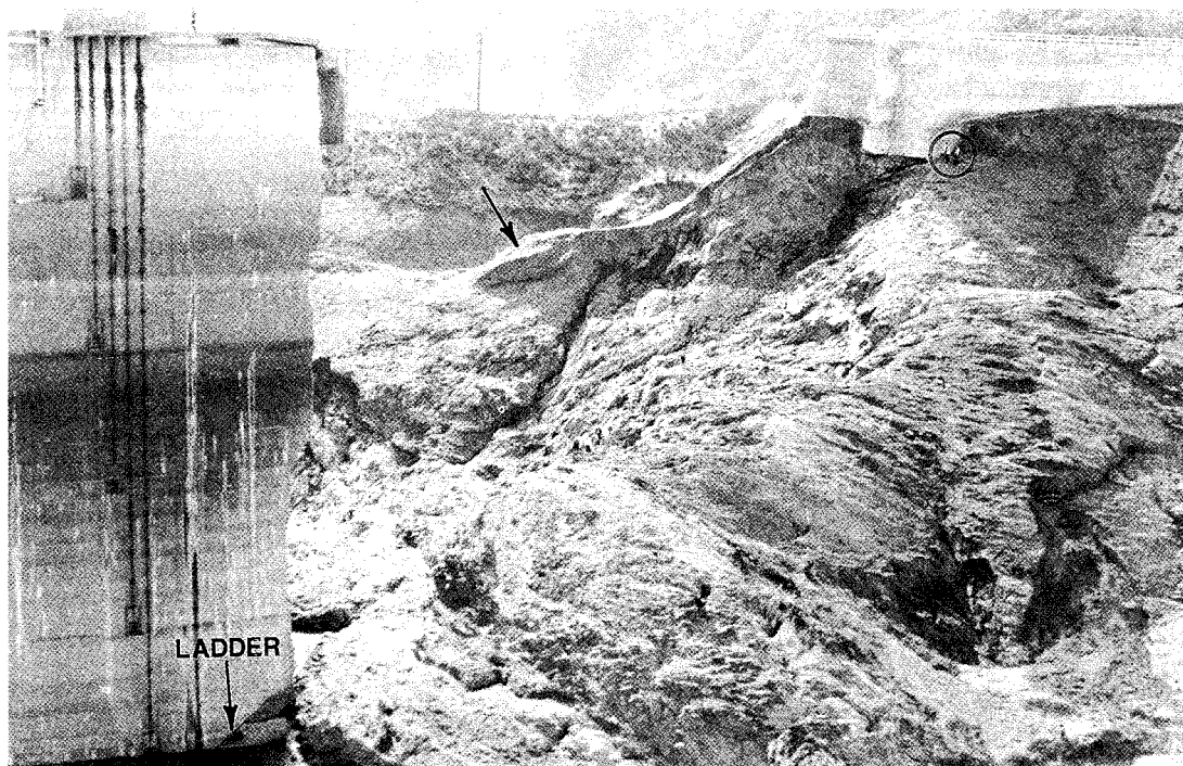
Figure 24. (lower) Detail of failed west abutment, looking downstream, with people circled for scale. Only a portion of the west dike access road side-cast fill was excavated by the outpouring water (arrow), with scrub brush left upon the cut slope, down to elevation 1785, 50 feet below the reservoir level. Grunsky's ladder, caught in the upstream heel crack as Block 1 tilted downstream, is annotated (photo courtesy of Ventura County Museum of History and Art).
