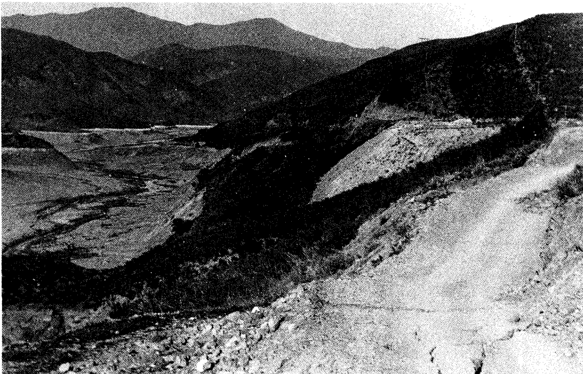
Figure 14. (lower) Post-failure view looking up-canyon from the higher, surge chamber road, above the east abutment slide headscarp (position "A" in lower portion Figure 13), a few days after the failure. Retrogressive tension scarps reached 200 feet uphill of the slide, encroaching on the high road as shown, dropping it by about 10 feet. The Edison Power line that went down at 11:57 PM is shown as "A" and the slide depicted in Figure 1 is delineated as "B".
