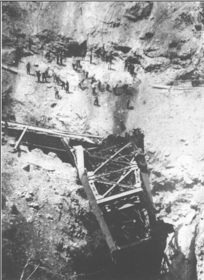
"By hand, meaning with compressed-air hammers, picks and shovels, the non-supporting rock is removed so the concrete foundation for the Roth-Wagner bridge pillars can be laid."
