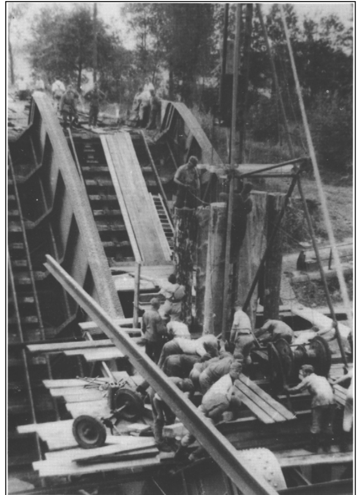
A railway bridge blown up by the Russians in 1941, being restored by railway engineers using a Diesel pile-driver.
